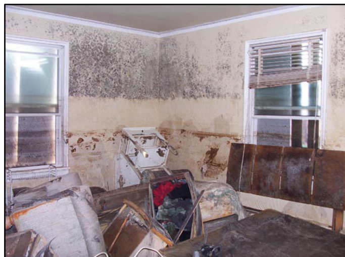
Fig 1. Typical flood damage to furniture and interior walls.
