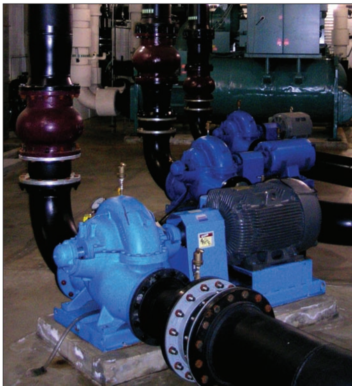
Furman University HVAC
