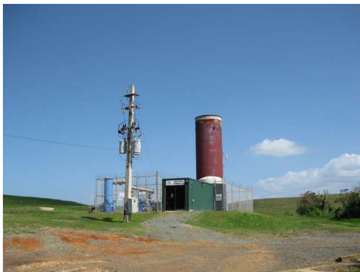
Figure 20. San Juan Landfill gas flaring facility
