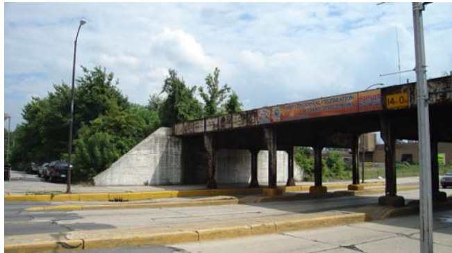
Figure 15. Photo of the CSS & SB rail corridor over Broadway circa 2007. The overpass for the rail line is rusting. Beyond the overpass, the railroad track is covered in overgrowth as a result of deferred maintenance. 28
