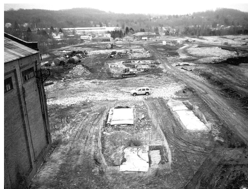
Fairmont Coke Works — 4/5/99 — The demolition is near completion, with many of the structures completely leveled.
