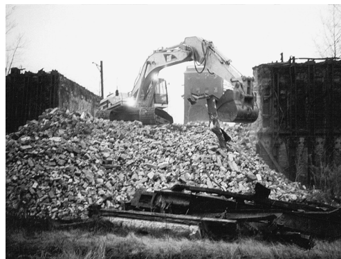
Fairmont Coke Works — 1/14/99 — Beginning the demolition. Trackhoe demolishes some of the onsite structures. This demolition will help to prepare the site for redevelopment.
