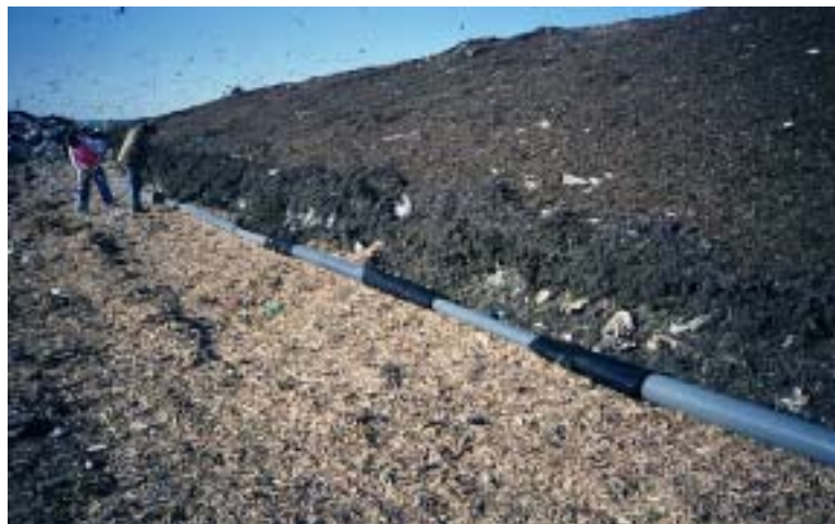
Image 3-2. Horizontal LFG collection line
