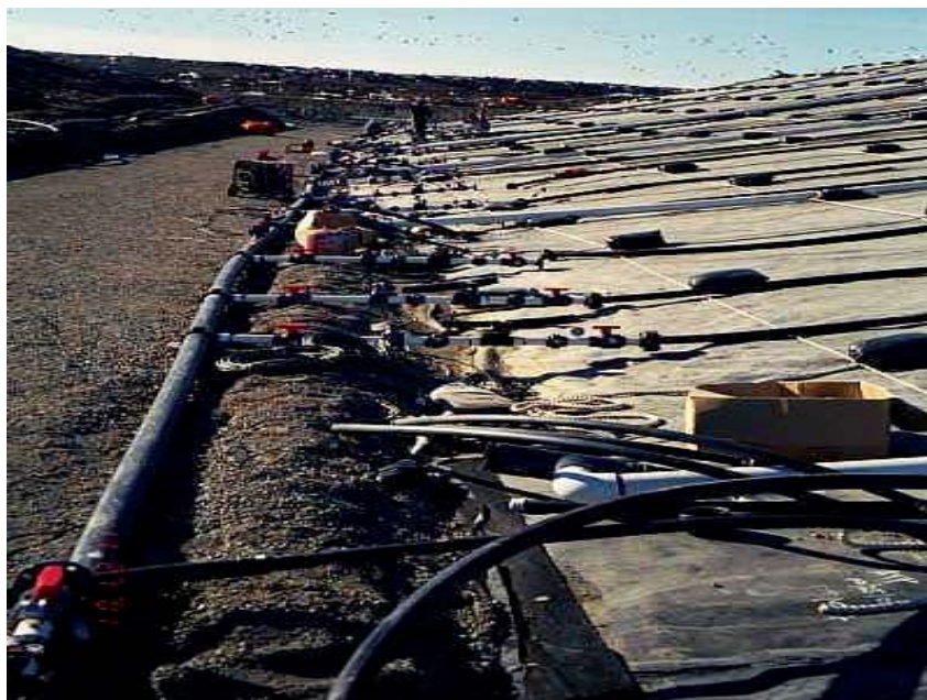
Image 3-7. Leachate injection header and laterals
