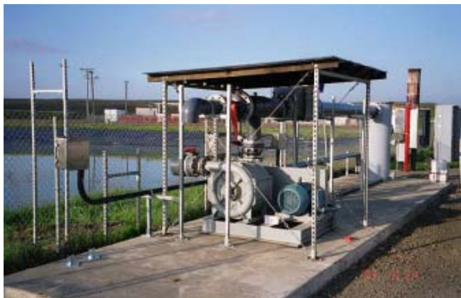
Image 5-7: Aerobic Cell Blower Station
