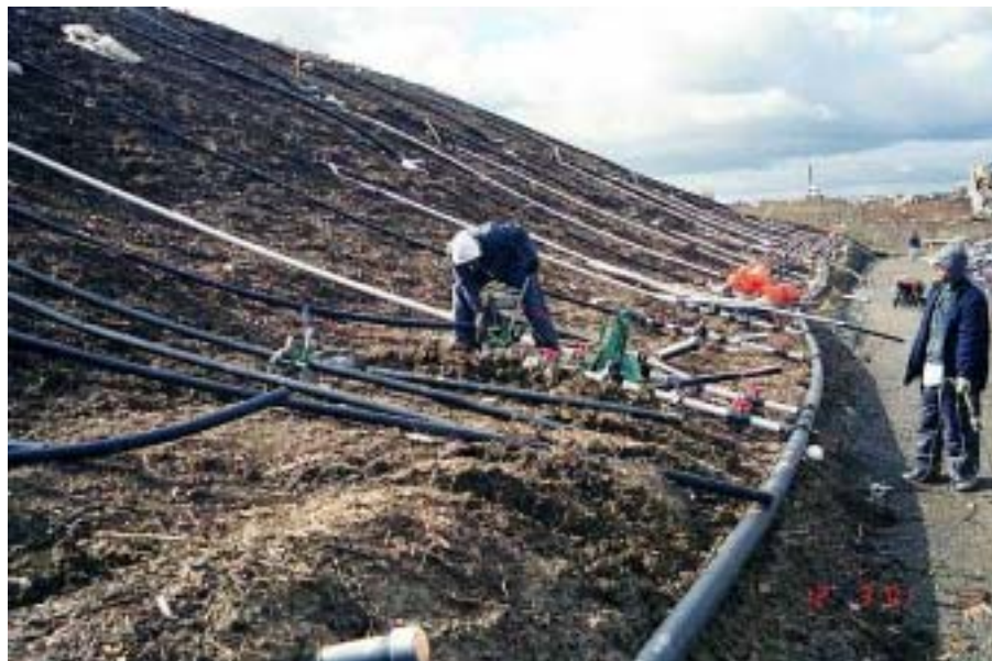
Image 5-5. Aerobic leachate injection header and lateral
