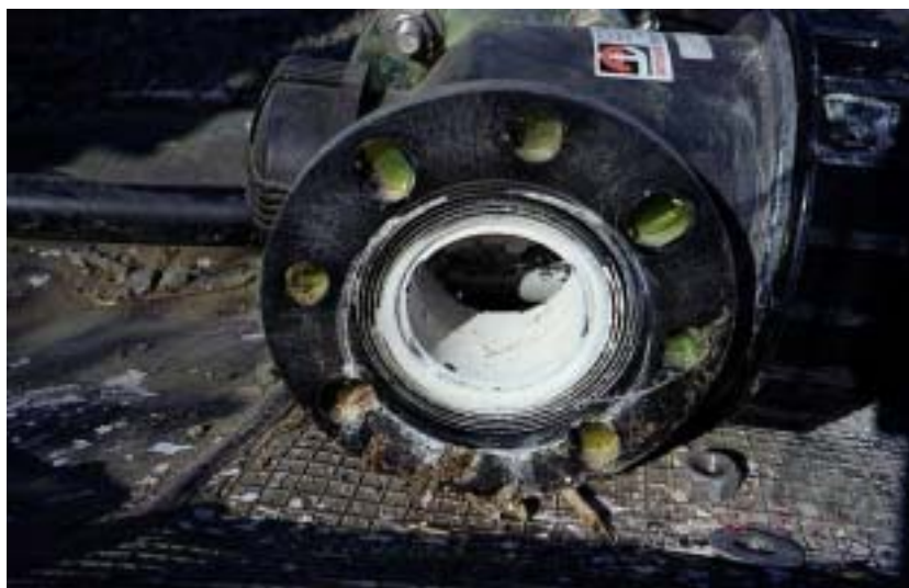
Image 3-8. Scale buildup on the northeast 3.5-acre leachate injection lines.
