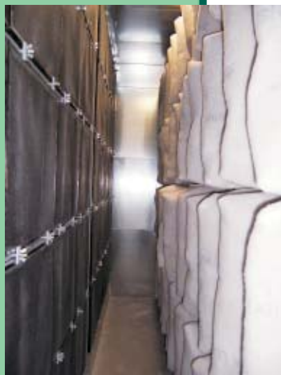
Paint booth carbon adsorption unit
