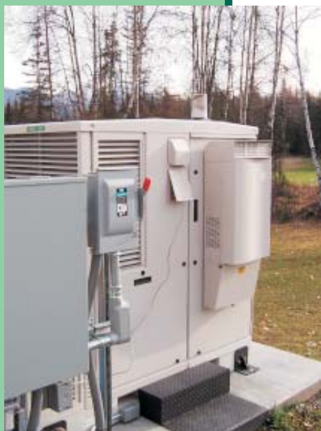
Fuel Cell at Fire Station 3
