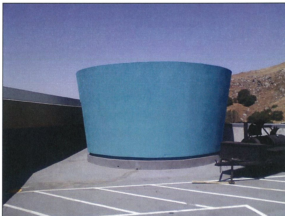
PHOTO 6: Kitchen and casino parking garage exhaust systems on the north of the top floor.
