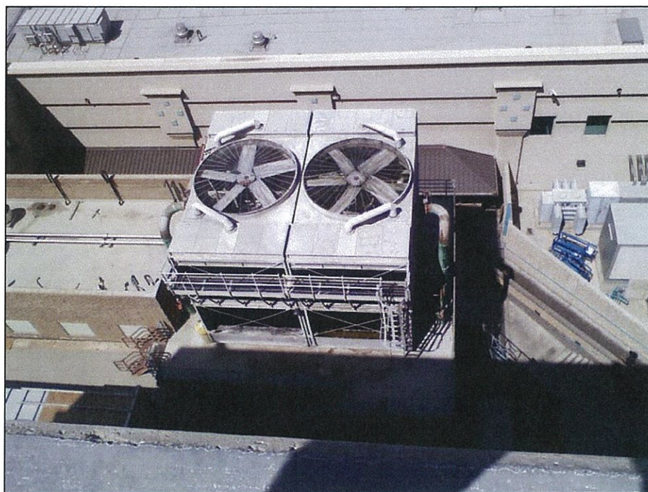
PHOTO 8: Air conditioning unit on the southwest side of the parking garage.
