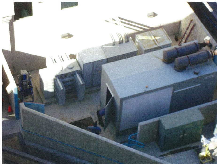
Figure 27: View of backup generators, November 20, 2008.
