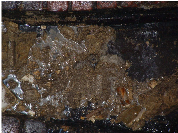
Sewer Line Impacted from Excess Grease Build-up
