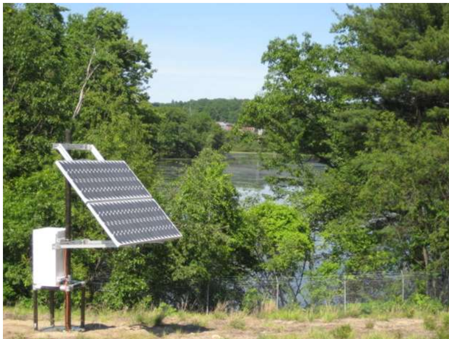
Figure 19 Solar power system was installed uphill south of Red Cove.
