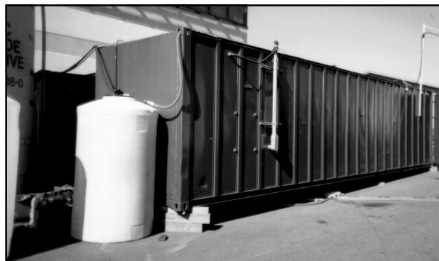
Exterior Photograph of Centrate Settling Tank and Processing Trailer
