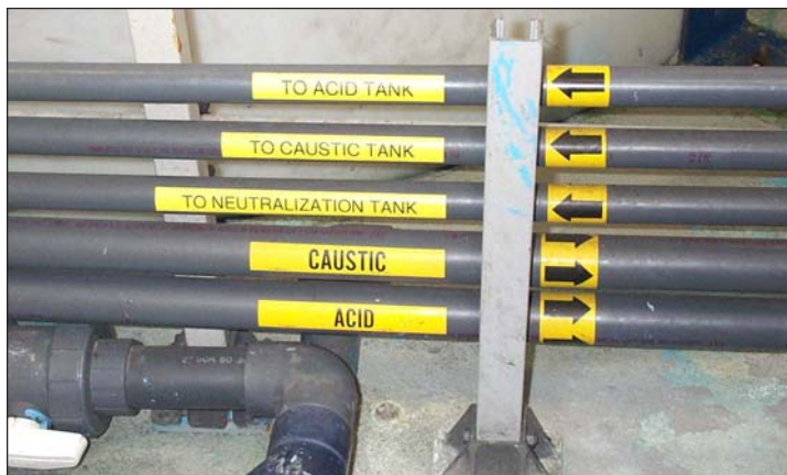
Photo 4. Acid, base and neutralization streams to and from the columns.
