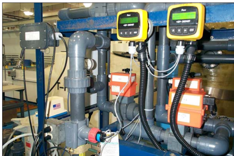
Photo 5. Signet flow totalizers and flow sensor (bottom).
