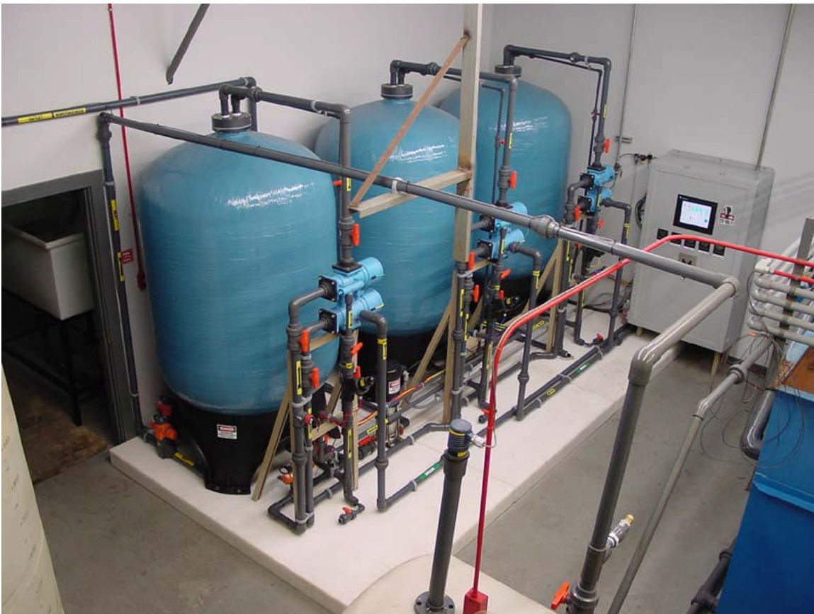
Figure 9. Photograph of the Ion Exchange Polishing System Installed at Gull Industries
