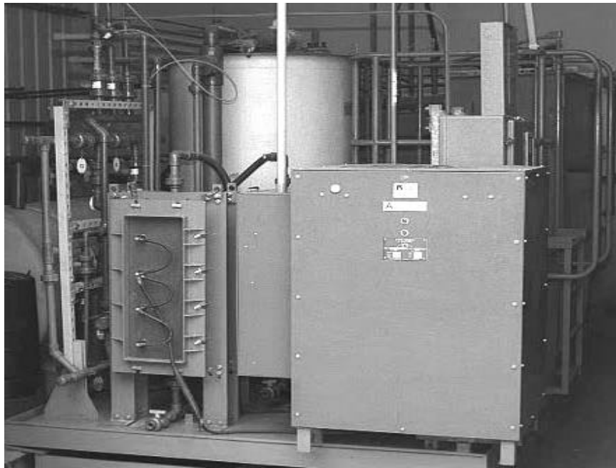
Figure 8. Photograph of the Kaselco System Installed at Gull Industries
