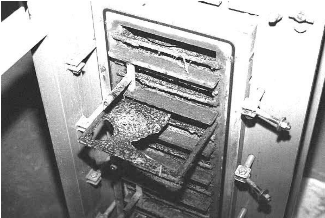
Figure 3. Photograph of Interior of Electrocoagulation Reactor (Rx)
