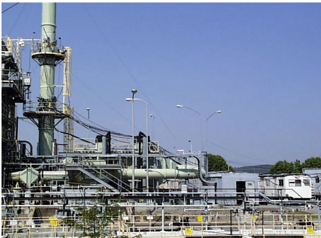
Figure 3-3. Side View of TSCAI Stack. Sampling platforms are at the left and CEM trailers are at the lower right.
