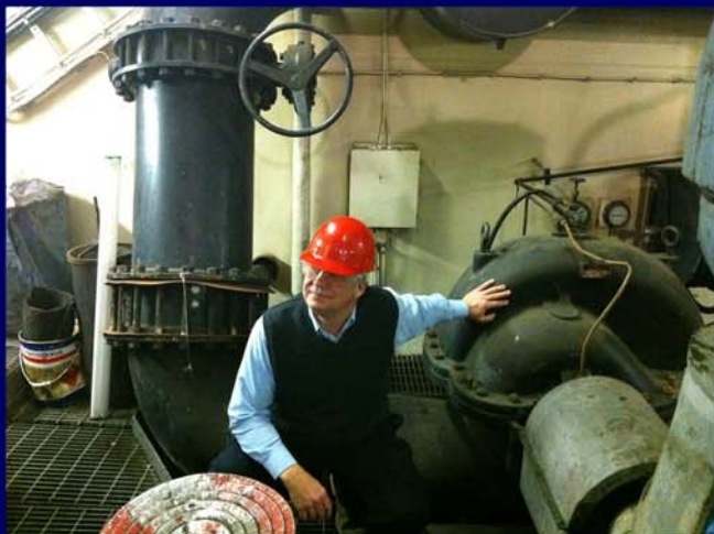
Richard Stewart, GLMRI, kneels in front of ballast water piping and pumps in the Edwin H. Gott .
