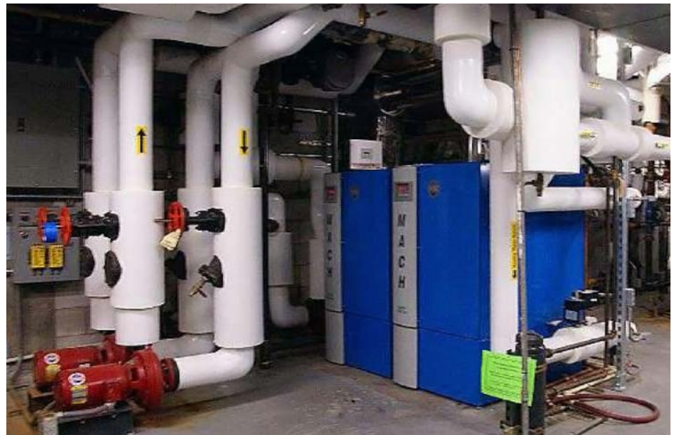
Engineered sites received boiler assessments and upgrades as part of the BLM ESPC. Photo from Bureau of Land Management
