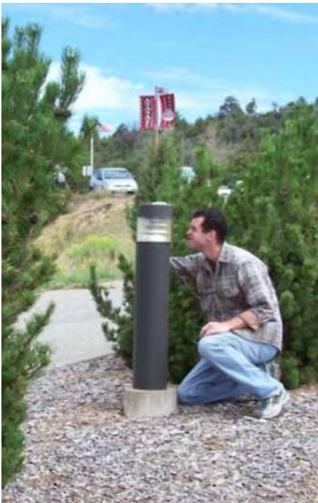
BLM replaced exterior lighting with energy-efficient models. Photo from Bureau of Land Management
