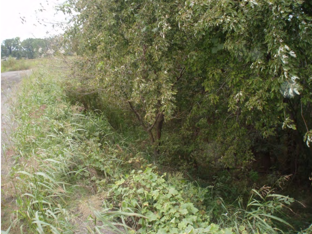
13. EXTERIOR OF NORTHWESTERN PORTION OF PERIMETER DIKE (AREA 4) – HEAVY VEGETATION AND TREES OBSERVED.
