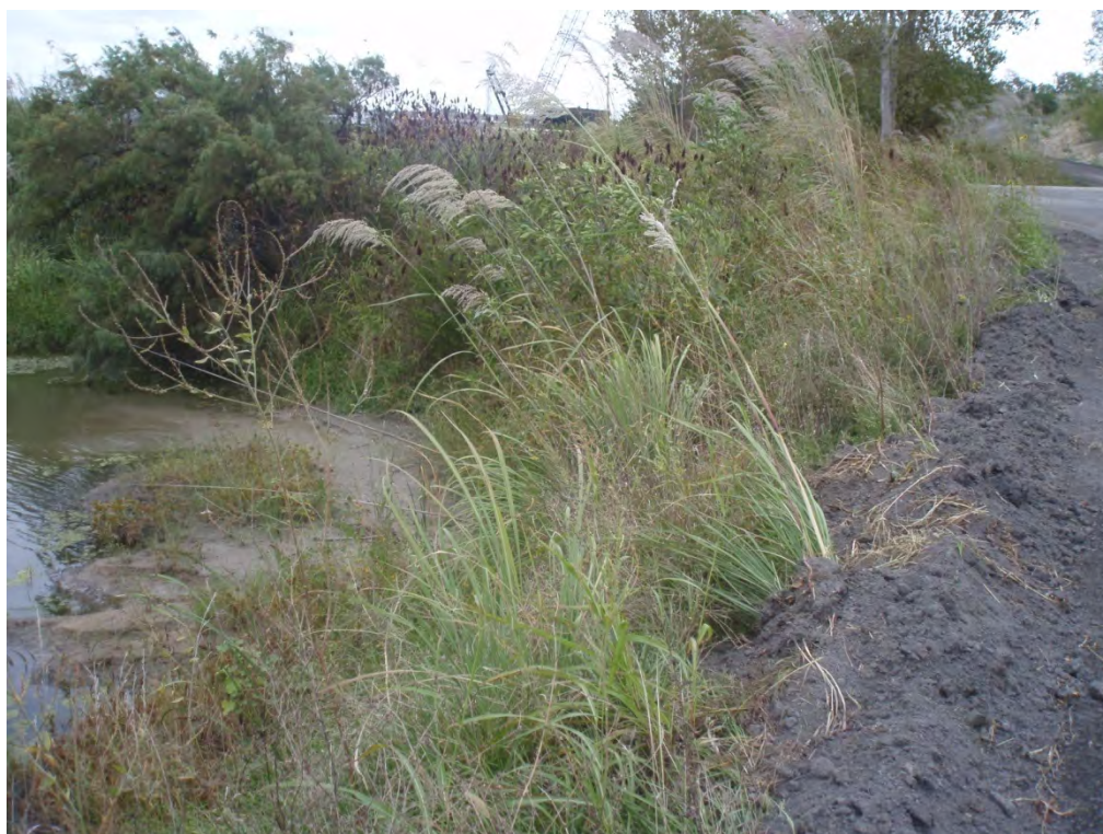
28. INTERIOR VIEW OF PERIMETER DIKE TO EXISTING GRADE/ROAD EMBANKMENT ALONG SOUTH SIDE OF AREA 3.
