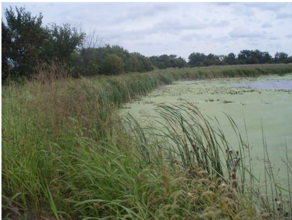
19. INTERIOR OF NORTHWESTERN PORTION OF PERIMETER DIKE – TAKEN FROM MIDPOINT (BETWEEN AREA 3 AND 4) LOOKING NORTH
