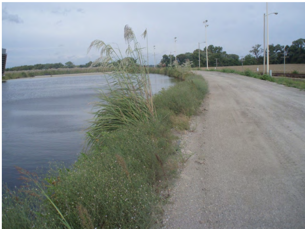
3. INTERIOR OF NORTHEASTERN PORTION OF PERMETER DIKE – TAKEN FROM EAST END OF AREA 1, LOOKING WEST
