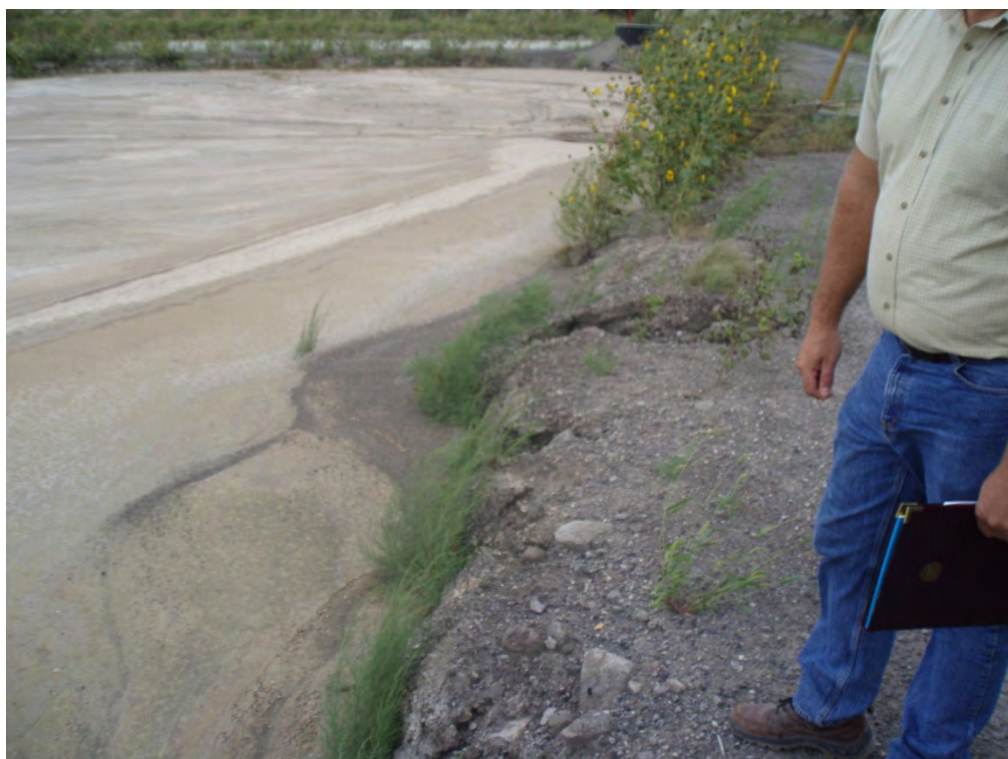
10. INTERIOROFNORTHEASTERNPORTIONOFPERMETERDIKE IN AREA 4 – SOME MINORWASHOUT/EROSIONOBSERVED.
