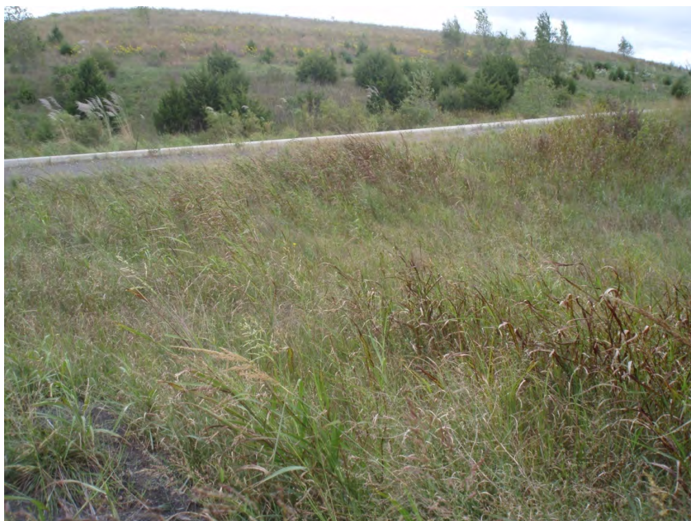
27. EXTERIOR VIEW OF PERIMETER DIKE TO EXISTING GRADE/ROAD EMBANKMENT ALONG SOUTH SIDE OF AREA 3.
