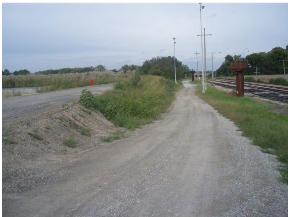
4. EXTERIOR OF NORTHEASTERN PORTION OF PERMETER DIKE – TAKEN FROM EAST END OF AREA 1, LOOKING WEST
