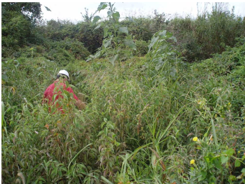
6. OUTFALL OF EMERGENCY OVERFLOW STRUCTURE – EXTERIOR OF NORTH SIDE OF AREA 1 DIKE. HEAVY VEGETATION MAKES ACCESS TO THE OUTFALL IMPRACTICAL.
