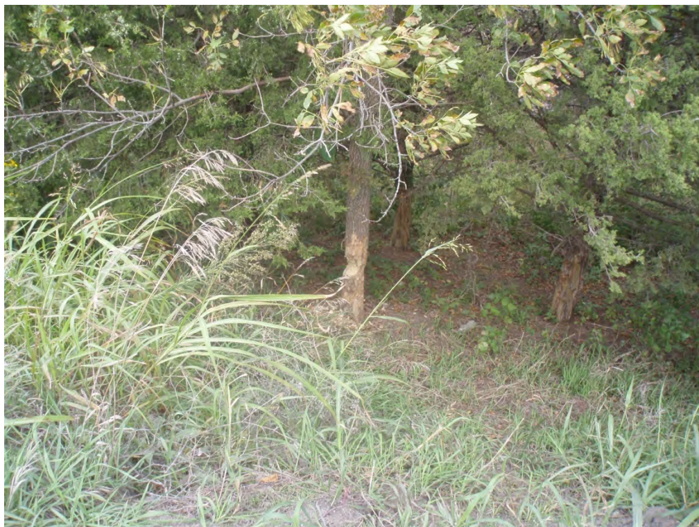
18. EXTERIOR OF NORTHWESTERN PORTION OF PERIMETER DIKE (AREA 4) - 10" TREE OBSERVED AT TOE OF EMBANKMENT
