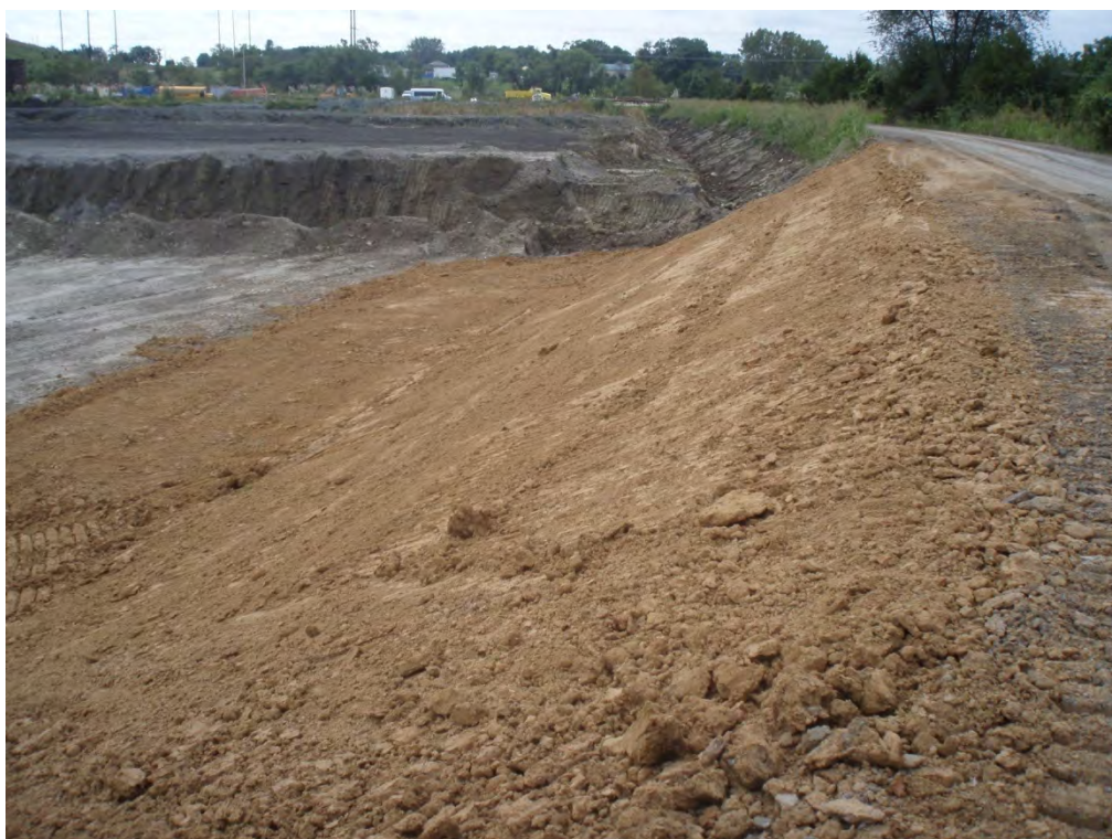
20. INTERIOR OF WESTERN PORTION OF PERIMETER DIKE (AREA 3) – TAKEN FROM WESTERN DIKE LOOKING SOUTH ALONG INTERIOR OF DIKE. CLAY LINER BEING INSTALLED
