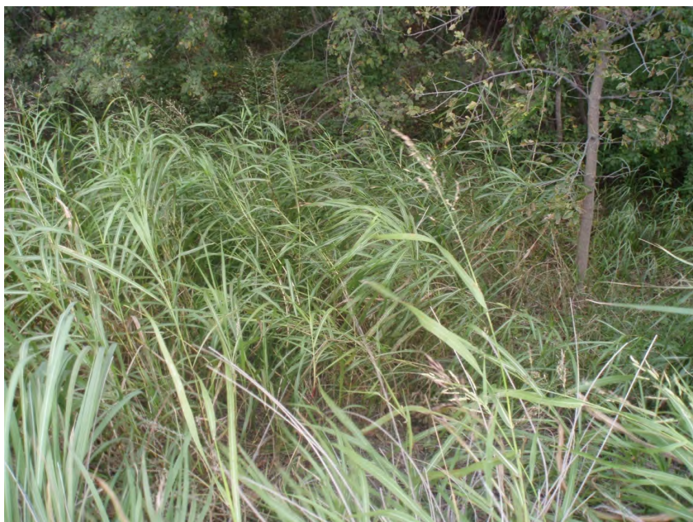
12. EXTERIOROFNORTHEASTERNPORTIONOFPERMETERDIKE (AREA 4) – HEAVYVEGETATIONOBSERVED.
