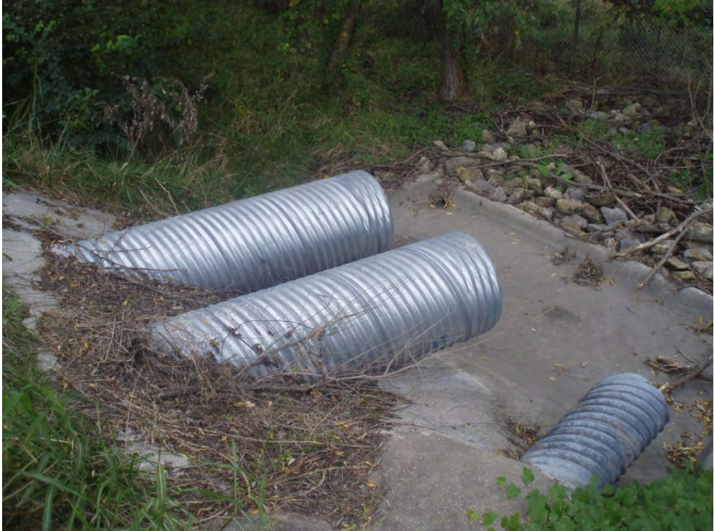
25. STORM WATERPOND OUTFALL PIPES ON EXTERIOR OF SOUTH SIDE OF AREA 3.
