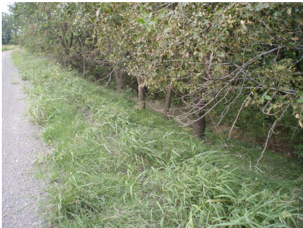
16. EXTERIOR OF NORTHWESTERN PORTION OF PERMETER DIKE (AREA 4) - MULTIPLE TREES OBSERVED ON EMBANKMENT
