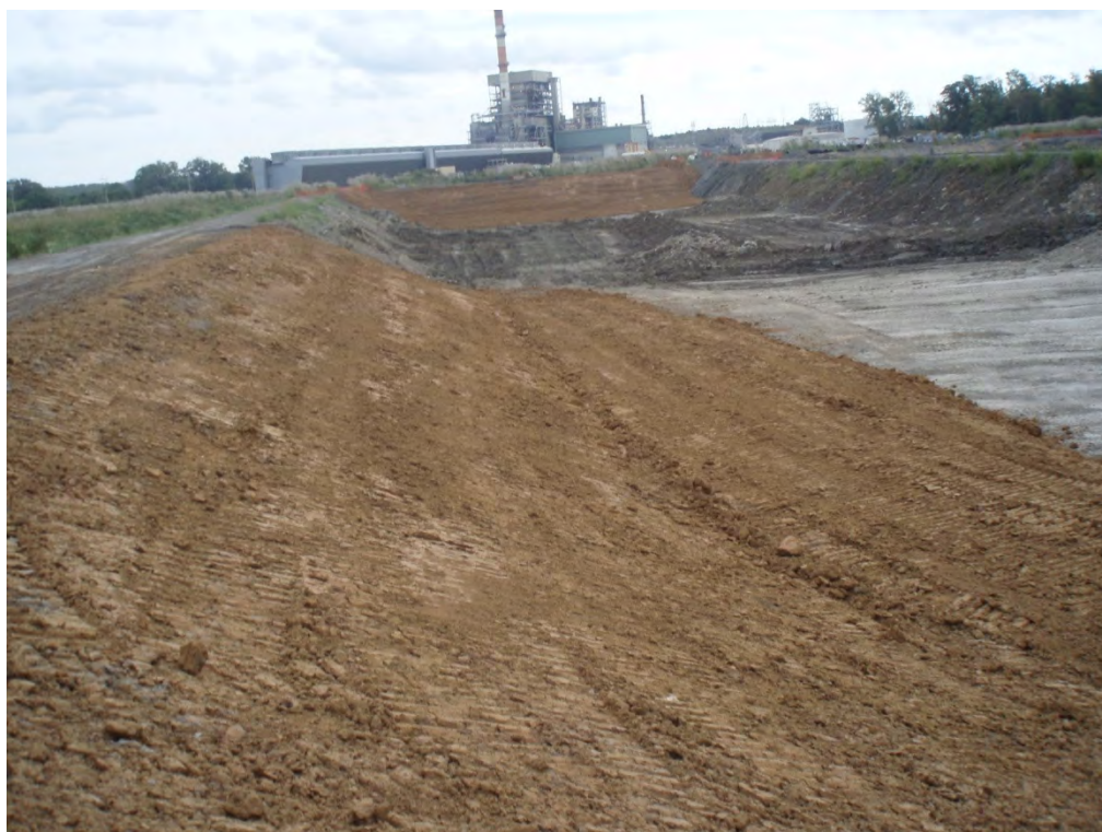
21. INTERIOR SEPARATION DIKE (AREA 3) - TAKEN FROM WESTERN PORTION OF PERMETER DIKE LOOKING EAST ALONG INTERIOR SEPARATION DIKE. CLAY LINER BEING INSTALLED
