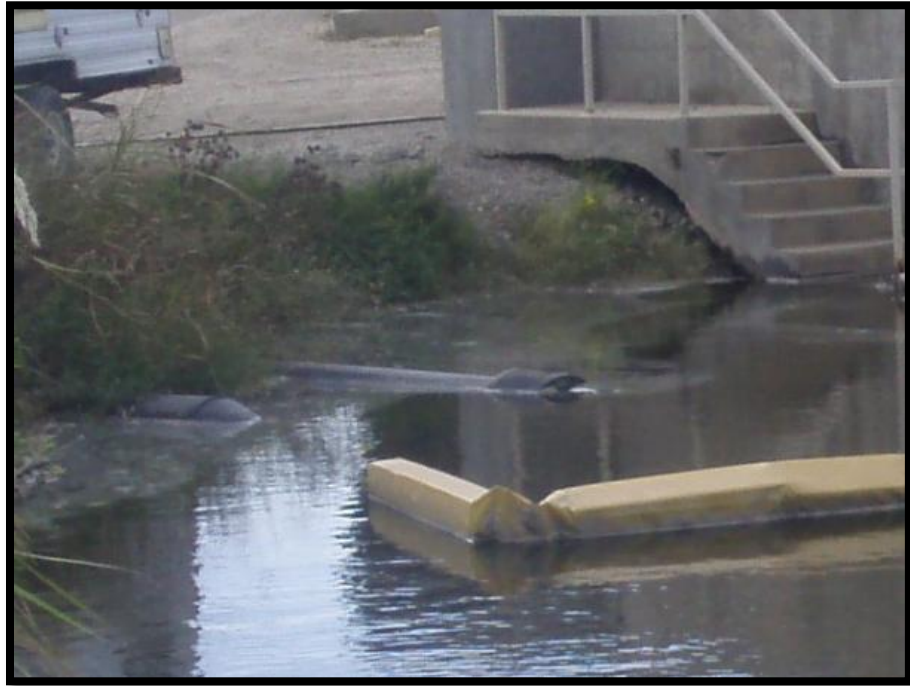
Figure 5.5.2-1: Inlet end of the Area 1 Outlet Structure that leads to the Kansas River.
