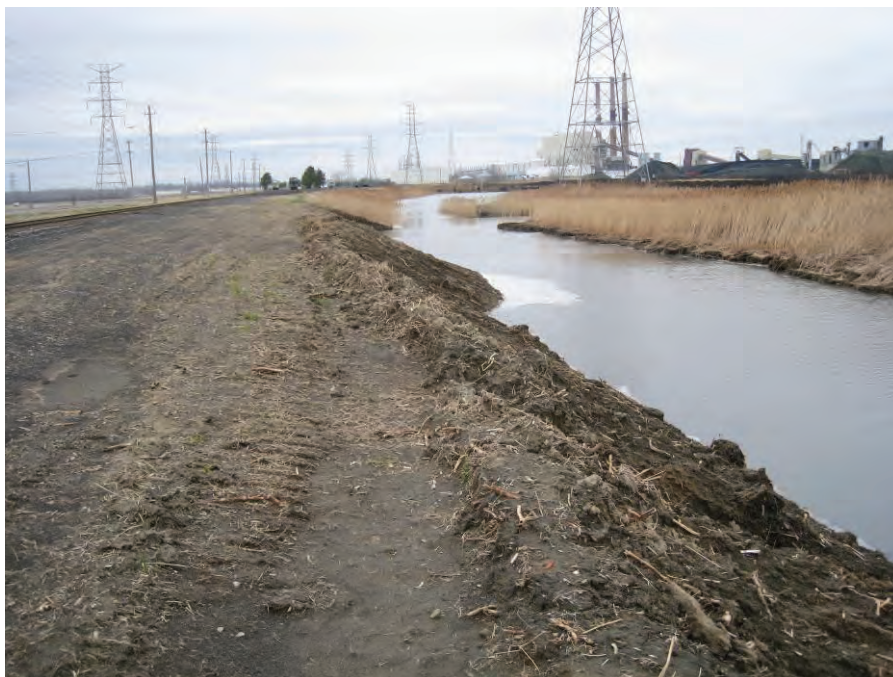
Drawing Mark EAP-1 Erosion is occurring on the interior slope along the south dike looking west.
