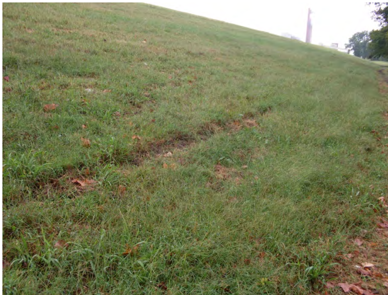
Photo 5.16: EAP Perimeter dike outside slope north side, looking west. Note mower rut.
