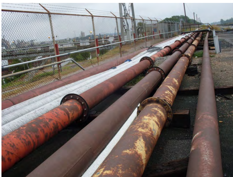
Photo 5.10: EAP View of ash sluice lines and plant process water line (leftmost) extending from the plant to the active pond, looking east. Rightmost line is abandoned.
