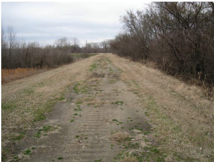
Drawing Mark WAP-3 Dense trees and vegetation are growing on the exterior slope of the north dike.
