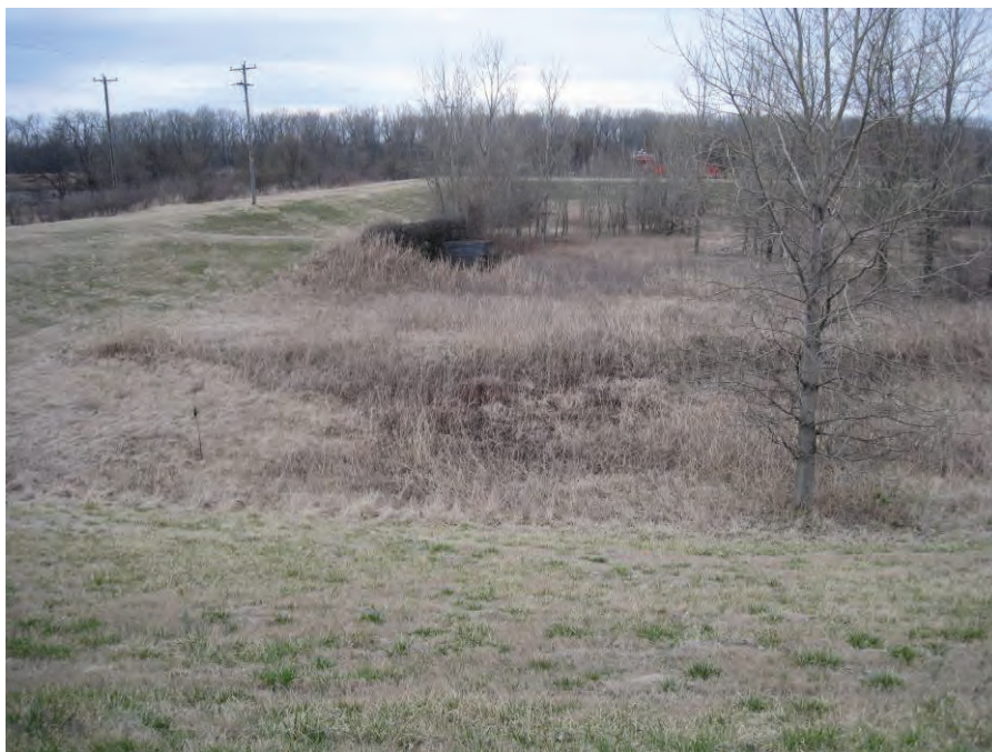
Drawing Mark WAP-1 Interior of Ash Pond mainly empty and covered with trees and dense vegetation.
