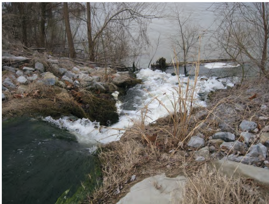
Drawing Mark EASP-7 Decant structure outlet into McKellar Lake has erosion occurring.
