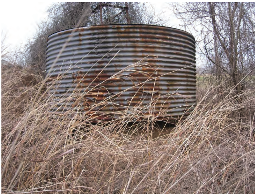
Drawing Mark WAP-4 Abandoned decant structure on west end of pond. Deteriorated and surrounded by heavy vegetation.
