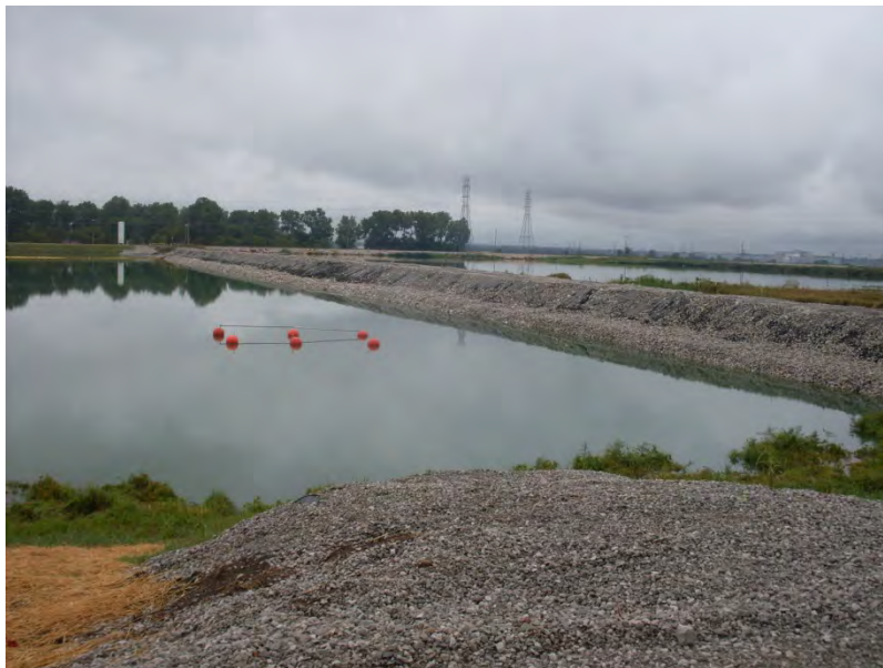
Photo 5.7: EAP Divider dike slope east side, looking southwest. Note minor gully erosion in slope above riprap blanket.
