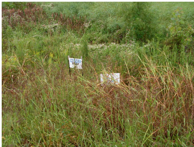
Photo 5.15: EAP Perimeter dike outside toe east side, identified seep area.
