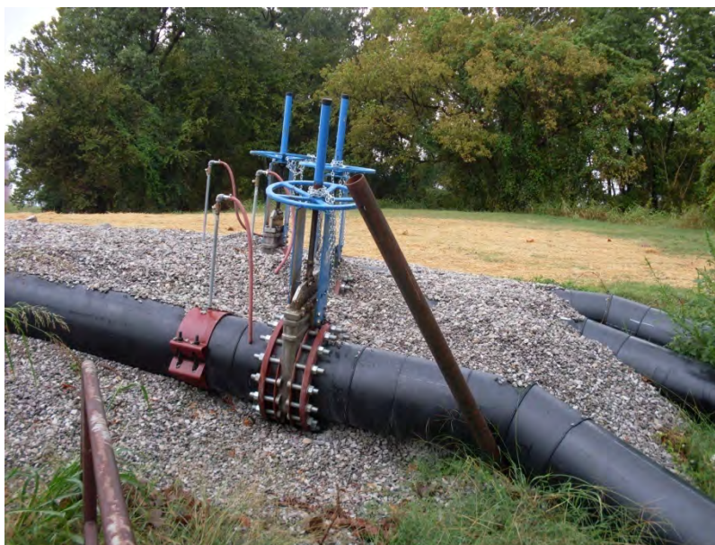
Photo 5.26: EAP Gate valves in siphons, looking west.
