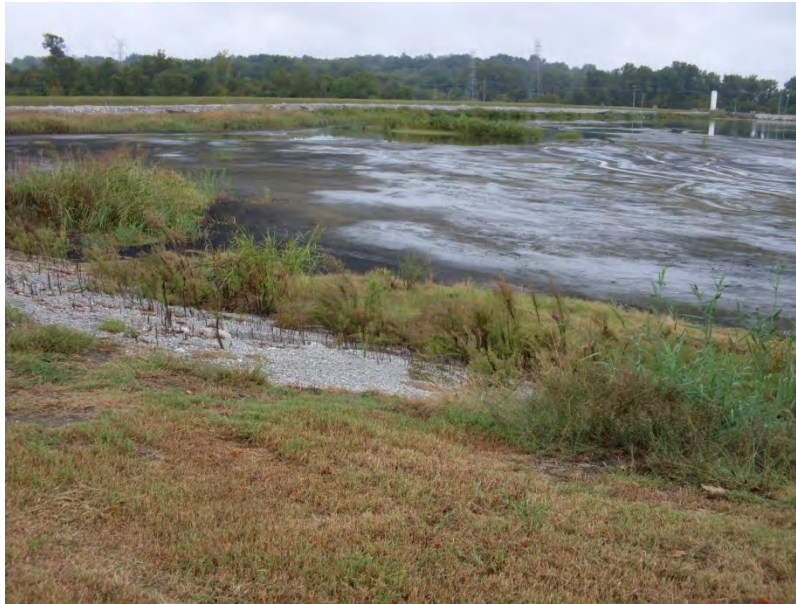
Photo 5.6: EAP Perimeter dike inside slope north side, looking east southeast in area of recent slump repair. Note crushed stone material used in the repair.
