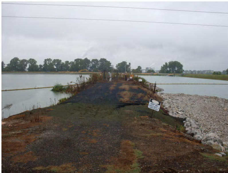
Photo 5.3: EAP Divider dike crest south end, looking north. Note gully erosion in the bottom ash embankment.
