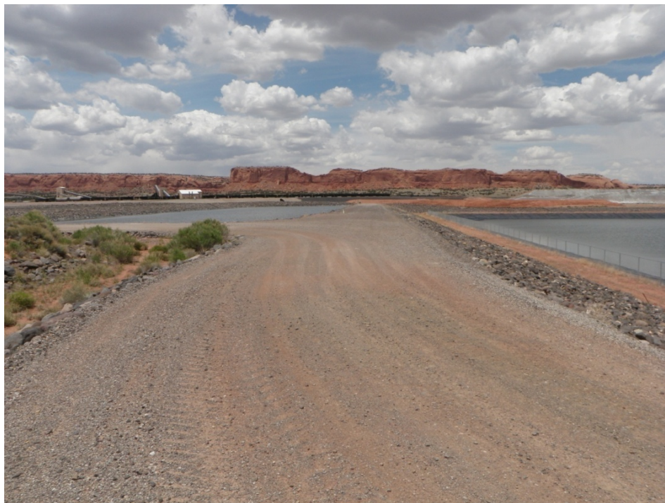
Photo 27: Evaporation Pond 4 (right) & Pond 3 (left) : Crest : Looking North along Pond 4 west dike
