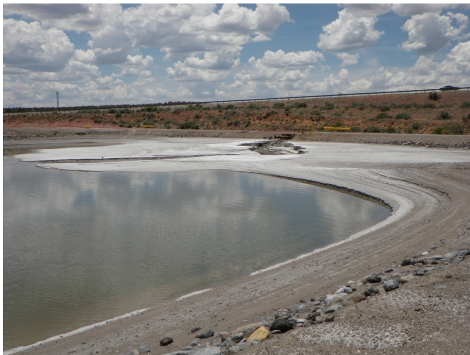
Photo 10: Bottom Ash Pond – North : Upstream Toe : Looking SW at Inlet pipes through the West Dike from the North Dike
