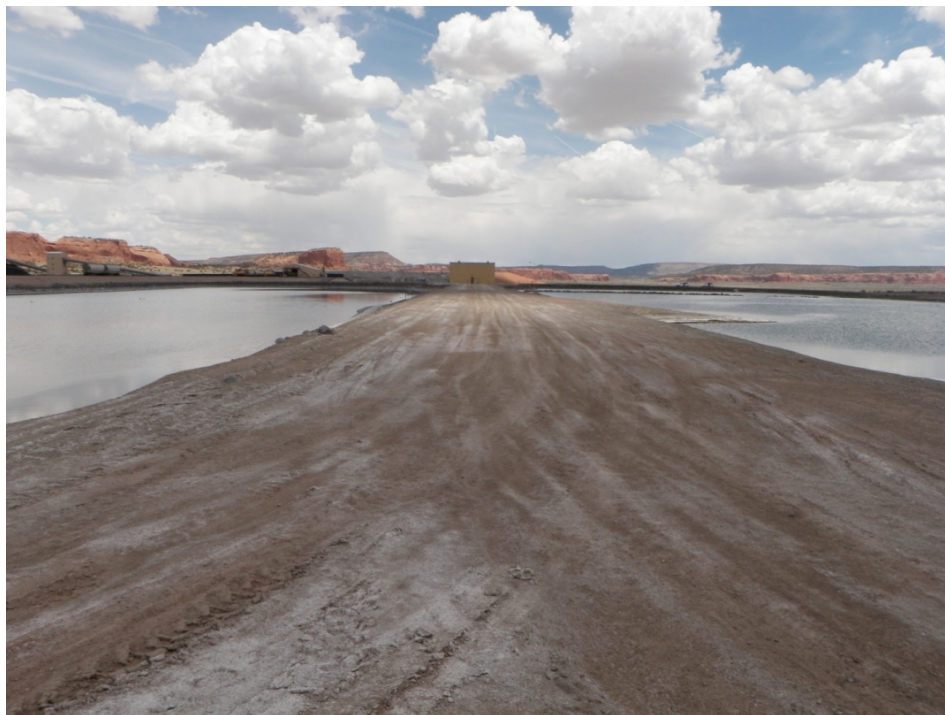
Photo 13: Bottom Ash Pond – North/South : Crest : Looking East along the Dike dividing the North and South Ponds. South Pond on the right- North Pond on the left.
