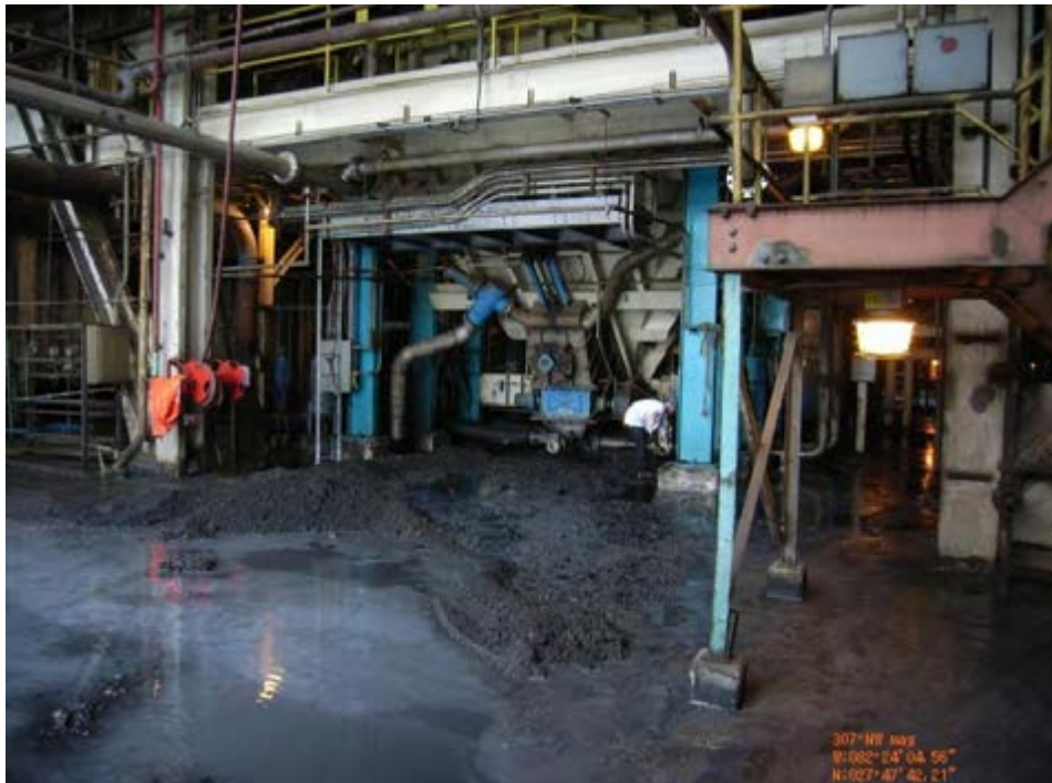
Boiler where boiler slag is collected
