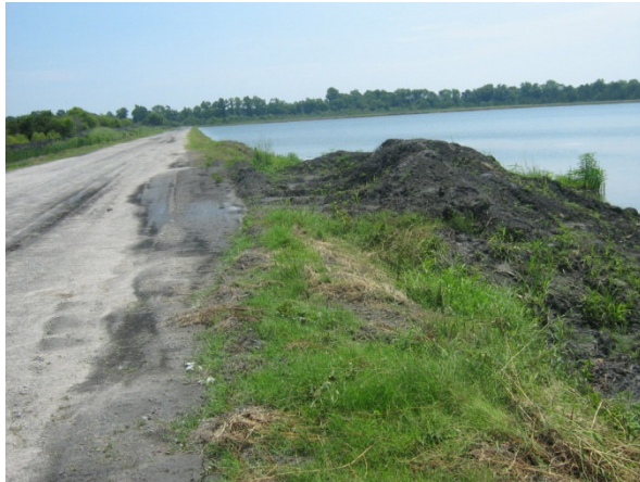
Photo 044: Internal Dike Slope
