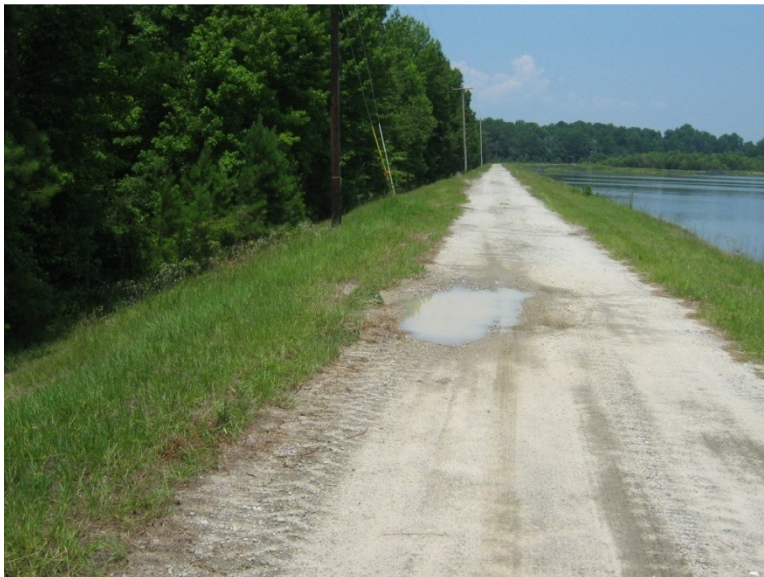
Figure 5.2.1: Ash Pond 2 Crest – Water Ponding
