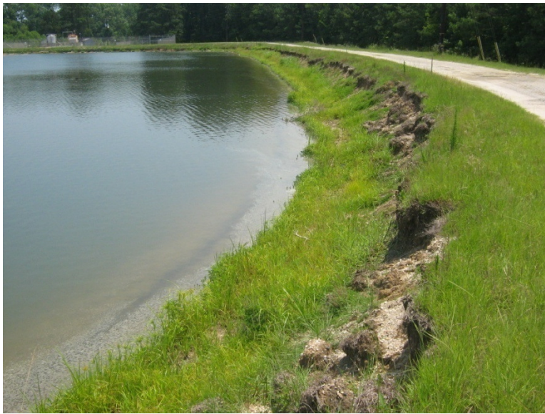
Figure 5.2.2: Ash Pond 2 Upstream Slope Erosion
