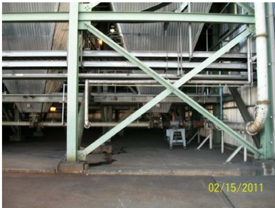
Hopper feeding ash sluice line
