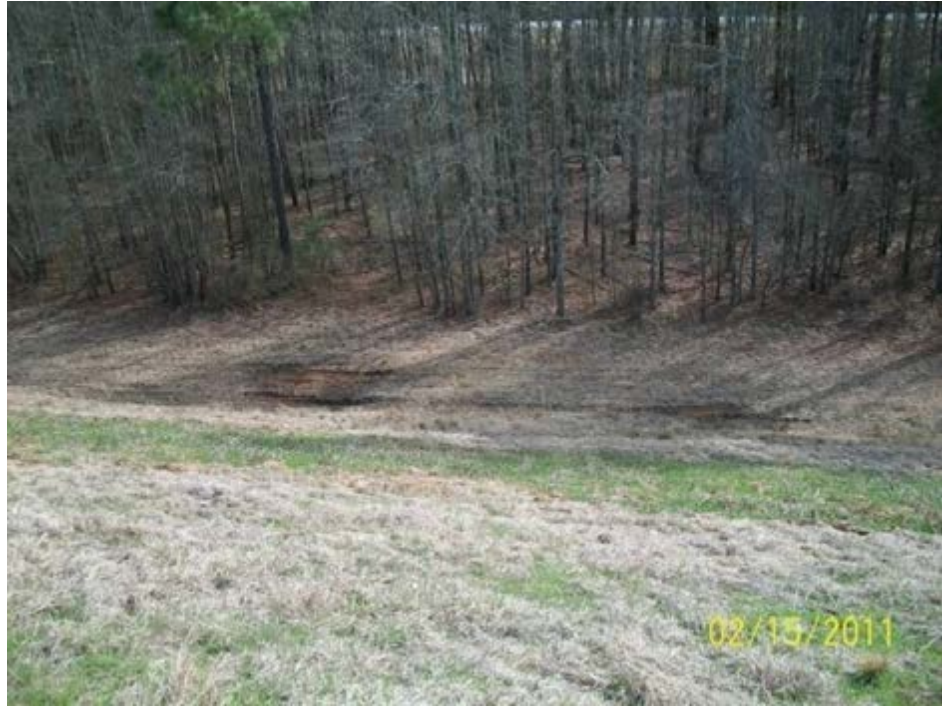
Photo 1. Standing water in vehicular traffic ruts
