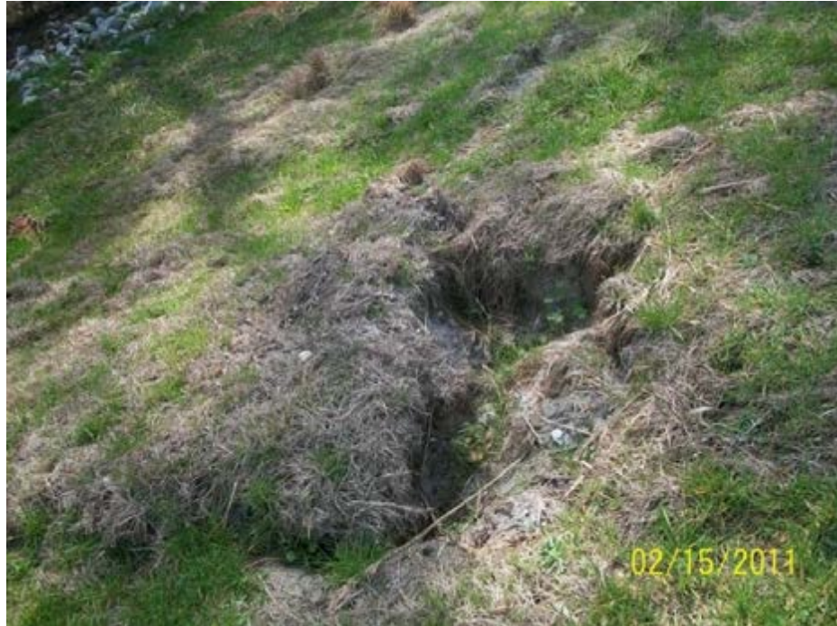
Photo 3. Surficial sloughing along downstream slope
