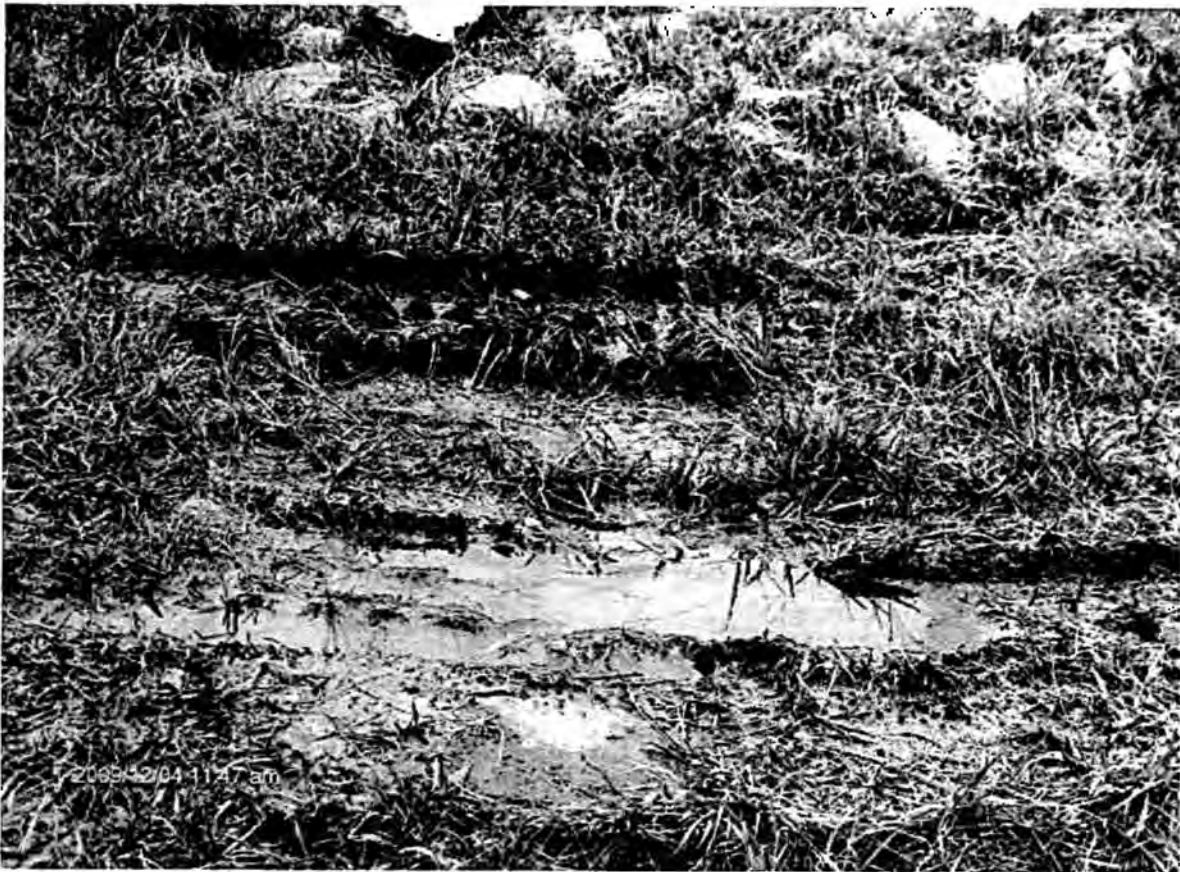
Figure 7: Example of Area of Standing Water along Toe of Active Pond West Berm
