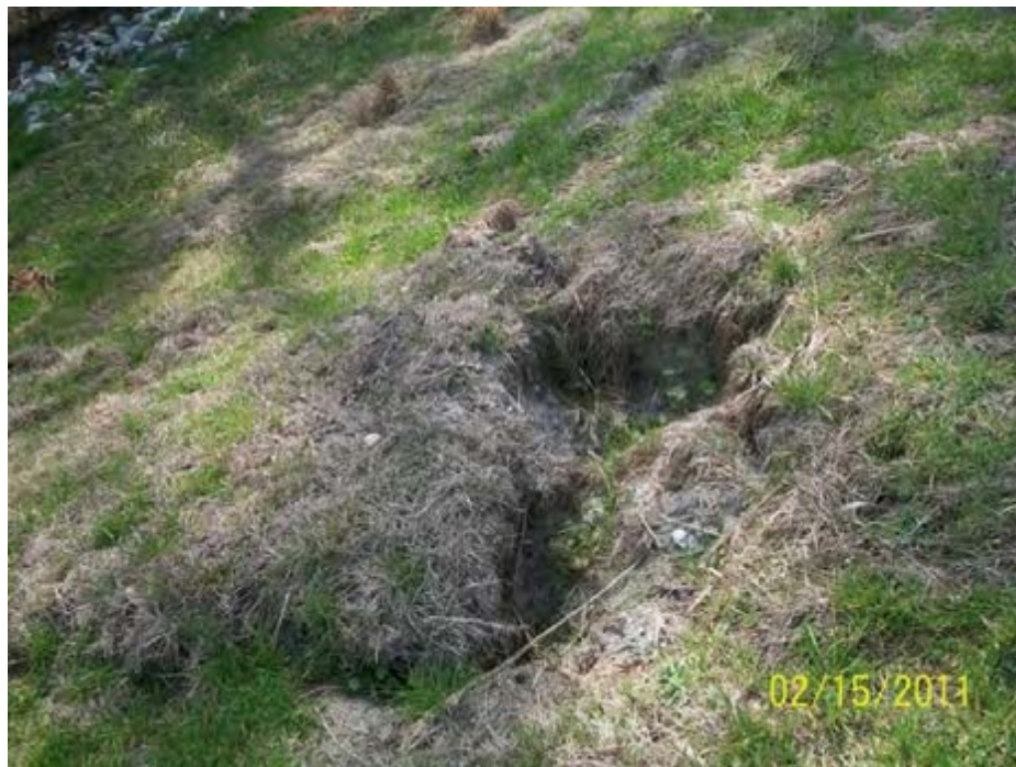
Photo 3. Surficial sloughing along downstream slope
