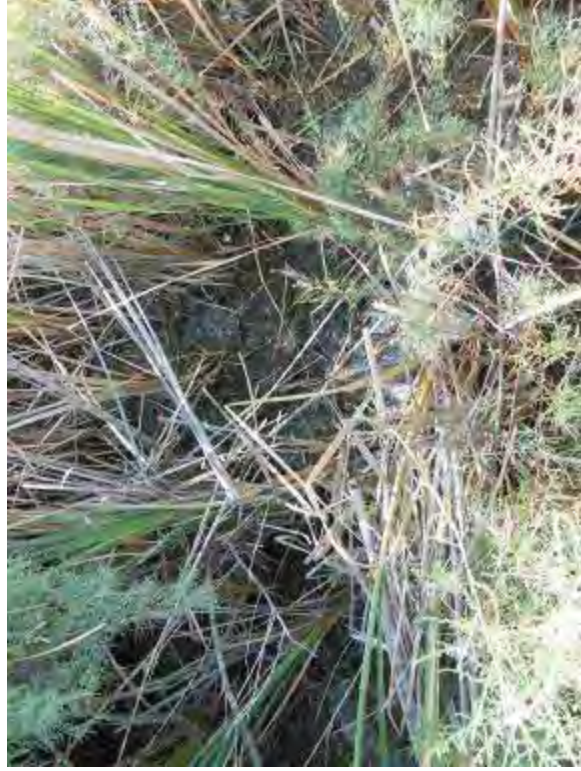
Photo 57: Wet area at west embankment exterior slope.
