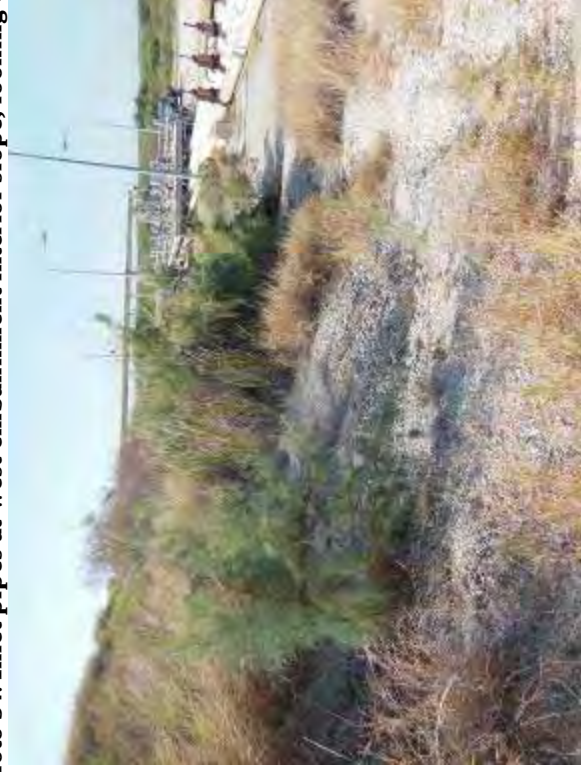
Photo 56: West embankment exterior slope, looking south. Note cattails and other vegetation growing near toe.
