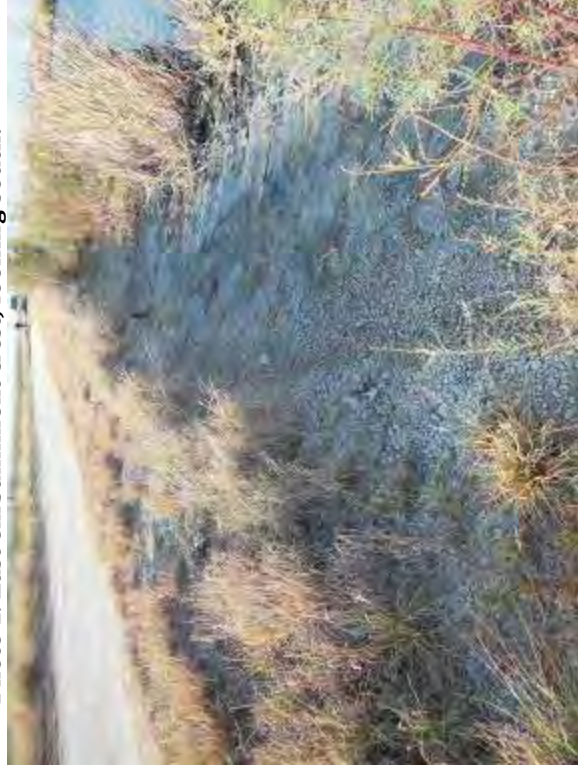
Photo 3: East embankment exterior slope, looking south. Note slope erosion.
