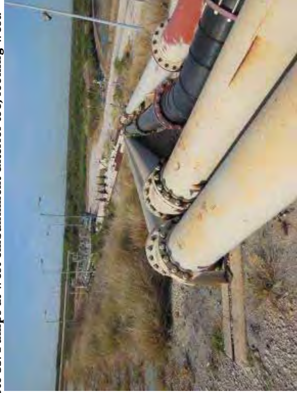
Photo 55: Piping from Plant to pumps at west embankment exterior slope, looking southwest.
