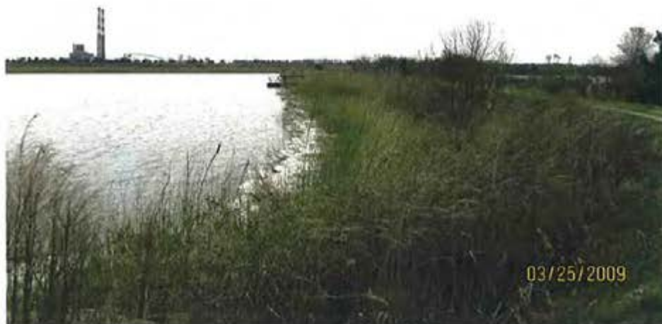
9. 1984 Ash Pond – View of interior slope of dike on west side of pond looking toward discharge riser.
