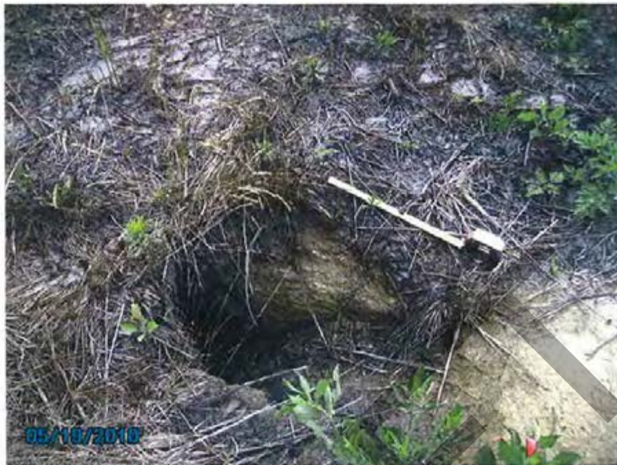
17. 1984 Ash Pond – View of animal burrow on the exterior slope for east dike (12 inch tape extension shown for scale).
