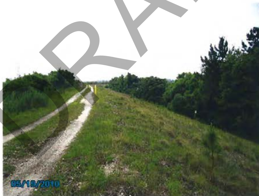
14. 1984 Ash Pond – View of exterior slope for west dike looking toward discharge structure.
