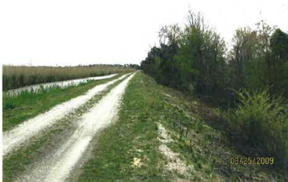
4. 1983 Ash Pond – View of crest and exterior slope adjacent to discharge canal.
