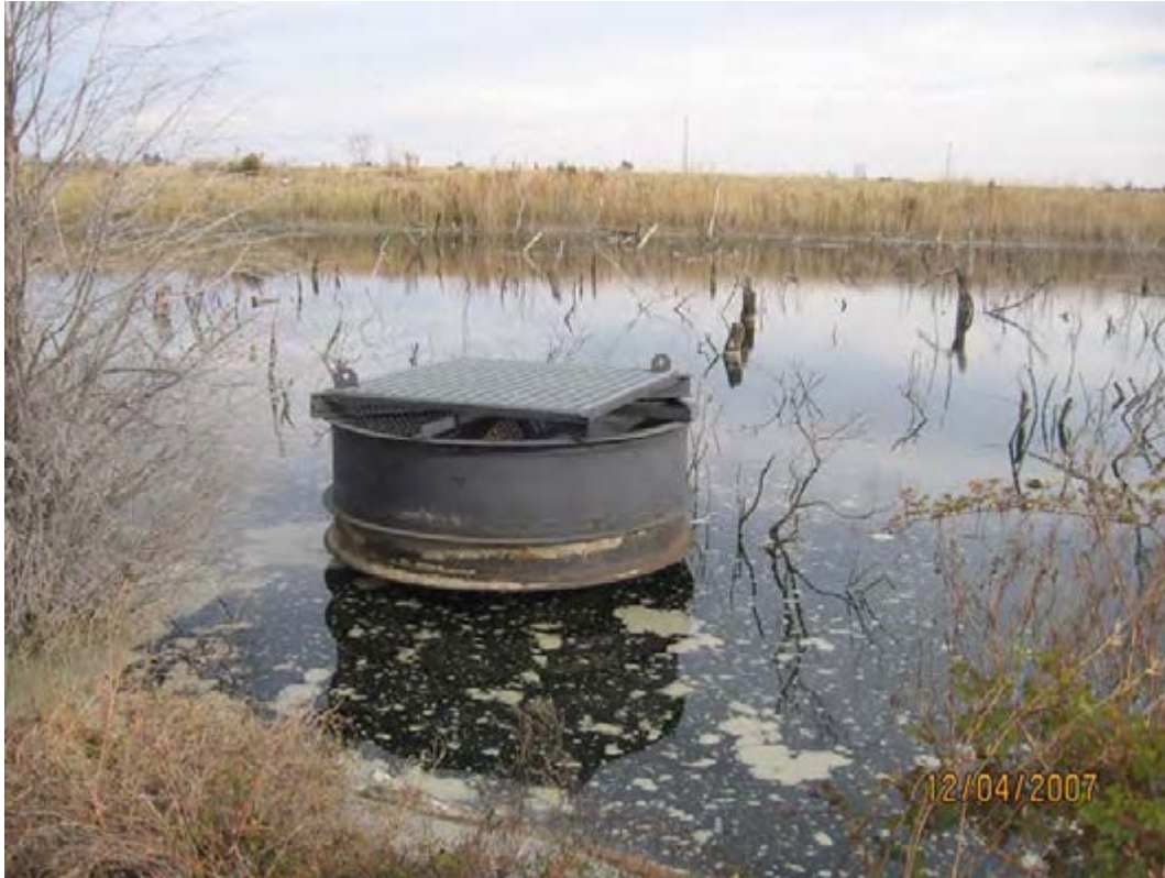
Photo 1. 1983 Ash Pond – Outlet riser and pond water.
