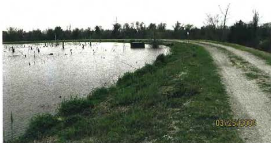
1. 1983 Ash Pond – View of interior slope, outlet riser and standing water near riser.
