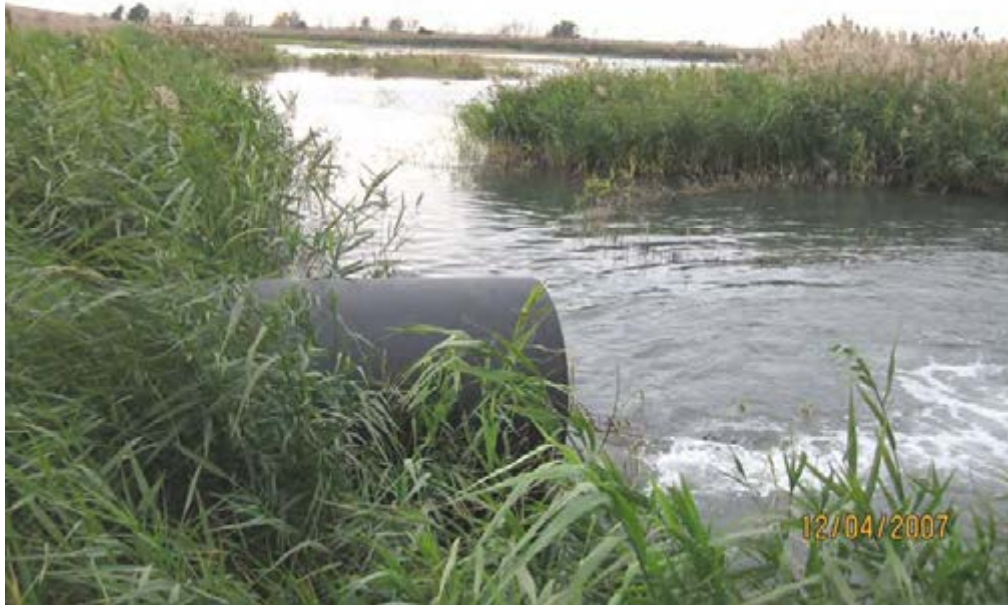
Photo 9. 2006 Outlet Pipe draining into 1984 pond.
