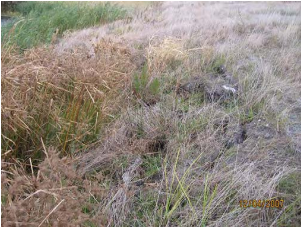
Photo 12. 2006 interior Ash Dike – Area of erosion of ash along exterior slope of dike.
