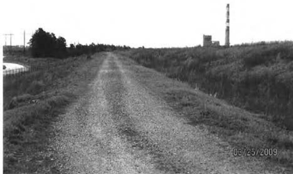
6. 1984 Ash Pond -- View of dike crest and exterior slope on east side of pond
