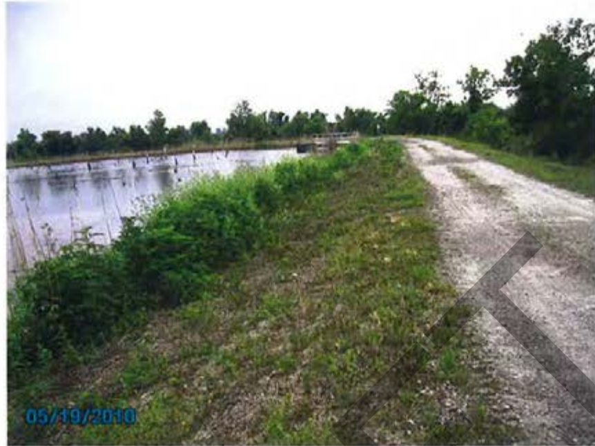
1. 1983/1971 Ash Pond – View of interior slope for west dike looking toward discharge structure.
