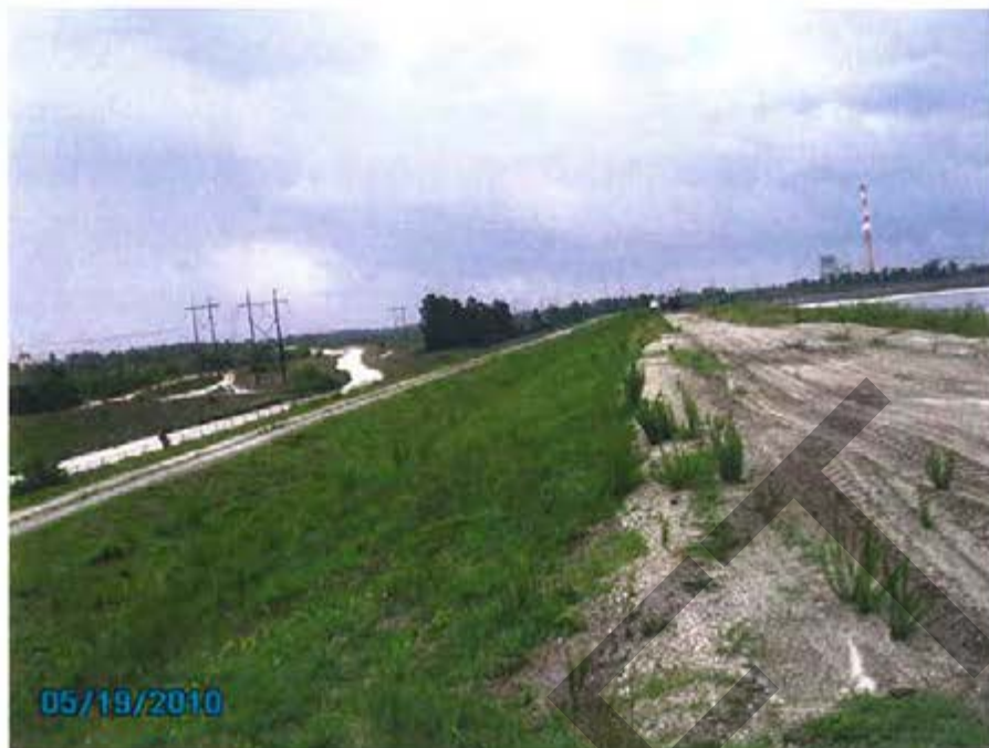
7. 1984 Ash Pond – View of exterior slope for east dike looking south (at northeast corner).
