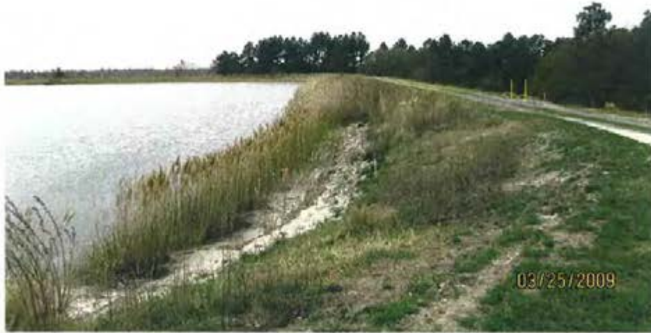
7. 1984 Ash Pond - View of riprap placed for interior slope on north side of pond.
