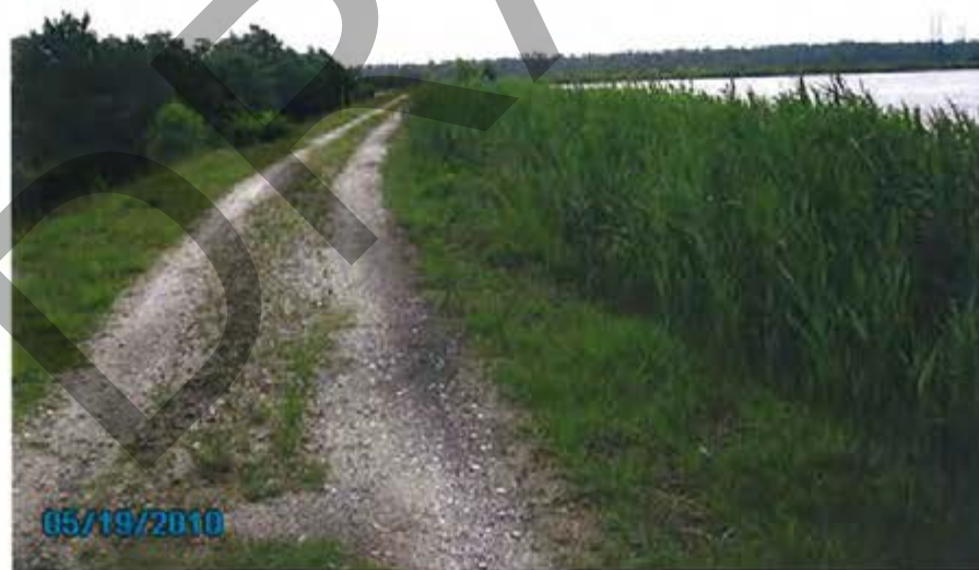
12. 1984 Ash Pond – View of exterior slope for south dike looking east (at northwest corner).
