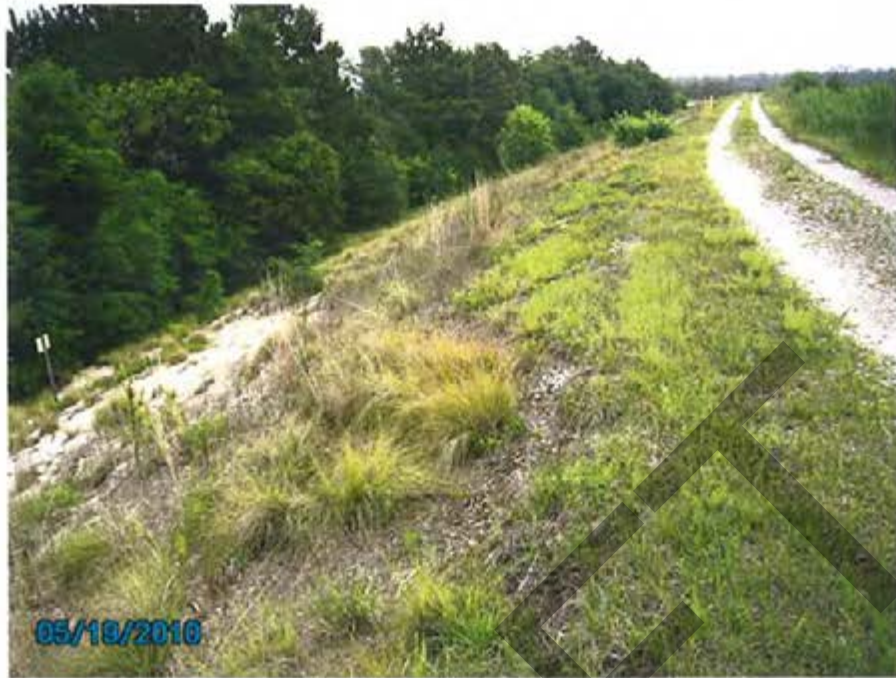
11. 1984 Ash Pond – View of exterior slope for south dike looking toward east (at northwest corner).
