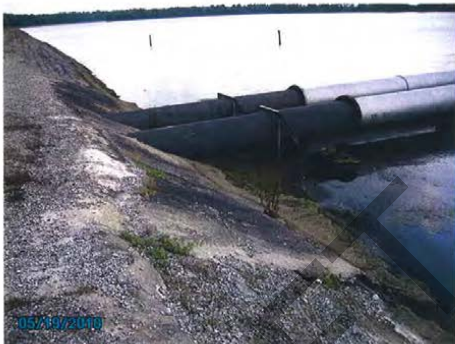
32. Cooling Pond – (Bay #4) View of makeup discharge pipes on upstream side of dike.
