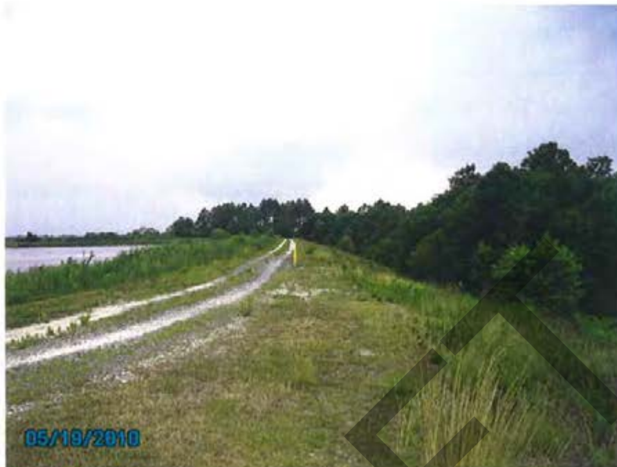
9. 1984 Ash Pond – View of exterior slope for south dike looking west (at northeast corner).
