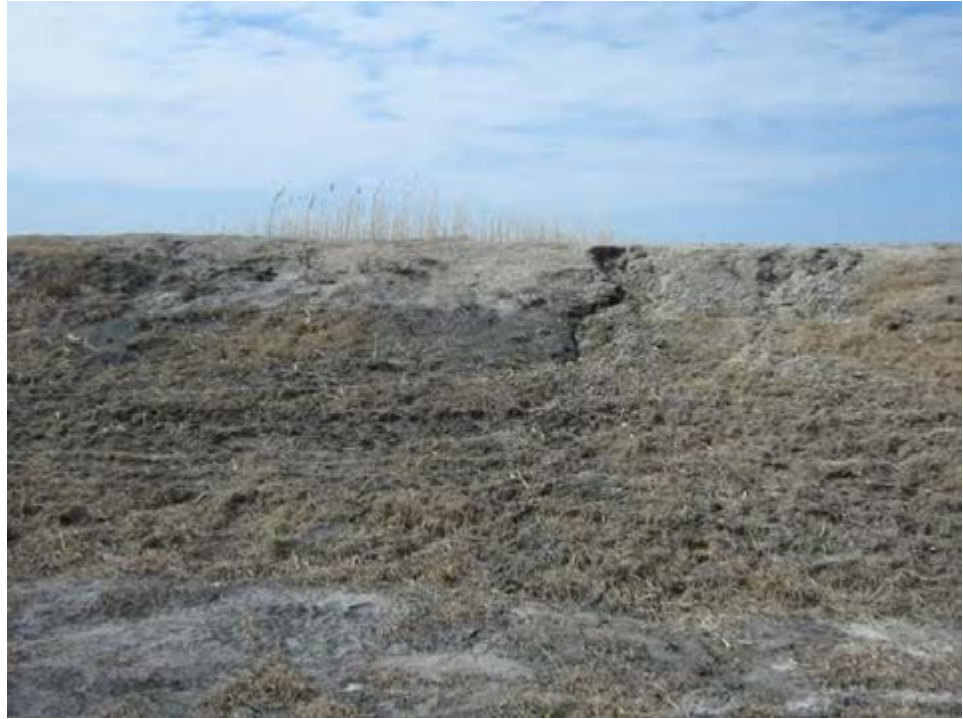
Rill erosion along downstream slope, 1984 Ash Pond
