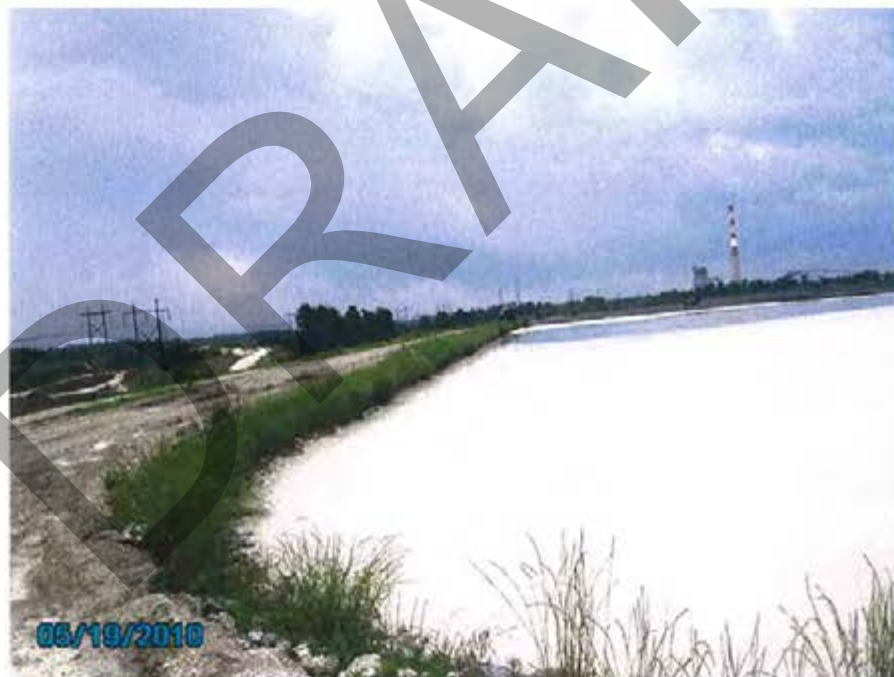
22. 1984 Ash Pond/Interior Storage – View of interior slope for containment dike looking south.
