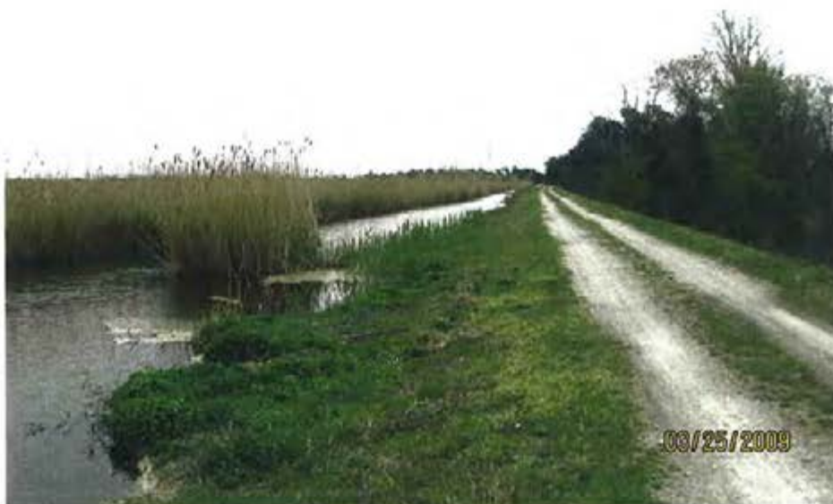
3. 1983 Ash Pond – View of crest, interior slope and standing water adjacent to discharge canal.
