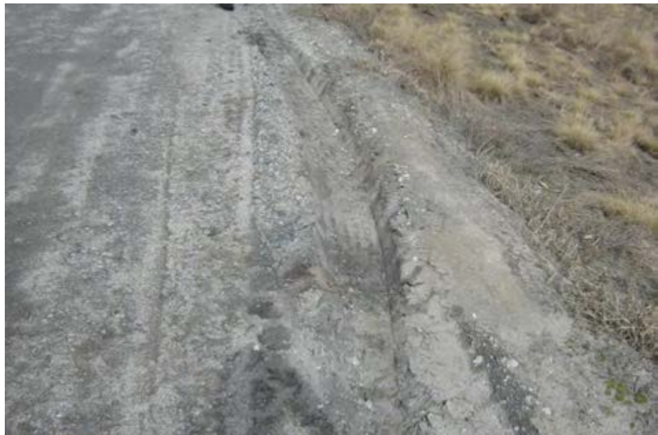
Vehicular rutting along crest
