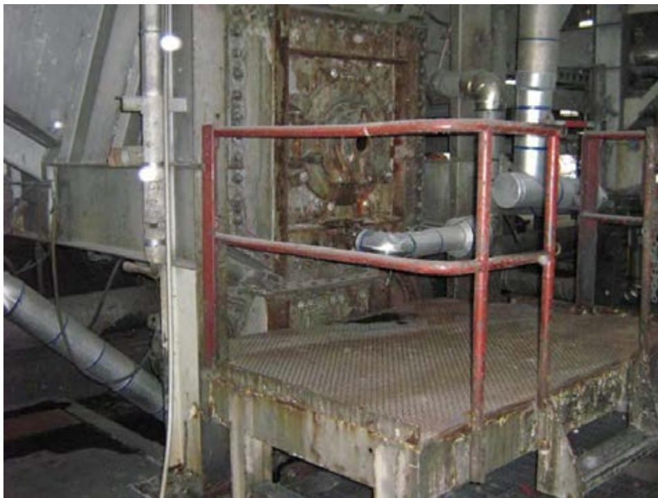
Location from where boiler slag is piped
