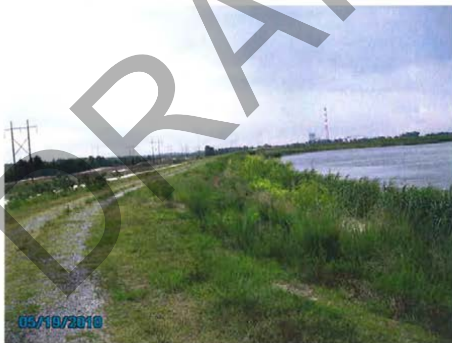
8. 1984 Ash Pond – View of interior slope for east dike looking south (at northeast corner).
