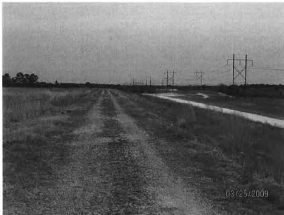
5. 1984 Ash Pond – View of dike crest and exterior slope east side of pond
