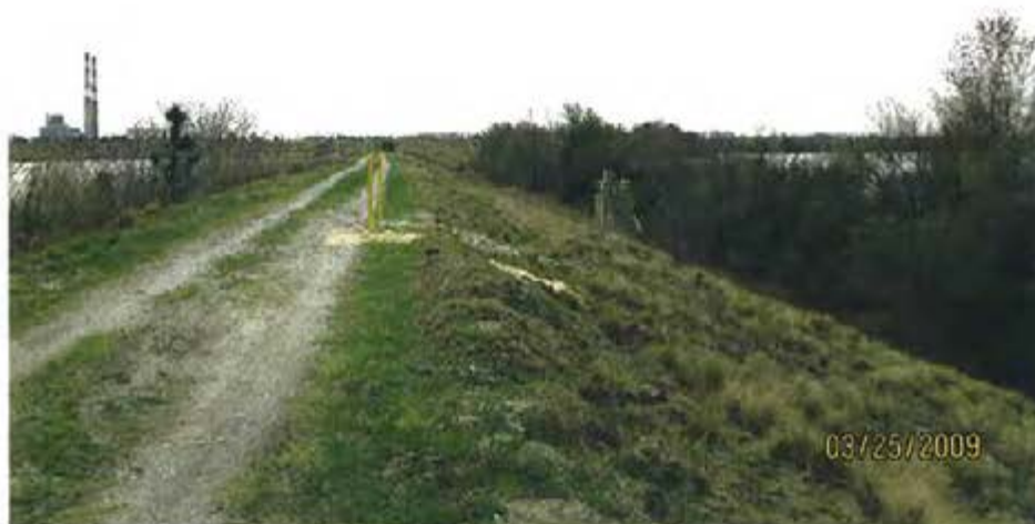
10. 1984 Ash Pond – View of exterior slope of dike on west side of pond looking toward outlet structure.
