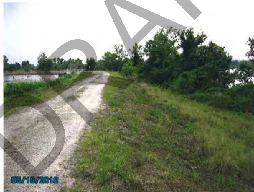
2. 1983/1971 Ash Pond – View of exterior slope for west dike looking toward discharge structure.
