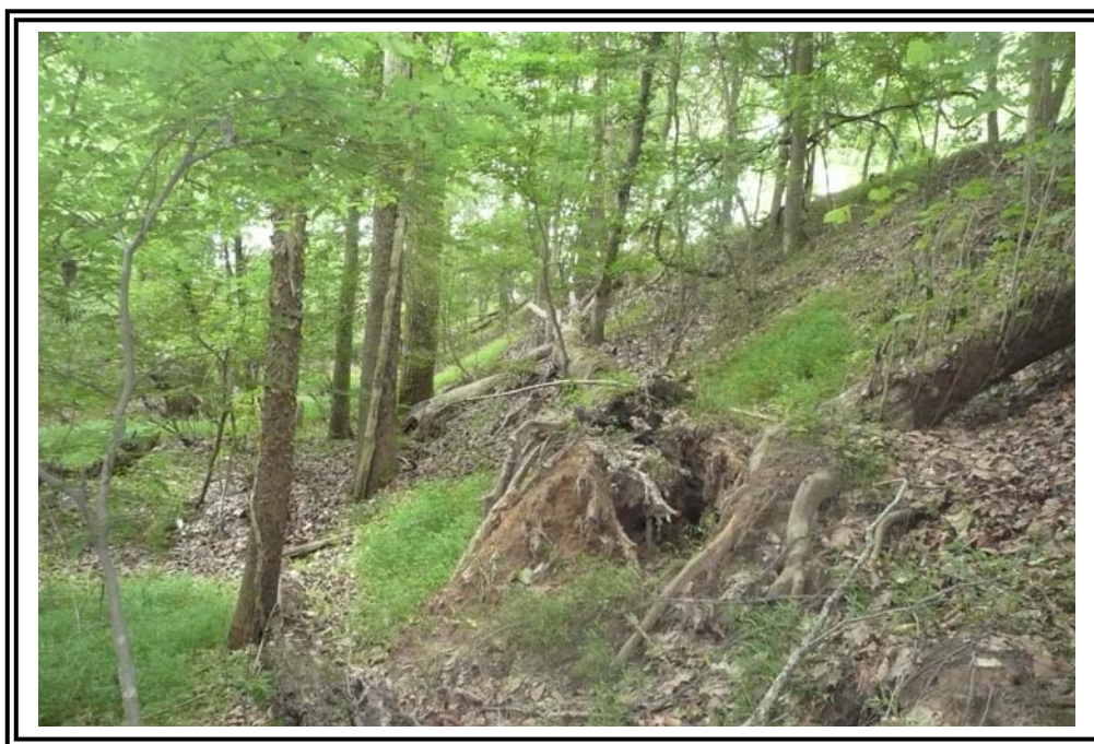
Uprooted tree on the 1956 Ash Pond Dike.
