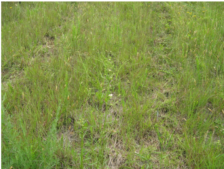
Photo 18: 1982 Dam – Minor Rill Erosion, Downstream Embankment, Photo: 033, 5/29/09
