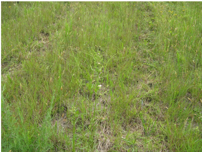
Photo 18: 1982 Dam – Minor Rill Erosion, Downstream Embankment, Photo: 033, 5/29/09
