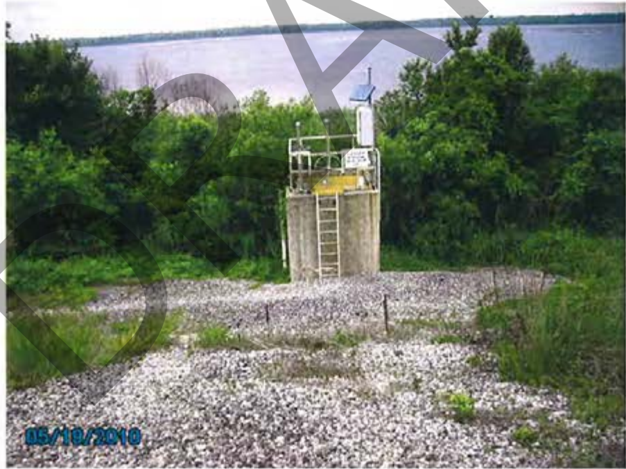
20. 1984 Ash Pond – View of discharge diversion structure at toe of west dike.
