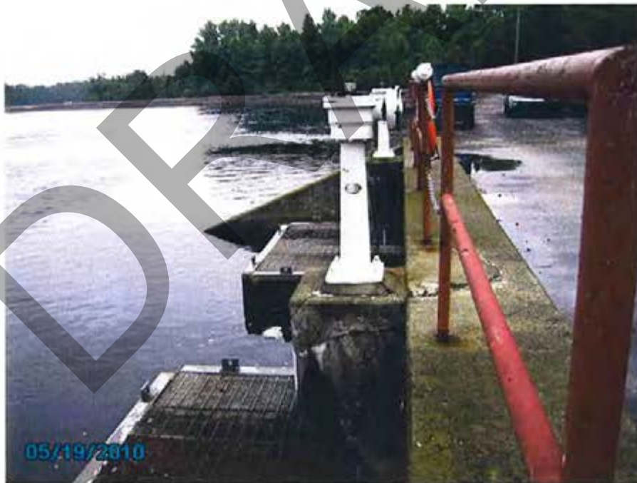
40. Cooling Pond – View of concrete cracking at sluice gate support on north side of discharge structure.
