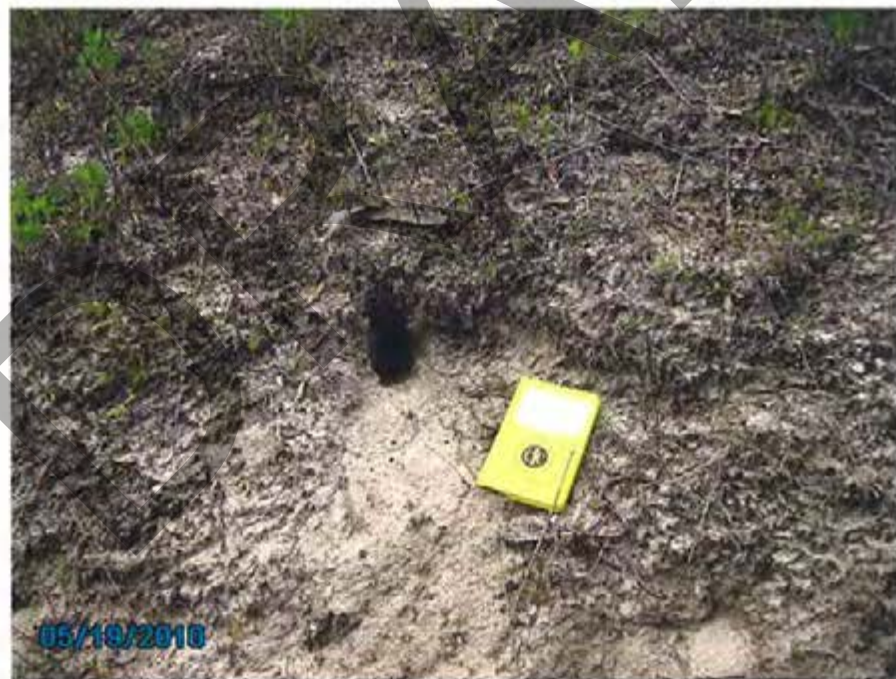
18. 1984 Ash Pond – View of animal burrow on the exterior slope for north dike (4" x 7" field book shown for scale).
