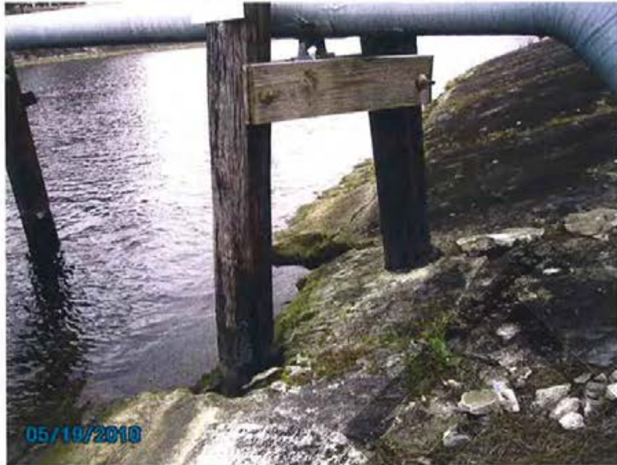
39. Cooling Pond – View of slope protection damage at pipe support on interior slope near the sluice gate structure.
