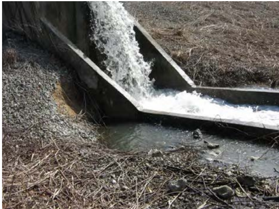
Concrete outfall of 1984 Ash Pond where undercutting is present
