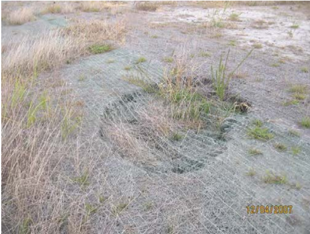
Photo 11. 2006 interior Ash Dike –Exterior Slope looking a sink hole.
