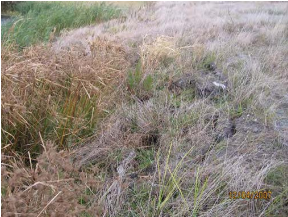
Photo 12. 2006 interior Ash Dike – Area of erosion of ash along exterior slope of dike.
