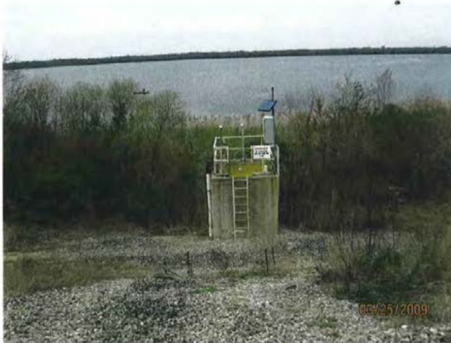
12. 1984 Ash Pond – View of top for discharge structure looking toward cooling pond.
