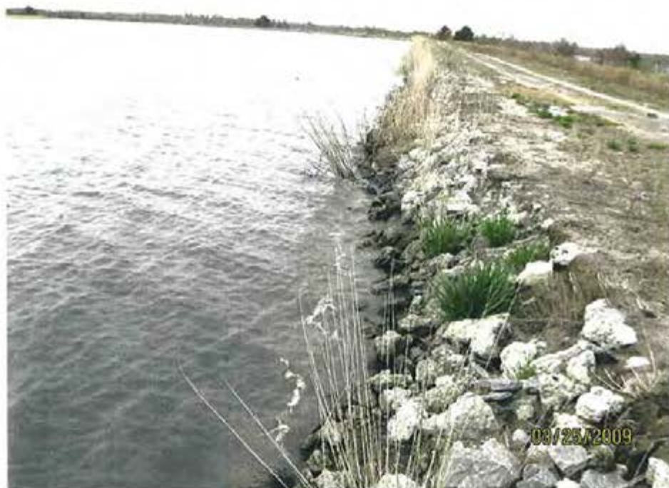
17. 1984 Ash Pond (Interior Storage Area) – View of riprap along interior slope on north side of pond.
