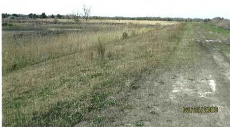
18. 1984 Ash Pond (Interior Storage Area) – View of exterior slope on south side of pond.
