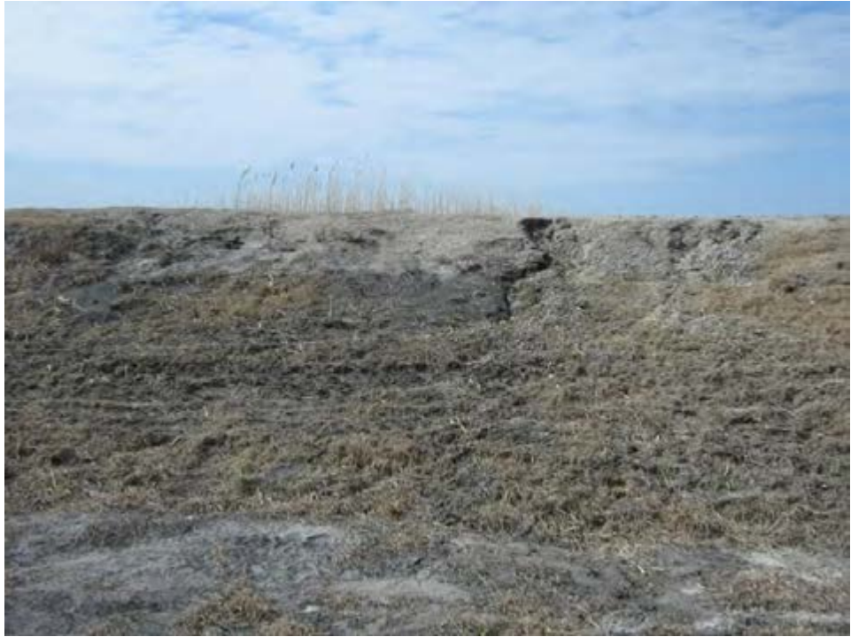
Rill erosion along downstream slope, 1984 Ash Pond
