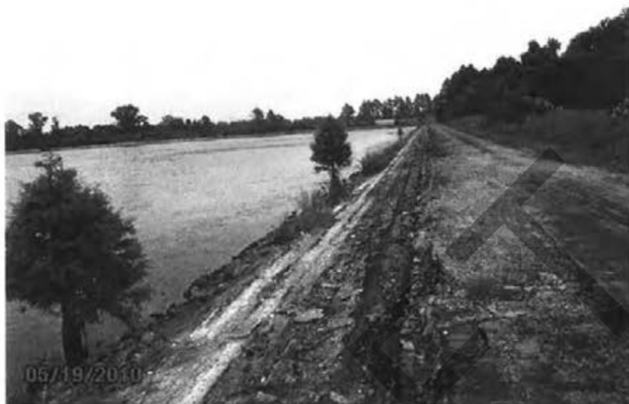
26. Cooling Pond – (Bay #1) View of crest and interior slope showing small trees growing at toe.
