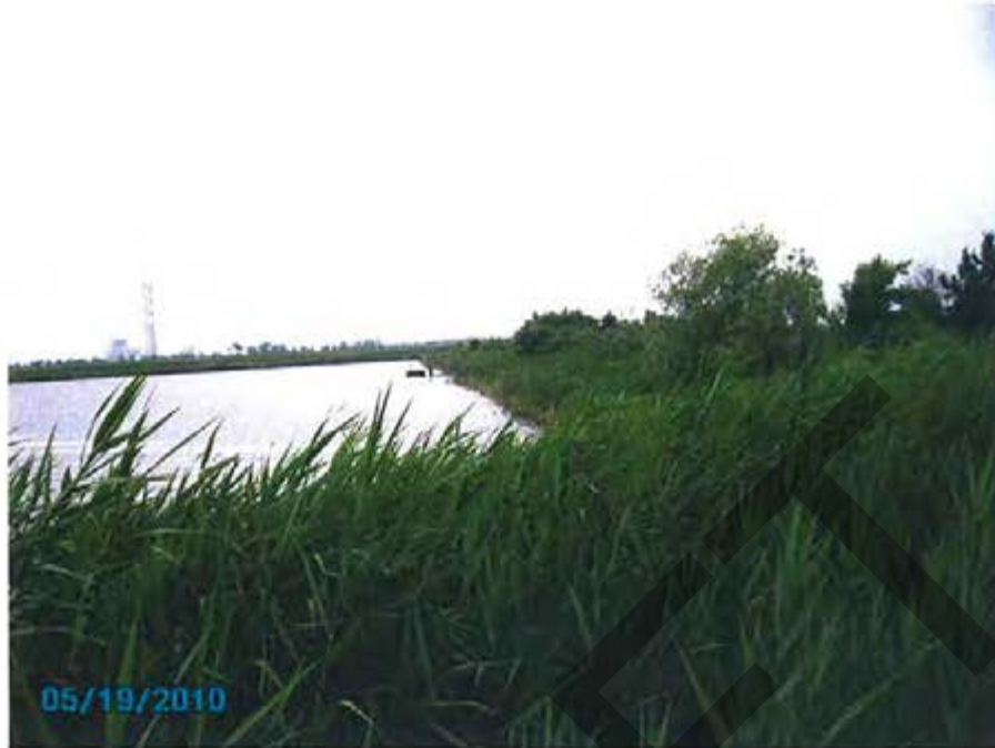
13. 1984 Ash Pond – View of interior slope for west dike looking toward discharge structure.
