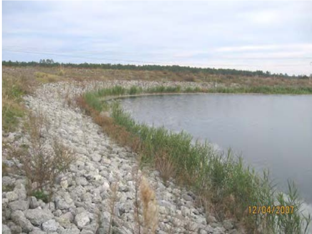
Photo 6. 1984 Ash Pond – Interior slope newly repaired with rip rap. Typical of section with good rip rap.
