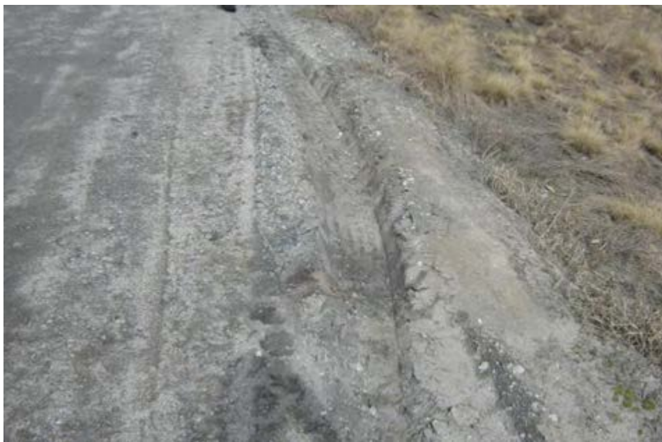
Vehicular rutting along crest
