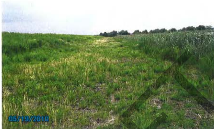
23. 1984 Ash Pond/Interior Storage – View of stability berm for containment dike looking west.
