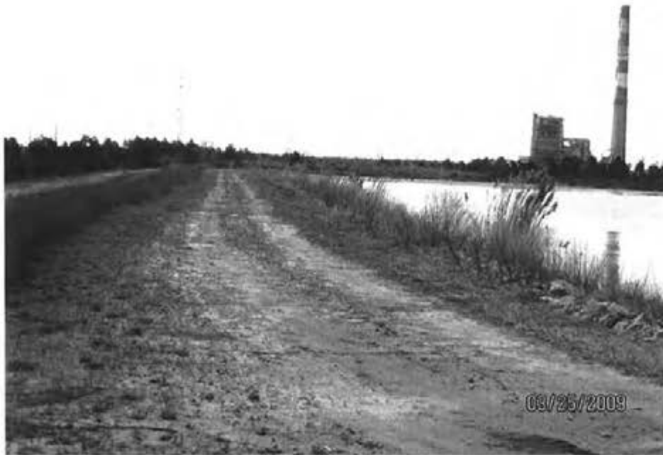
15. 1984 Ash Pond (Interior Storage Area) – View of crest of dike and interior slope along east side of pond.
