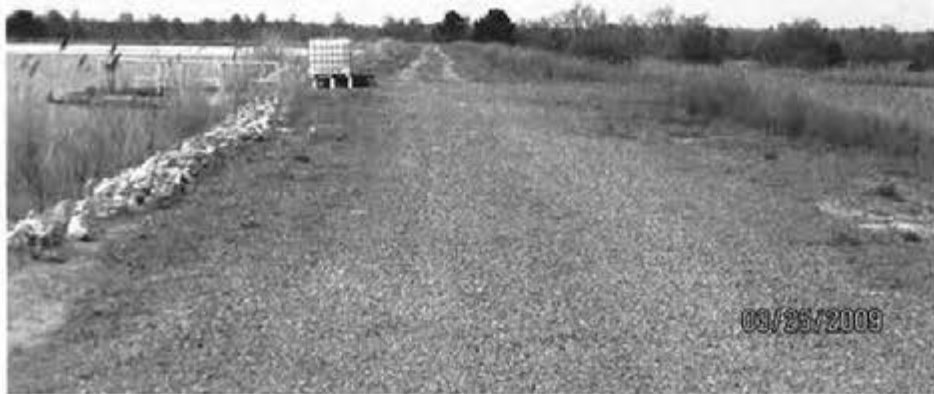
13. 1984 Ash Pond (Interior Storage Area) – View of dike crest looking toward discharge structure on north side of pond.
