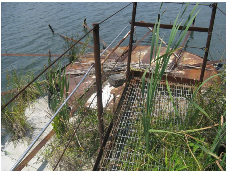
Photo 9: riser and skimmer at stilling pool, Photo: 079, 6/3/09
