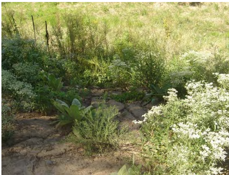
Figure 5.2.3b: Erosion along Downstream/Outside Slope of North Ash Pond dike.
