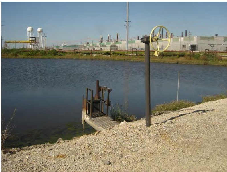
Figure 5.4.1: Overflow Structure of South Ash Pond (note control valve for decant pipe system in foreground).
