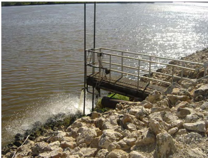
Figure 5.4.2: Outlet Conduit for South Ash Pond (note presence of overflow pipe outlet).
