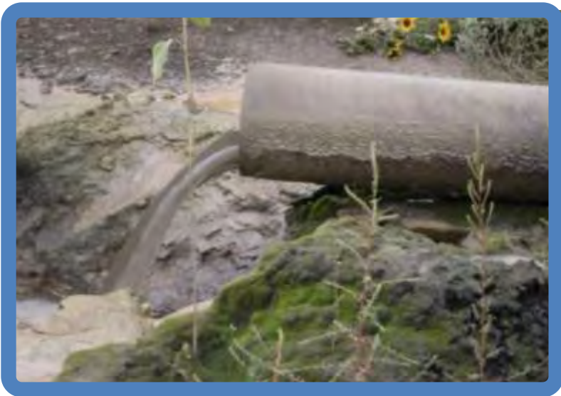
Photo 2.15 Pond 2 ash sluice discharge pipe
