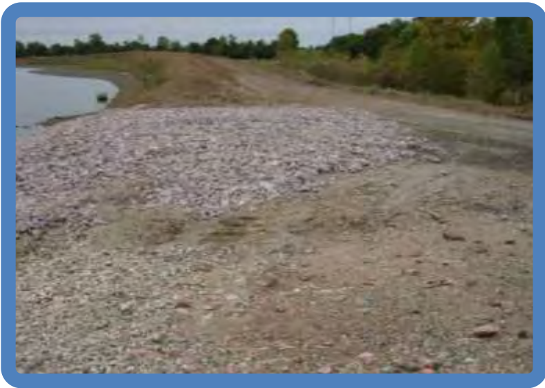
Photo 3.5 Pond 3B South dike inside slope (S side viewed NE) -low crest
