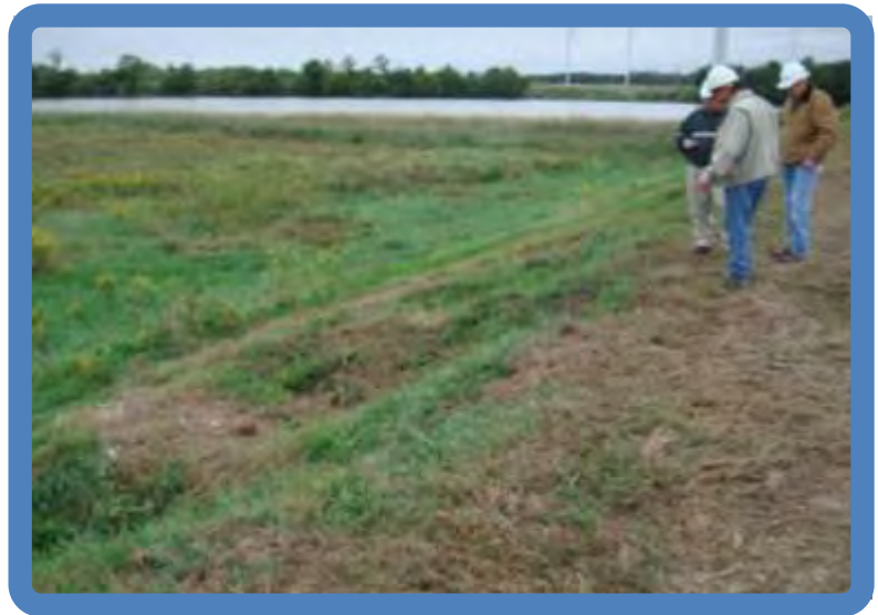
Photo 3.8 Pond 3B North dike outside slope (NE side viewed SE) -note erosion holes
