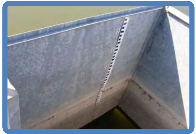
Photo 4.2 Pond 3B South Skimmer Box with staff gauge
