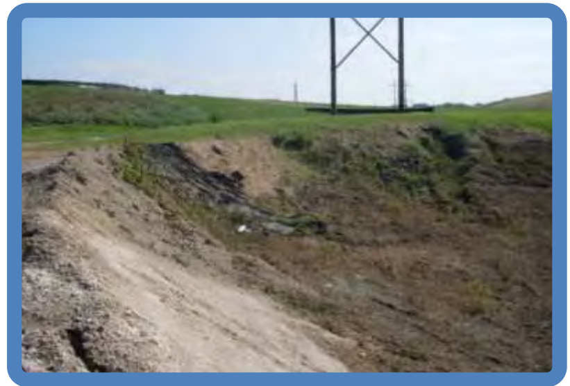
Photo 2.12 Pond 3A dike outside slope (SW segment viewed SE) -note erosion repair area
