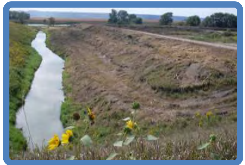
Photo 2.8 Pond 2 dike outside slope and outlet channel (SE side viewed SW from fill ramp to landfill)
