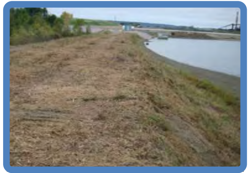
Photo 3.6 Pond 3B South dike crest and inside slope (S side viewed SW)
