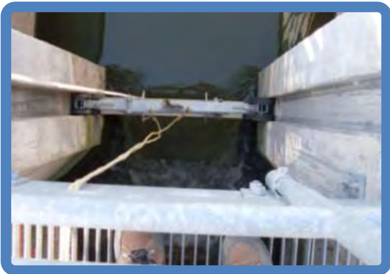
Photo 4.3 Pond 3B South Stop-log Structure adjustable weir
