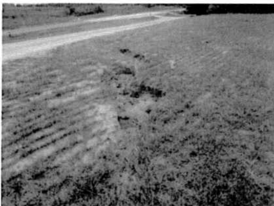
Figure 77: Erosion at South Access Ramp
