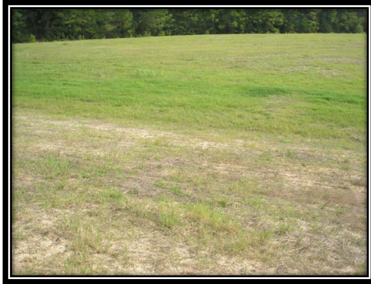
Figure 5.4.4-1 South groin of PDP-5.
