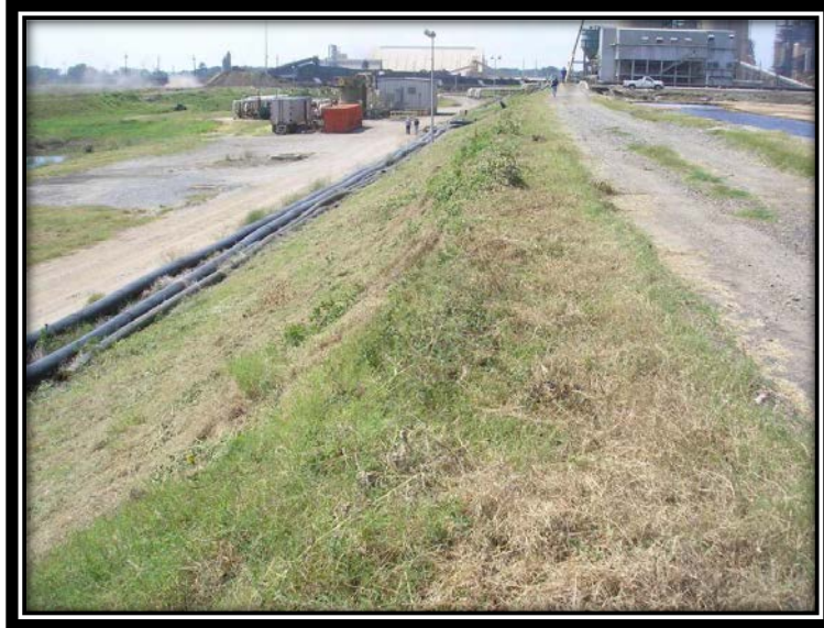
Figure 5.2.3-3 Ash Disposal Pond West cell south dike exterior slope.
