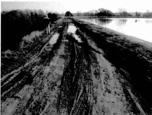
Figure 5: Crest Rutting North Side
