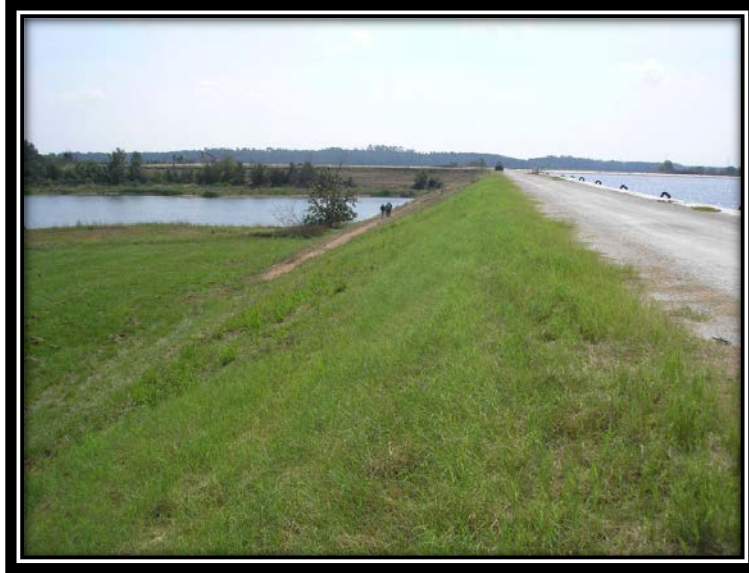
Figure 5.2.1-2 Ash Disposal Pond East cell Dike. Martin Lake is shown to the left of the dike.
