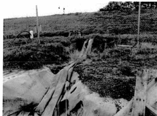
Figure 59: Erosion at Crest of Impoundment
