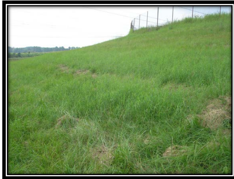
Figure 5.3.4-1 Typical groining area at PDP-4 Pond. Potential rodent burrow lower left quadrant.
