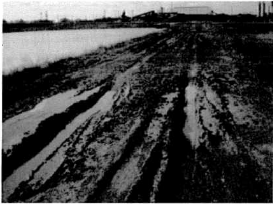
Figure 23: Crest Rutting from Vehicular Traffic
