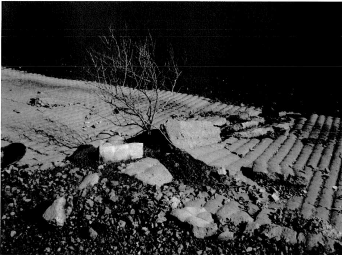
Figure 7: Revetment Damage and Plant in Liner Vent
