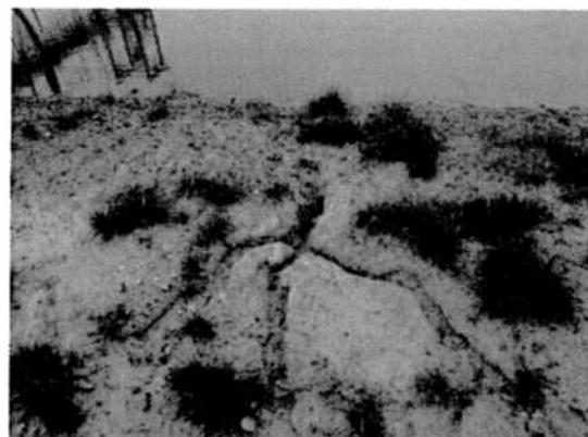
Figure 66: Moderate Erosion Rills Upstream Face
