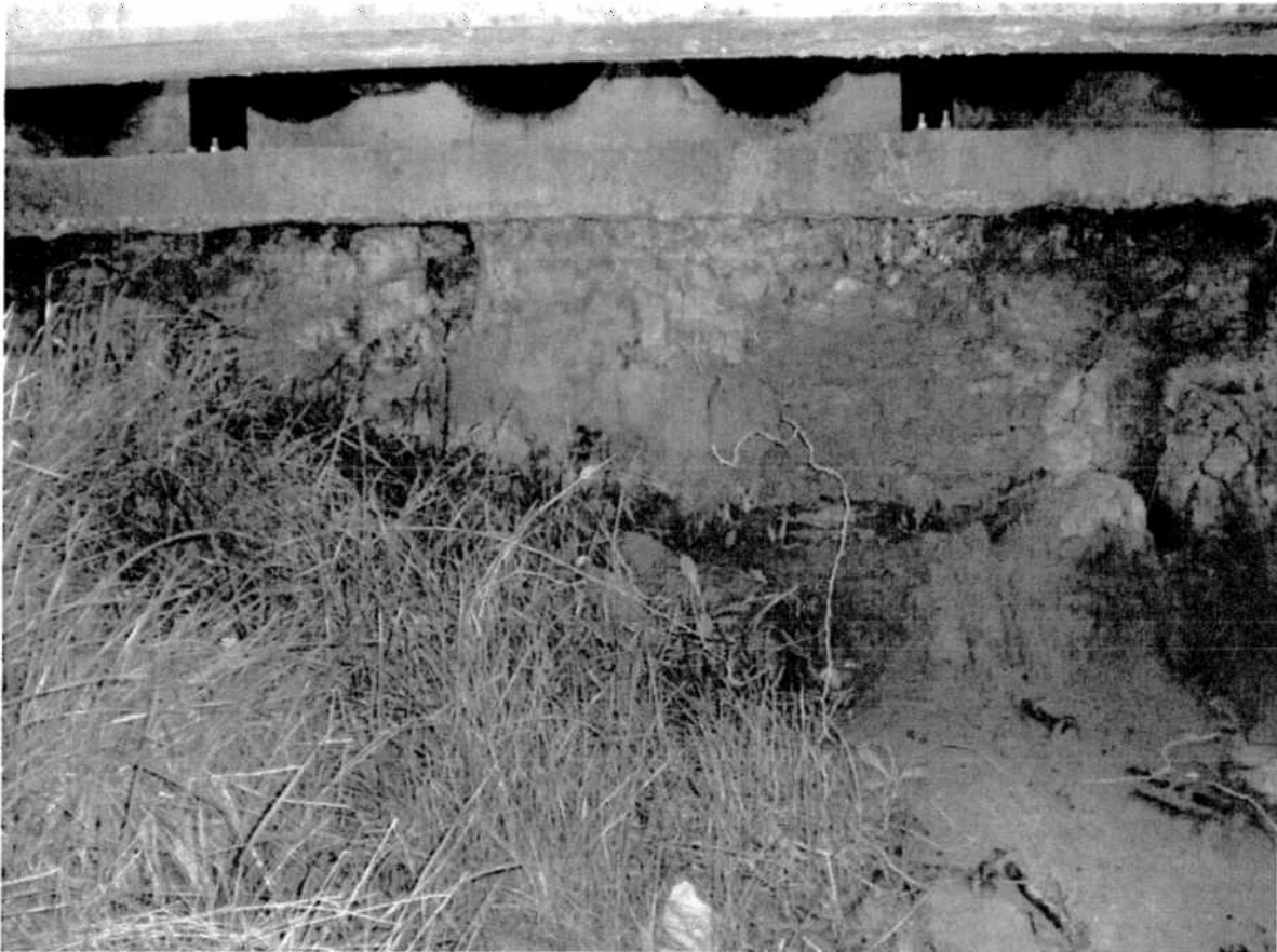
Figure 21: Erosion Under Pipe Rack
