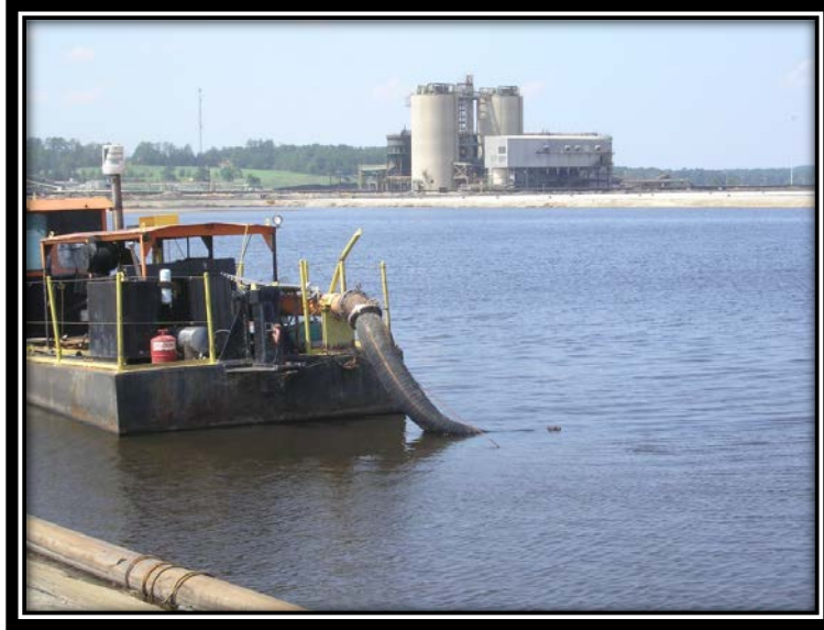
Figure 5.5.2-1 Outlet pump for Ash Disposal Pond.
