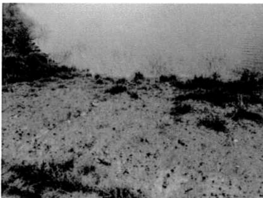
Figure 65: Minor Erosion Rills Upstream Face
