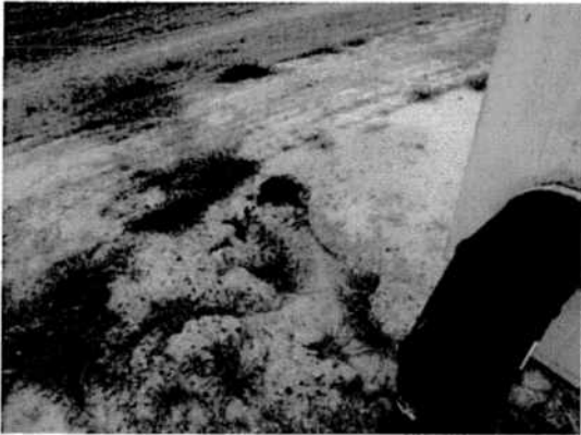
Figure 79: Erosion at Northeast Access Structure
