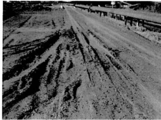
Figure 14: Rutting in Crest
