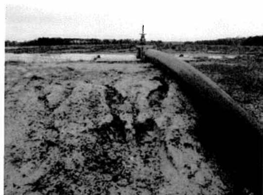
Figure 78: Erosion at Slurry Transmission Line
