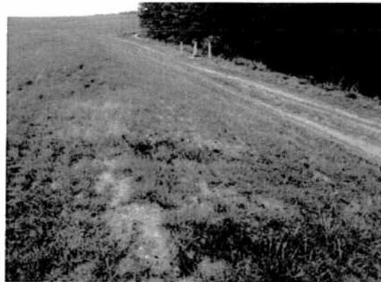
Figure 80: Erosion at PDP #3 Cap
