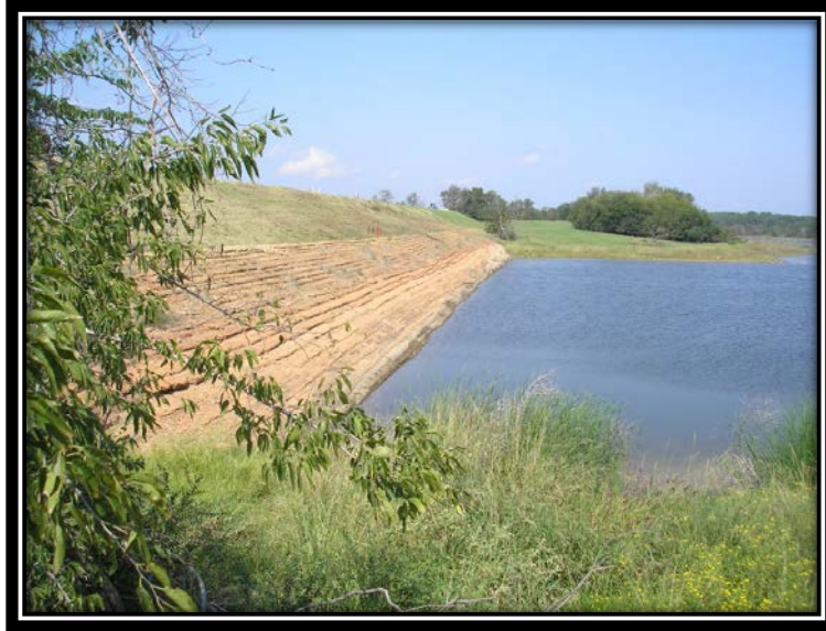
Figure 5.2.3-1 Ash Disposal Pond East cell exterior slope south end. Martin Lake right of the embankment.
