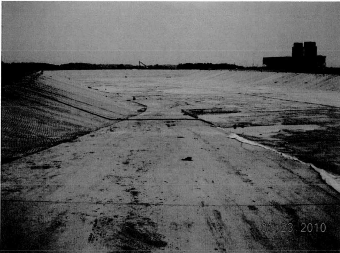
Figure 2: East Bottom Ash Pond (Note this picture was taken during construction before becoming operational and not during the inspection)
