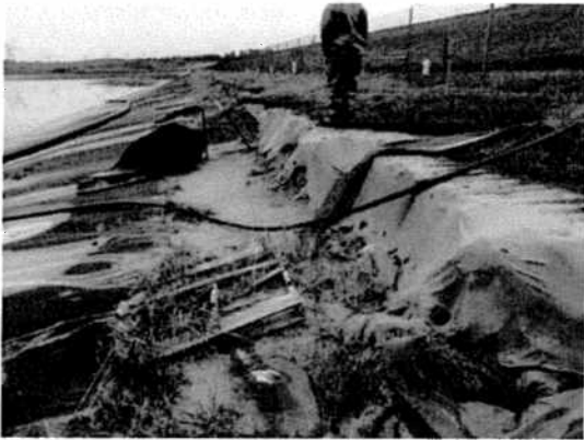
Figure 58: Erosion at Crest of Impoundment
