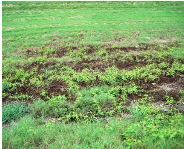
Figure 5.2.3-3. Photograph Showing Soft Wet Area at Toe of Downstream Slope of Bottom Ash Cell Embankment
