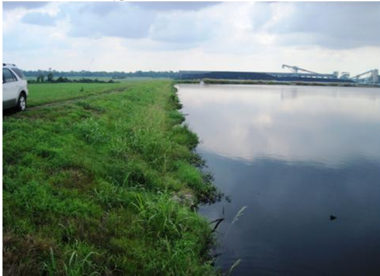
Figure 5.2.1-1. Photo Showing Crest and Upstream Slope of Fly Ash Cell Dike View to East at North Embankment
