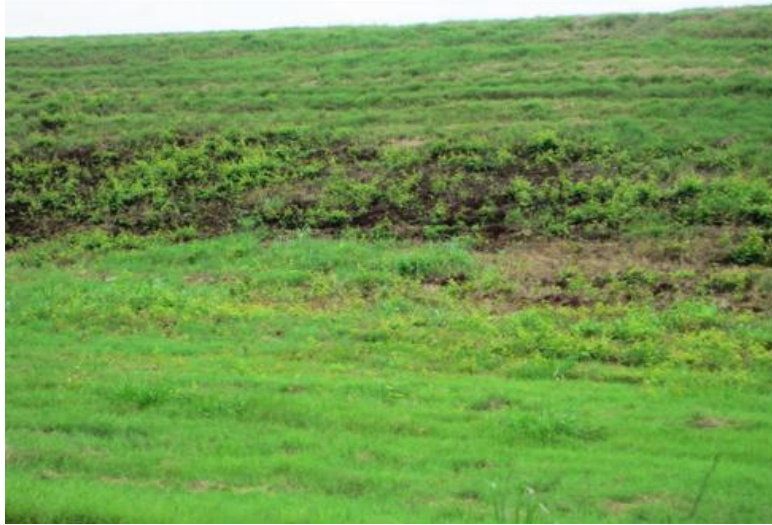
Figure 5.2.3-2. Photograph Showing Soft Wet Area and Shallow Sloughing at Toe of Downstream Slope of Bottom Ash Cell Embankment
