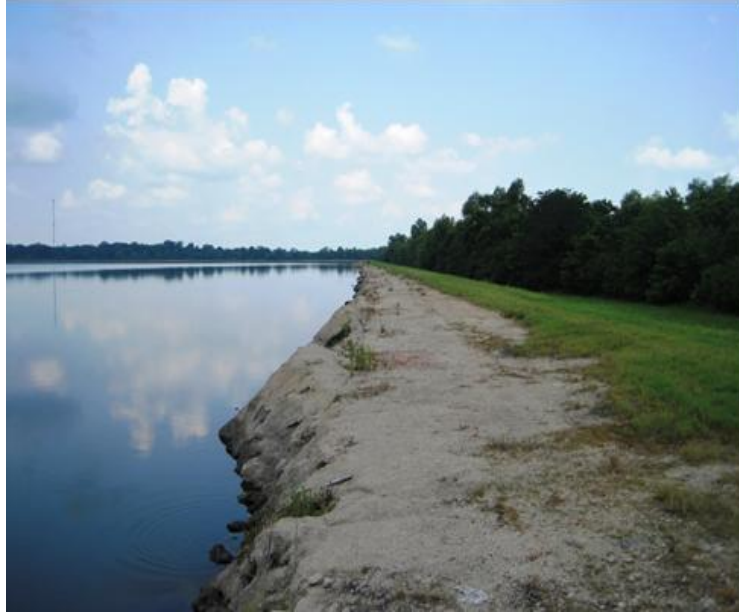
Figure 5.2.2-2. Photo Showing Long Unprotected Section of Upstream/ Inside Slope at Fly Ash Cell
