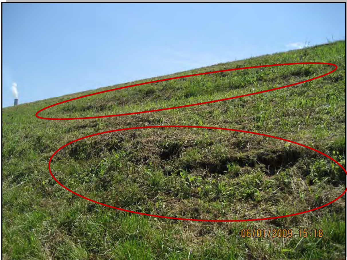
Photo 13 – Old slough on eastern downstream slope
