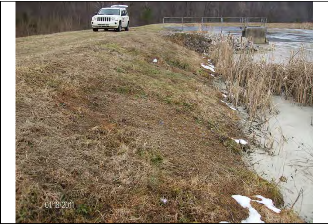
Photo #5: Interior slope, south embankment, sparse vegetation, southeast corner, looking west
