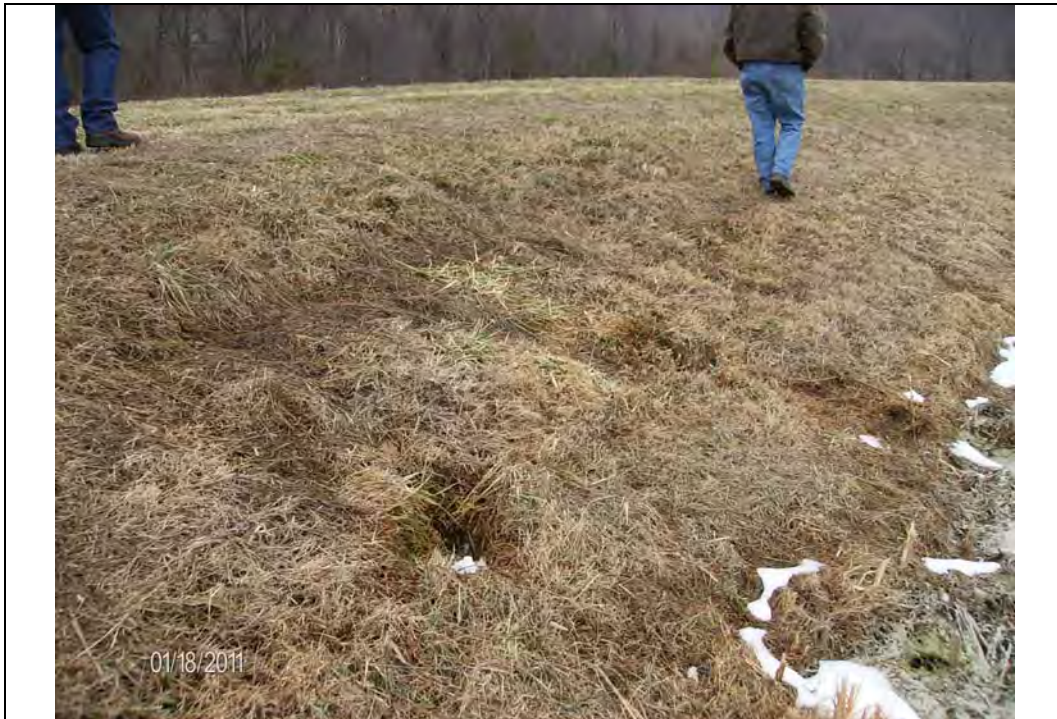
Photo #2: Interior slope, west end of south embankment, various animal burrows observed along slope, looking west
