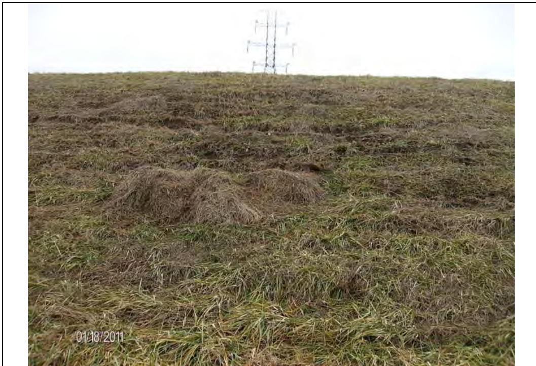
Photo #8: Exterior slope along west embankment, need to repair rutting and re-establish vegetation along slope, looking east
