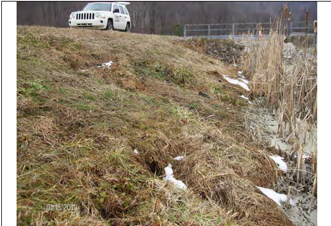
Photo #1: Interior slope, east end of south embankment, various animal burrows observed along slope, looking west
