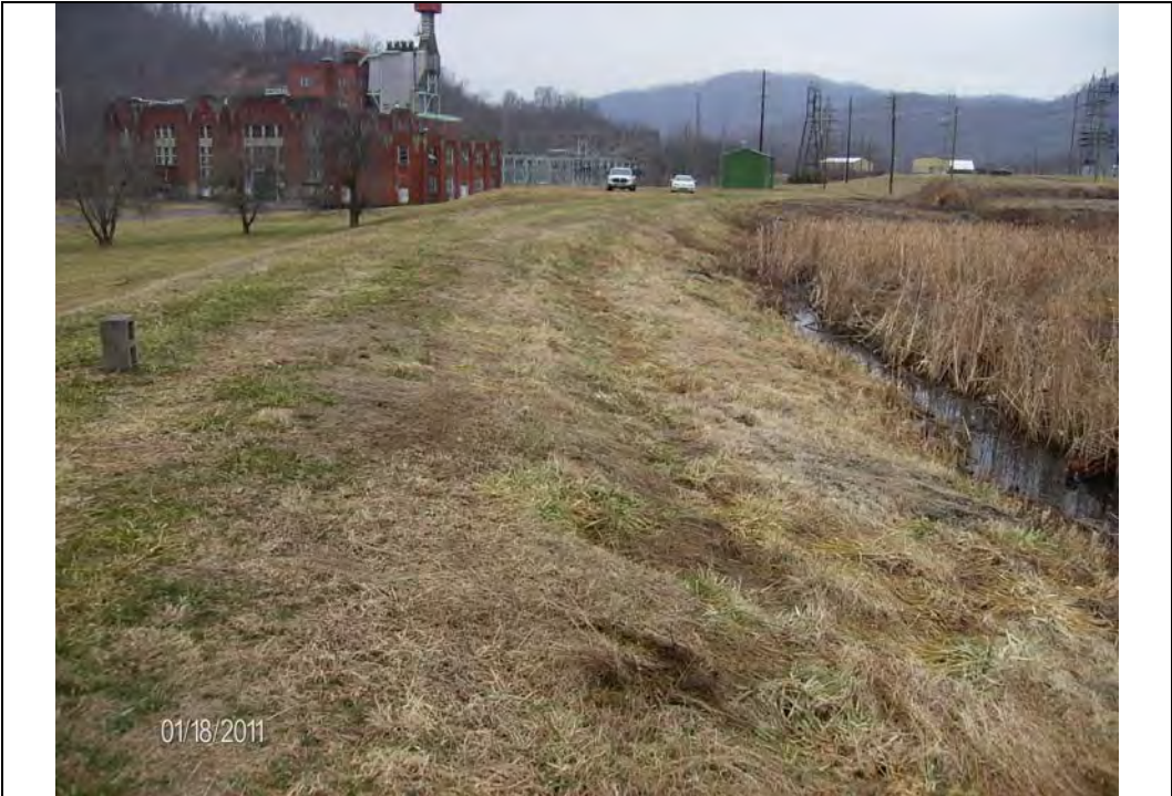
Photo #9: Crest of west embankment, fill low area at upstream side to restore to nominal width, looking north
