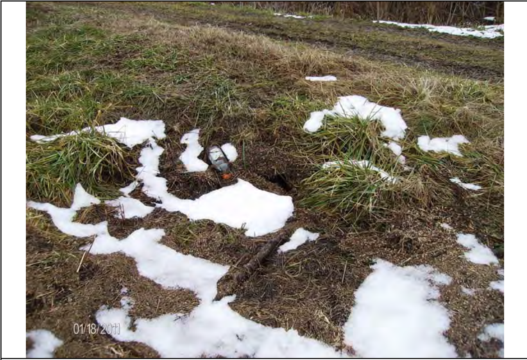
Photo #6: Exterior slope, partially blocked culvert draining ditch below toe at SW corner, looking southeast
