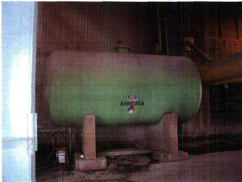
Photograph 006, Ryan Kivett. March 5, 2009. Chemicals are stored inside the generating plant. Utilicorp has spill emergency plan with trained personnel. The plant floor drains terminate into the storage lagoon at the outfall 006. Utilicorp is careful to monitor all agents and chemicals stored within the building to keep them from spilling or tracking into the environment. Utilicorp captures all agents before discharging from outfall 006.
