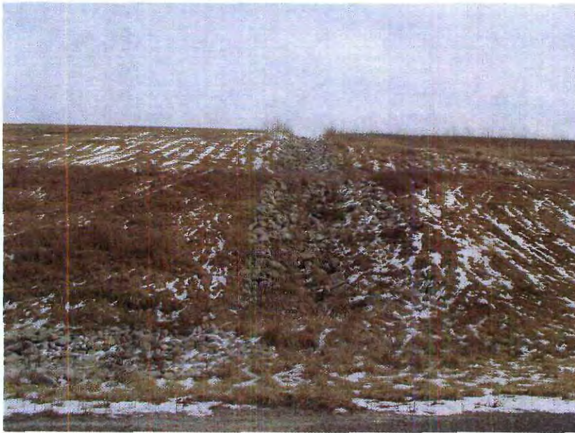
Photograph 005, Ryan Kivett. March 5, 2009. Closed fly ash landfill. Leachate is discharged to the fly ash storage pond. This landfill is well maintained.
