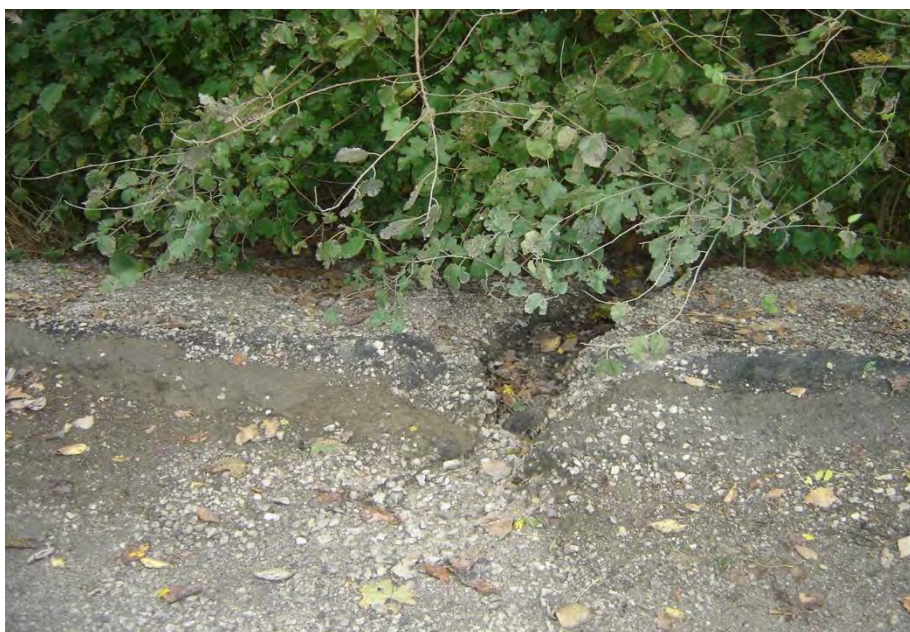
Figure 5.4.3-2. Outside Slope of North Dike Erosion.
