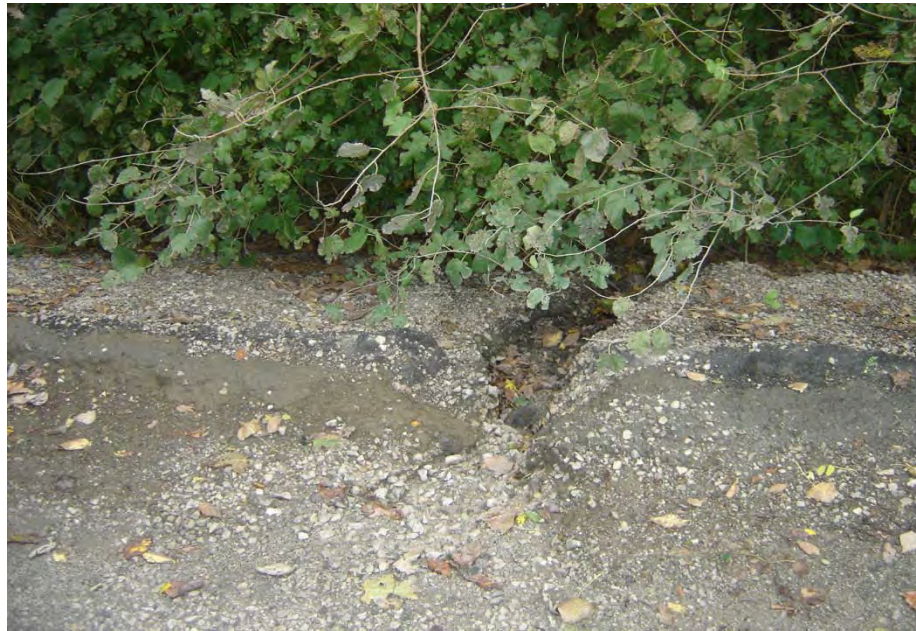
Figure 5.4.3-2. Outside Slope of North Dike Erosion.
