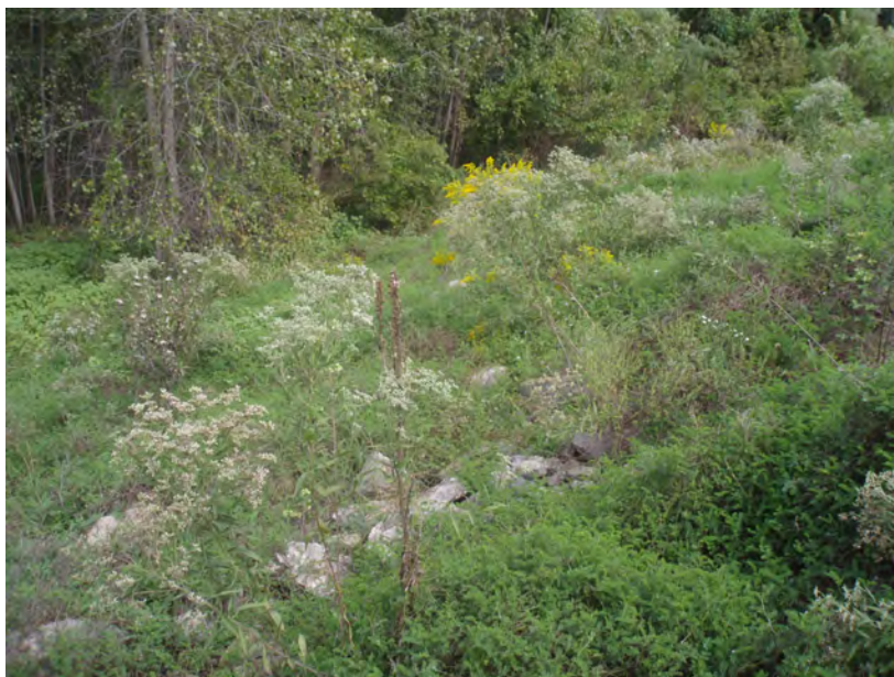
13. Exterior of dike – Taken from north side of pond looking northeast down side of dike. Heavy vegetation at base and on dike.
