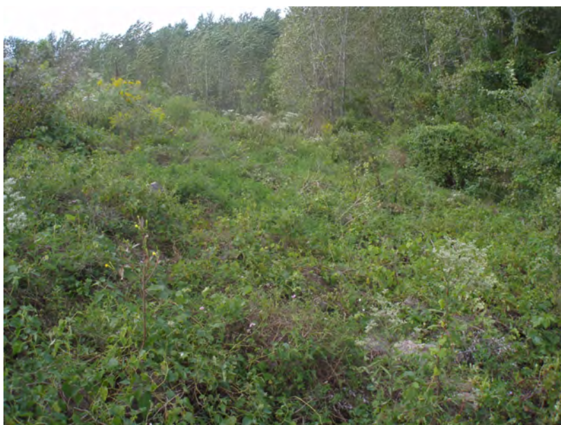
10. Exterior of dike – Taken from east end of pond looking north. Heavy vegetation at base and on dike.
