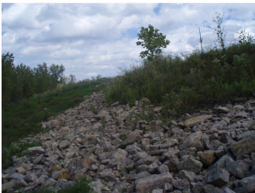
20. Exterior of dike – Taken from north side of pond looking east. Heavy vegetation at base and on dike.
