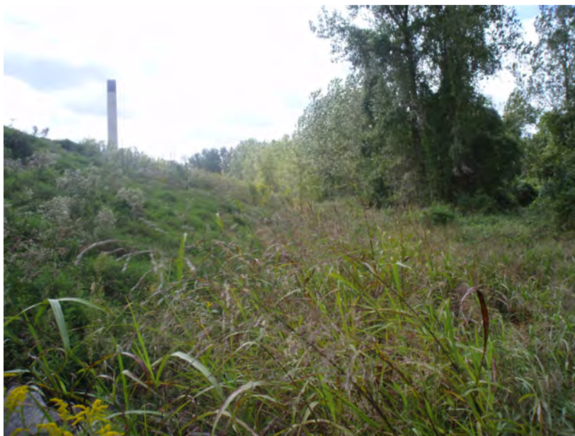
16. Exterior of dike – Taken from north side of pond looking southwest/west. Heavy vegetation at base and on dike.
