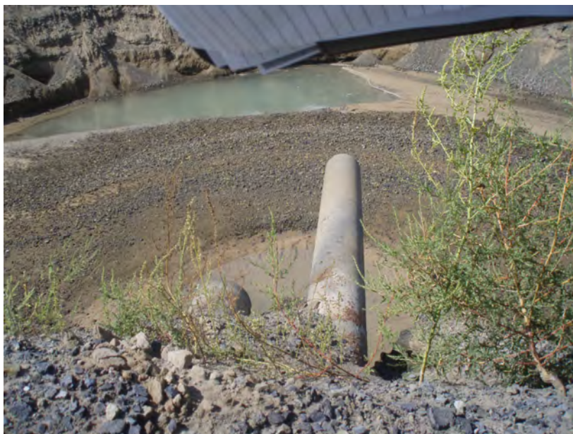
31. Discharge from plant on south side of ash pond, taken from interior berm between ash pond and clear water pond.
