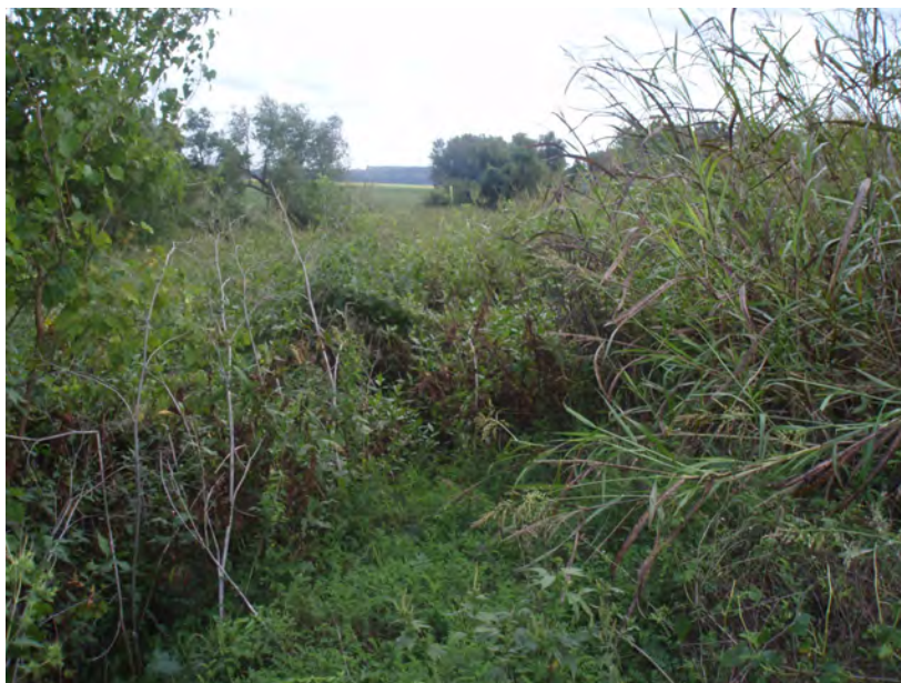
9. Exterior of dike – Taken from east end of pond looking south. Heavy vegetation at base and on dike.
