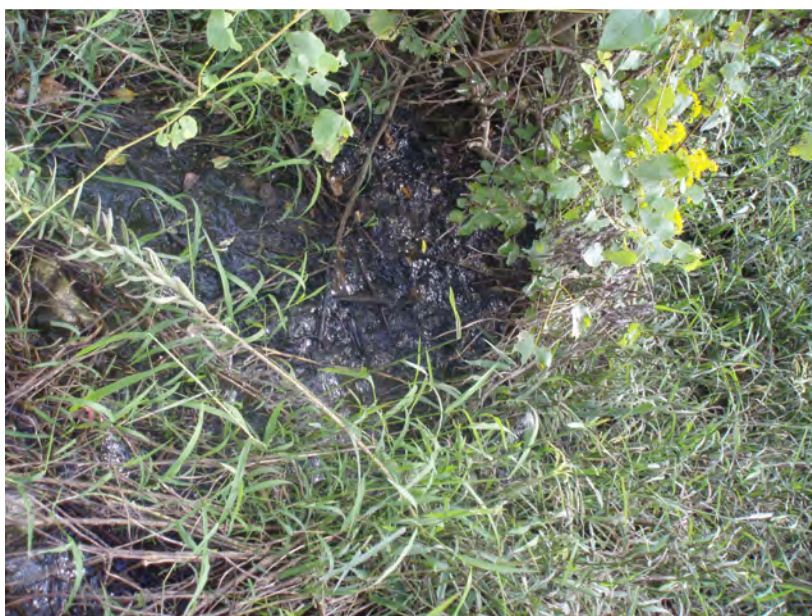
4. Outfall pipe – small amount of discharge observed
