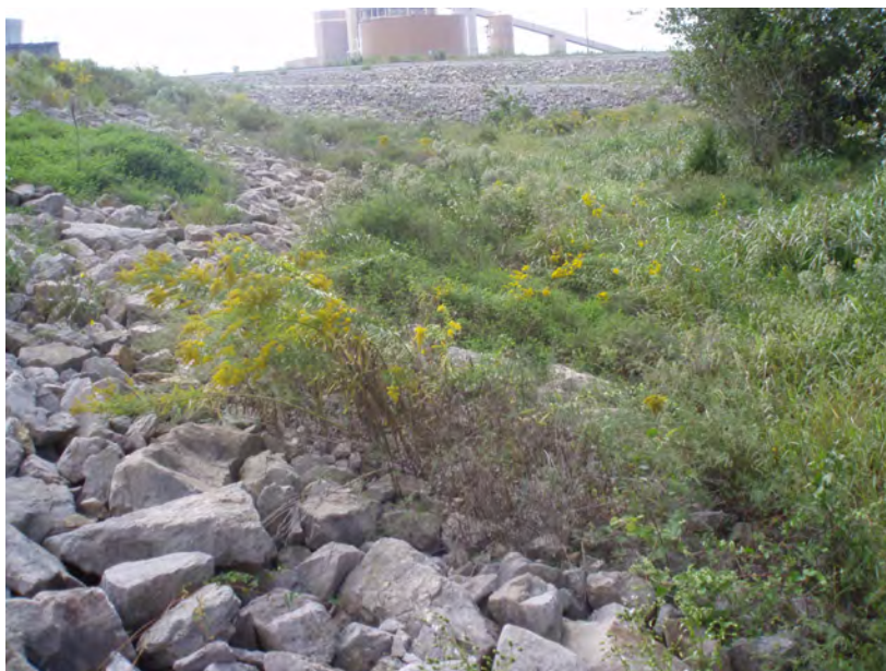
19. Exterior of dike – Taken from north side of pond looking west. Heavy vegetation at base and on dike.
