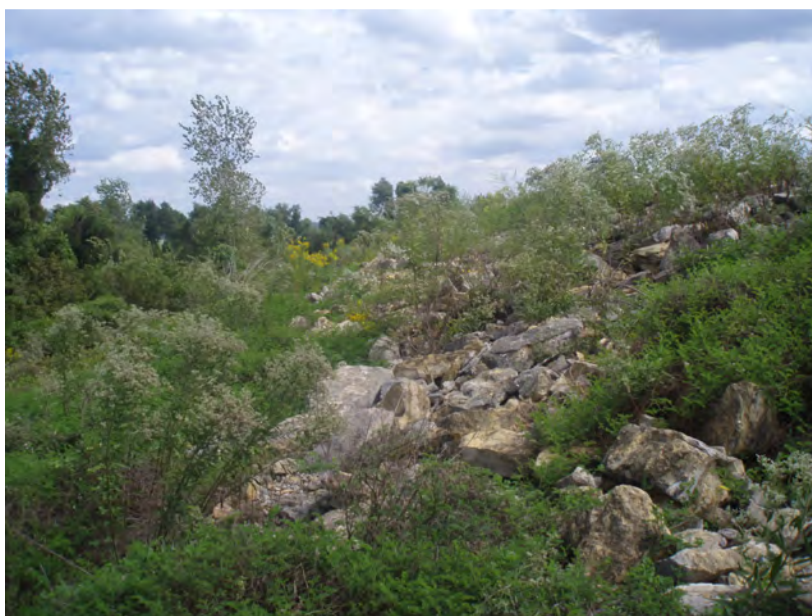
12. Exterior of dike – Taken from north side of pond looking east. Heavy vegetation at base and on dike.
