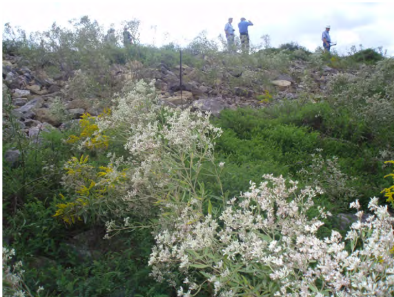
14. Exterior of dike – Taken from north side of pond looking southwest up side of dike. Heavy vegetation at base and on dike.
