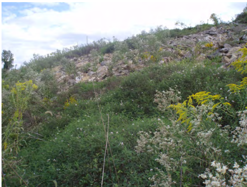
15. Exterior of dike – Taken from north side of pond looking southeast up side of dike. Heavy vegetation at base and on dike.
