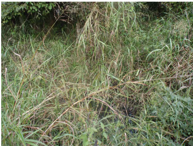
5. Standing water at foot of dike below outfall pipe
