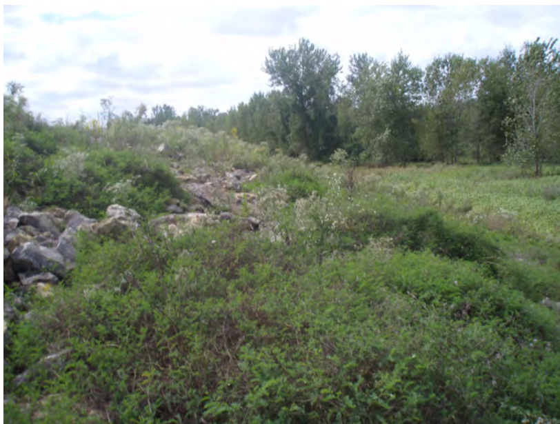
11. Exterior of dike – Taken from north side of pond looking west. Heavy vegetation at base and on dike.
