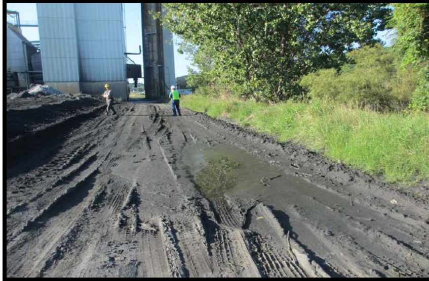
Photo 5.3.3g: Ponded water along west toe of West Pond
