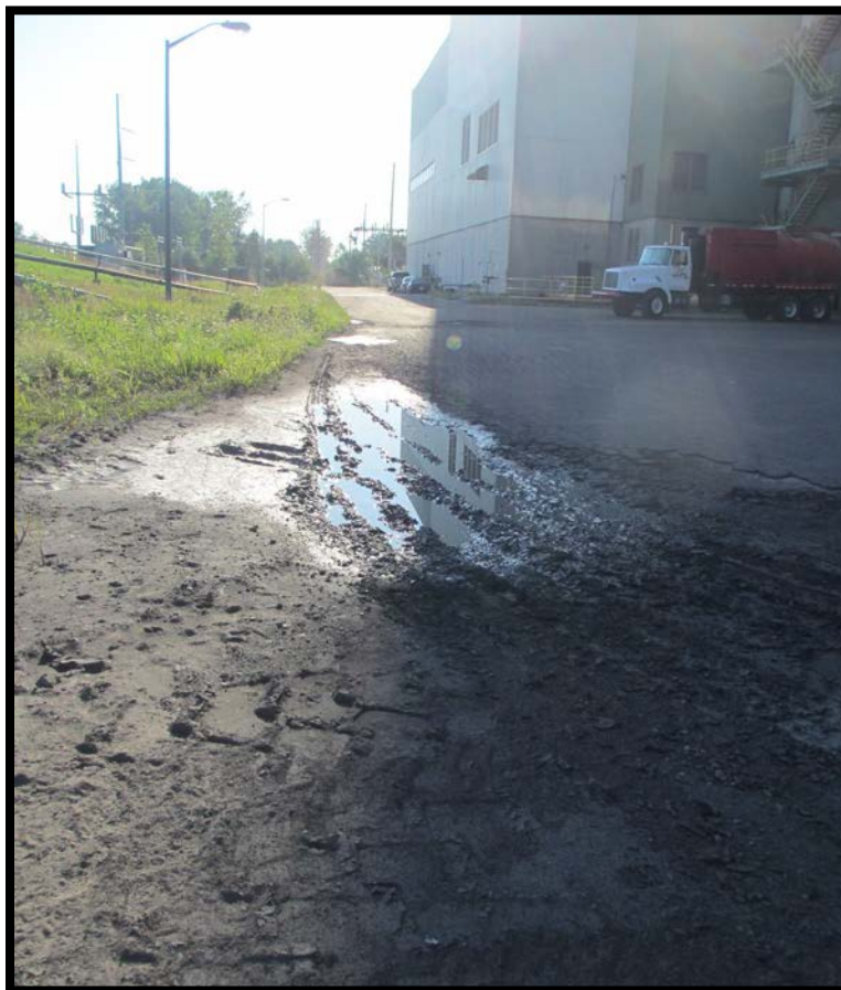
Photo 5.3.3j: Looking east from West Pond's southwest toe at presence of ponded water along Ponds' south toe
