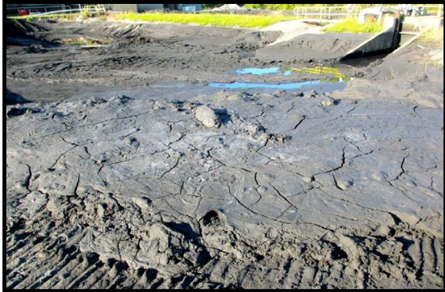
Photo 5.2.2: Inside slope of East Pond at the northeast corner (Note disturbance of clay liner at top of photo.)
