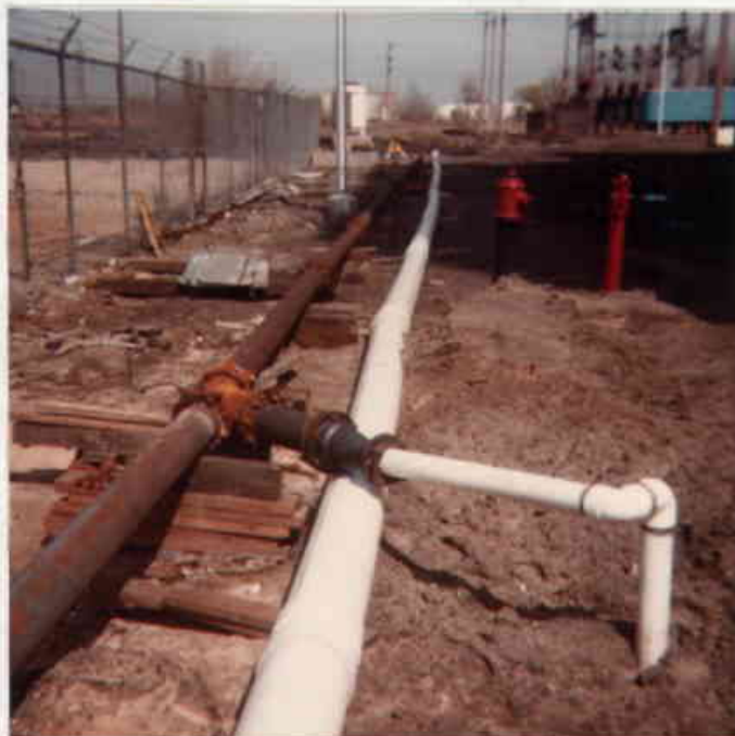
3. Temporary piping leading to Units 1 & 2 ash pond.
