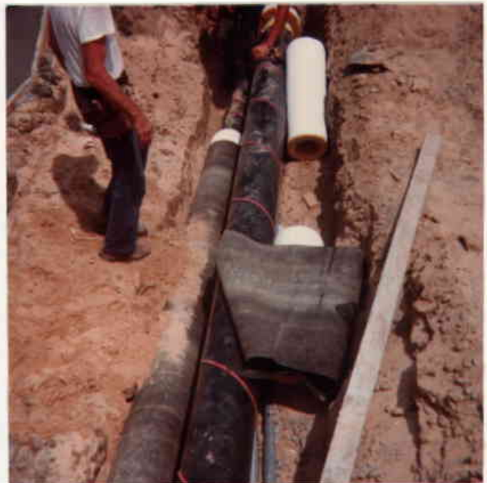
78. Heat tracing and insulating the piping through the center dike at the location of the overflow wier.
