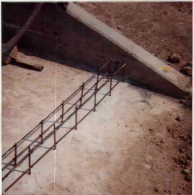
54. Re-steel set in place for the stop log wall at the west end of the structure.
