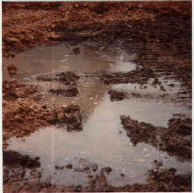
13. Close proximity of the ground water table to the bottom of the clay lining.
