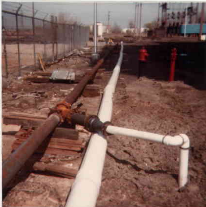
3. Temporary piping leading to Units 1 & 2 ash pond.
