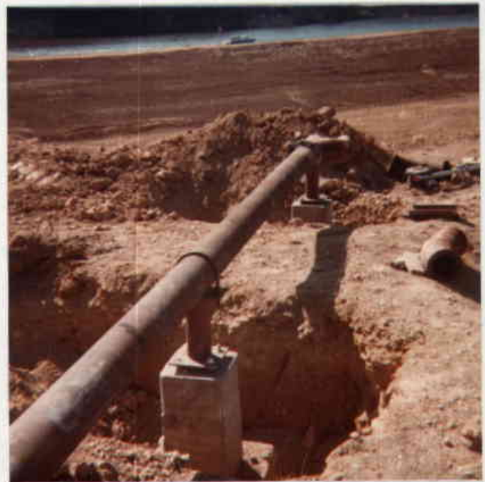
70. Bottom ash line installation at the south end of the center dike.
