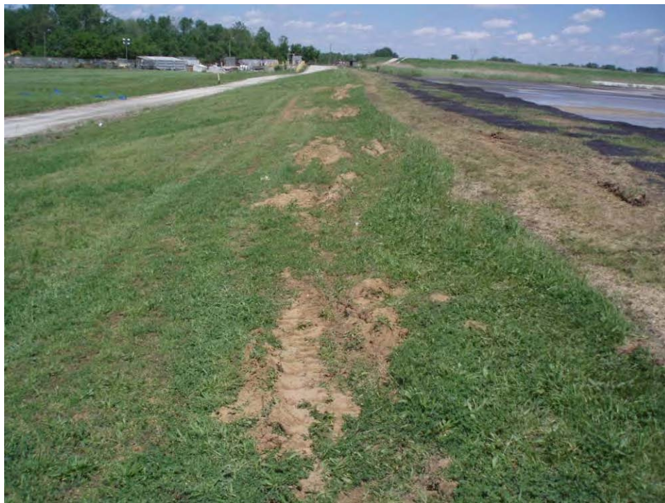
23. Pond A - West embankment exterior slope, looking north at tractor ruts.
