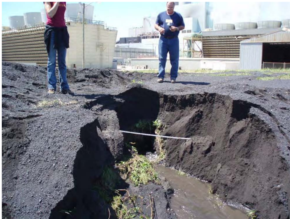
15. Pond A - Active erosion/piping of south embankment interior slope from unknown water source. Water was clear. Eroded area 5'Wx8'Lx3.5'D. IPL personnel were trying to determine source of flow.
