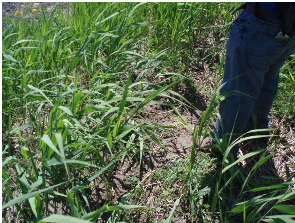
61. Pond B - South embankment exterior slope looking at bare spots of very soft, fine grained stabilized FGD.
