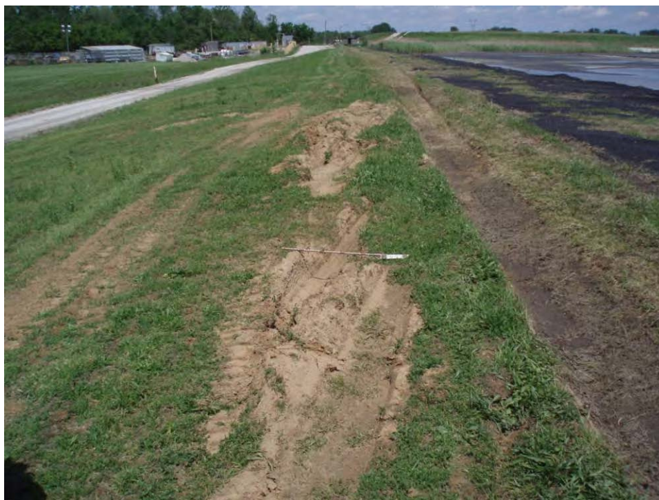
26. Pond A - West embankment exterior slope, looking north at large tractor ruts and excavator tracks.
