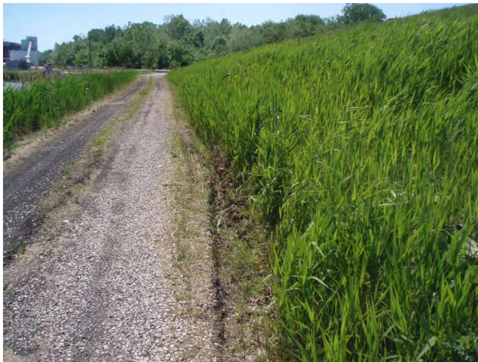
63. Pond B - South embankment exterior slope, looking southwest at possible seepage at toe.
