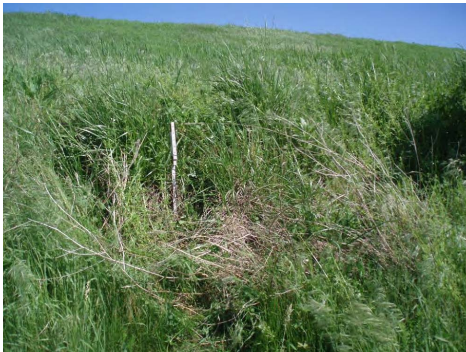
85. Pond B - West embankment lower exterior slope, looking at over-steep area and surficial erosion at bench.
