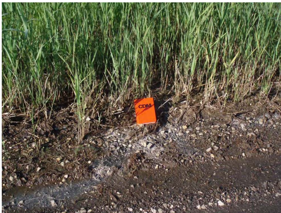
122. Pond C - North embankment bench, looking at active seepage located at toe of upper exterior slope. Note the white sheen in the water.
