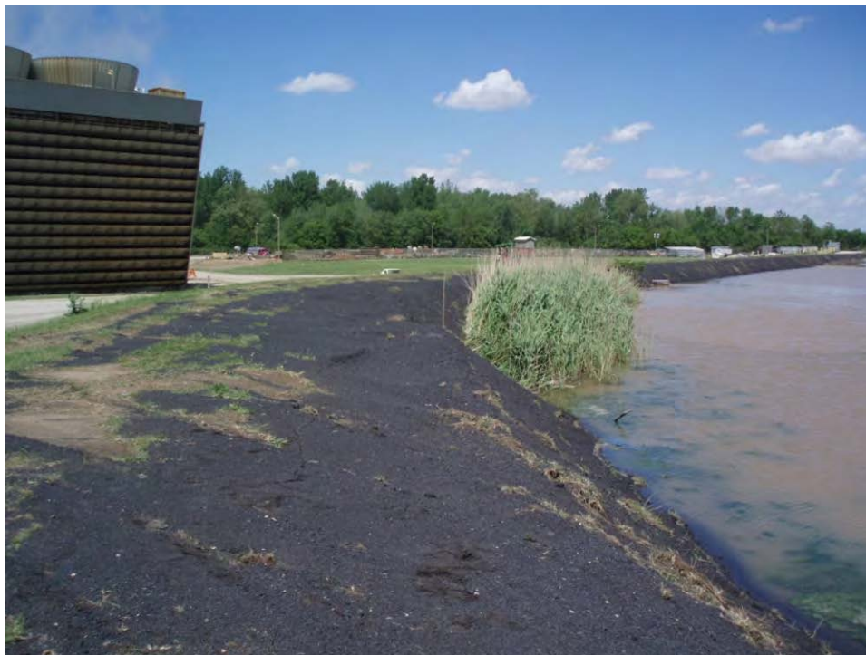
17. Pond A - South embankment crest, looking northwest at recently placed ash. Note existing embankment was not cleared or grubbed before placing material.
