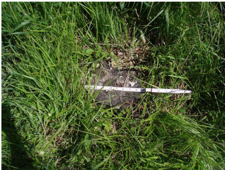
80. Pond B - West embankment lower exterior slope, looking at 0.9-foot-diameter tree stump at toe.
