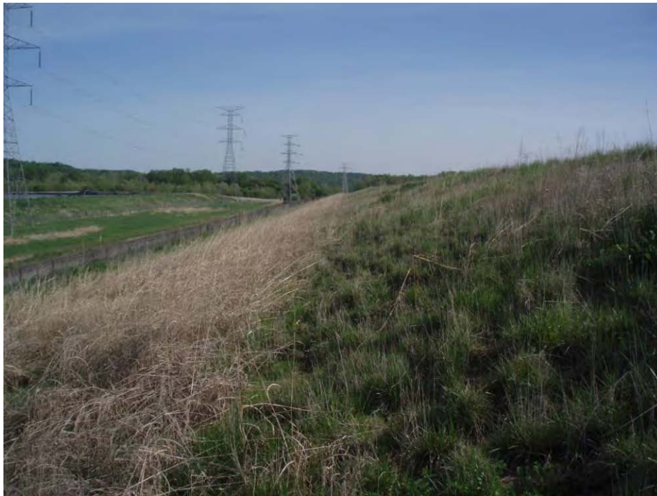
89. Pond D - West embankment exterior slope, looking north. Note bands of vegetation from the vertical expansions. Bare spots observed on upper third.
