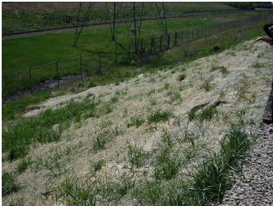
3. Pond A - East embankment exterior slope. Erosion control blanket installed near northeast corner looking southeast. Note: Blanket appears to be improperly staked, there are 1- to 3-inch gaps beneath the blanket, and there is no apparent anchor trench or roll overlap.
