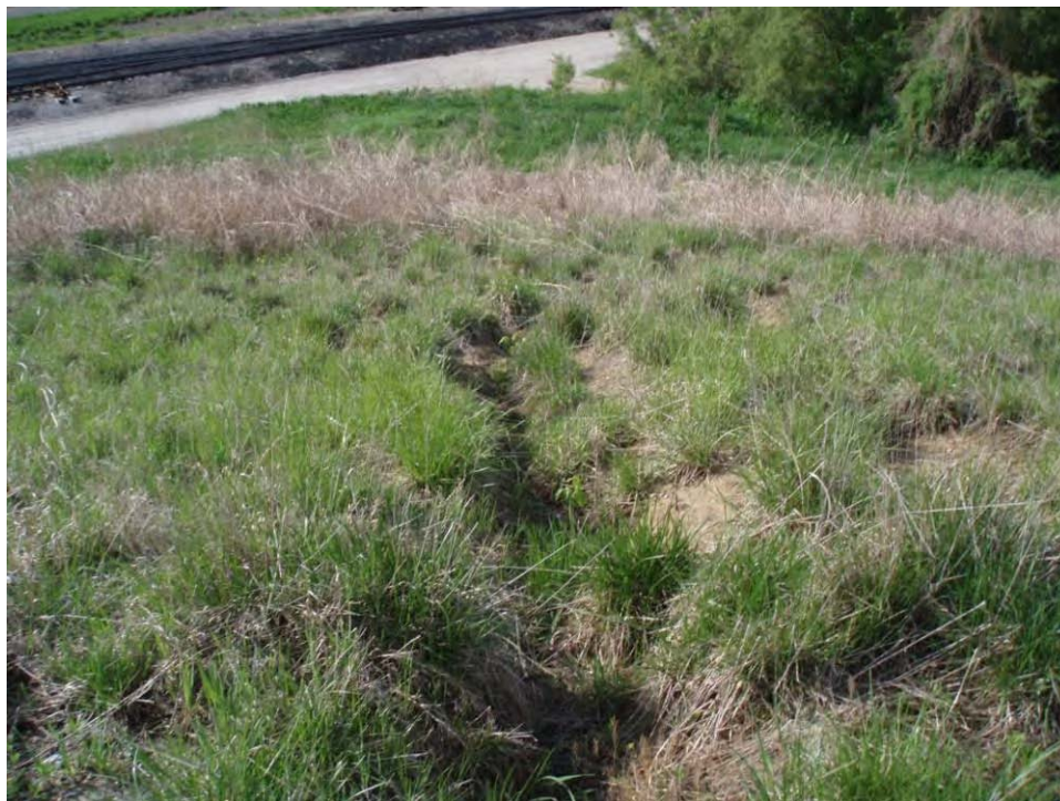
85. Pond D - Erosion rill on southeast embankment exterior slope, looking southeast.
