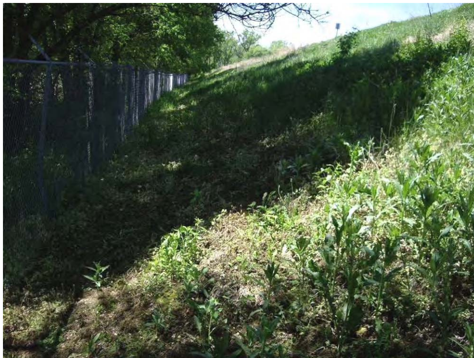
21. Pond A - Soft spongy area at toe of south embankment under tree canopy (possible former active seepage area).
