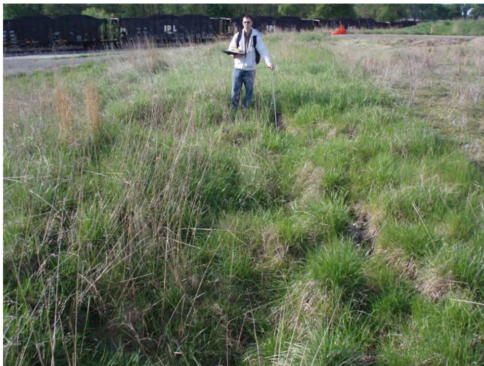
72. Pond D - Erosion rill and depression on east embankment buttress berm, looking south.
