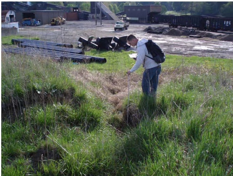
73. Pond D - Erosion rill on east embankment buttress berm, looking northeast
