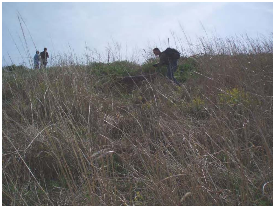
107. Pond E - 8'Wx4.5'Dx15'L erosion gulley at crest of west embankment exterior slope from previous failure event. Note erosion is scheduled to be repaired.
