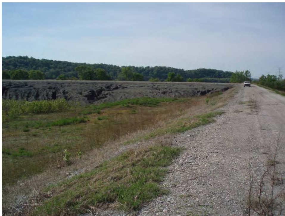
92. Pond D - West embankment interior slope, looking south at edge of ash limit prior to Pond D/E embankment failure.
