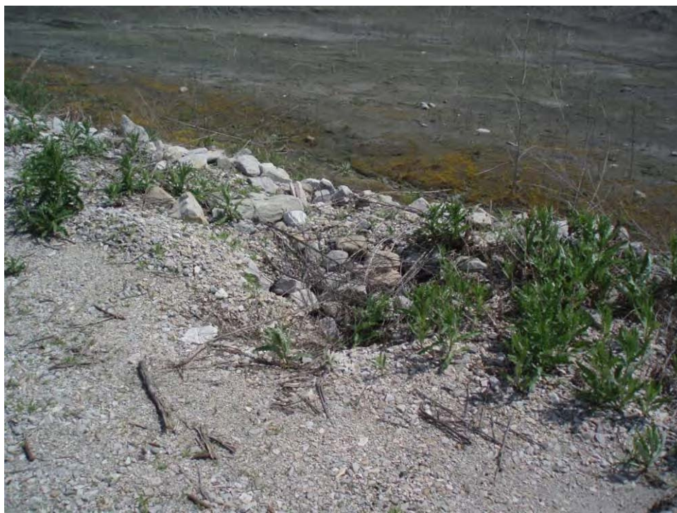
130. Pond D - Depression with piping on east slope of divider embankment, looking northeast.
