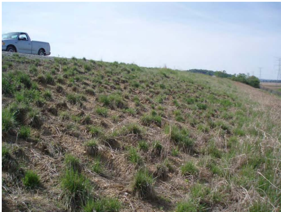
97. Pond D - Typical bare spot and erosion on west embankment exterior slope, looking southeast.
