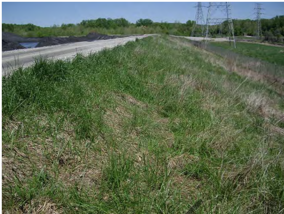
7. Pond A - depression near crest of east embankment, looking north.
