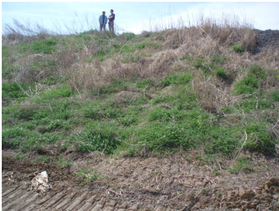
119. Pond E - erosion feature on north embankment exterior slope from previous failure event.
