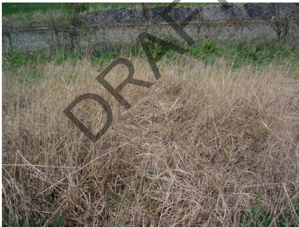
112. Pond E - 8'Wx3'Dx25'L erosion gulley at mid-slope of west embankment exterior slope from previous failure event. Note erosion is scheduled to be repaired.
