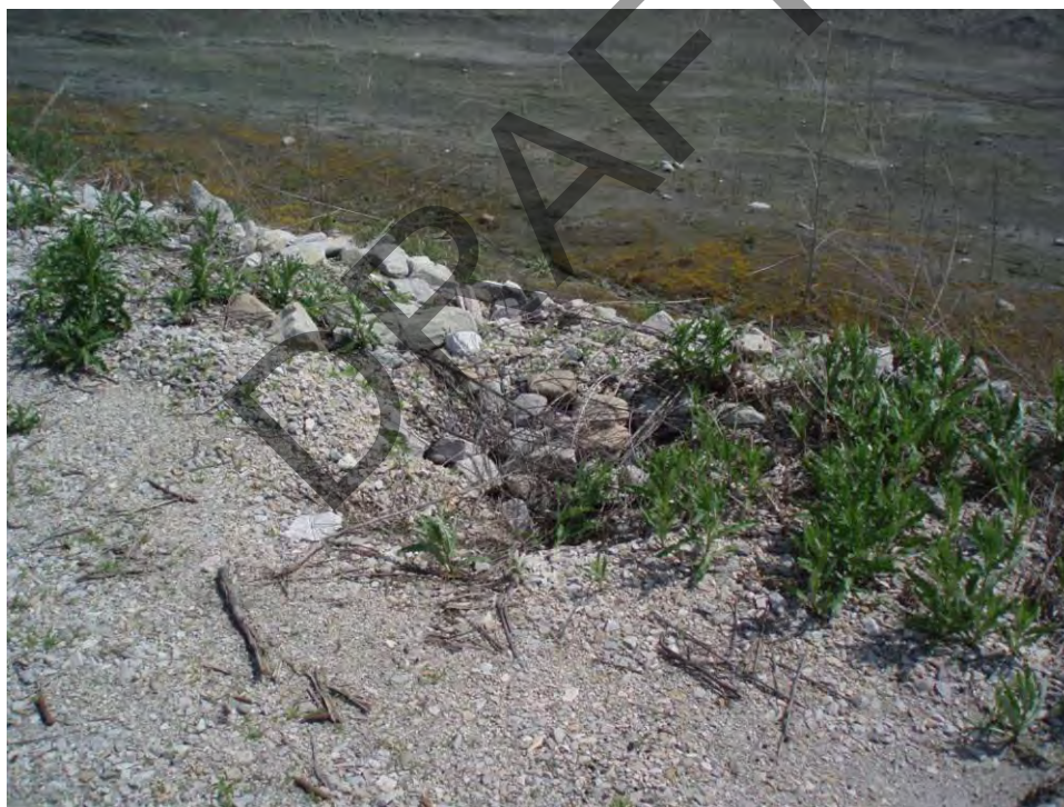
130. Pond D - Depression with piping on east slope of diversion embankment, looking northeast.
