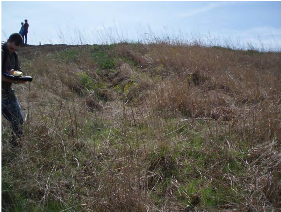
113. Pond E - two approximately 4'Wx3'Dx20'L erosion gulleys at mid-slope of west embankment exterior slope from previous failure event. Note erosion is scheduled to be repaired.
