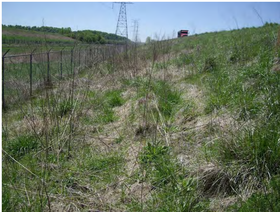
5. Pond A - East exterior slope looking south. Low spot and minor slough at toe of slope.. Possible tractor rutting.
