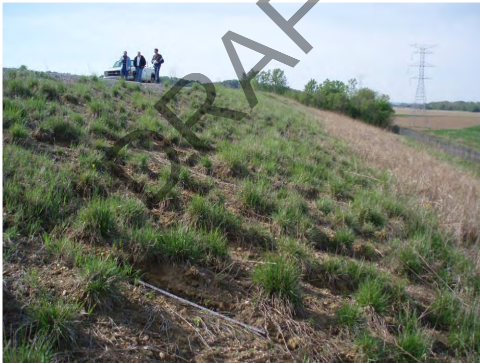
90. Pond D - Typical bare spots on upper third of west embankment exterior slope, looking south.
