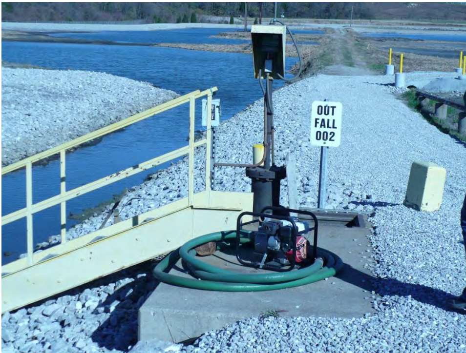
Photo 12: Outfall 002 and associated channel which is the outlet from the Bottom Ash Pond into the sanitary sewer system.
