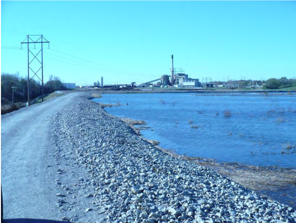
Photo 1: Looking south along the east dike of the North Fly Ash Pond.
