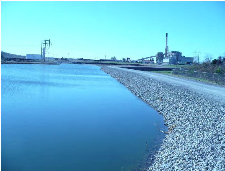
Photo 10: Looking south at the Bottom Ash Pond west dike. Taken from the northwest corner of the Bottom Ash Pond.
