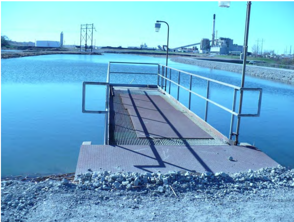
Photo 6: The Bottom Ash Intake Structure at the north end of the Bottom Ash Pond.
