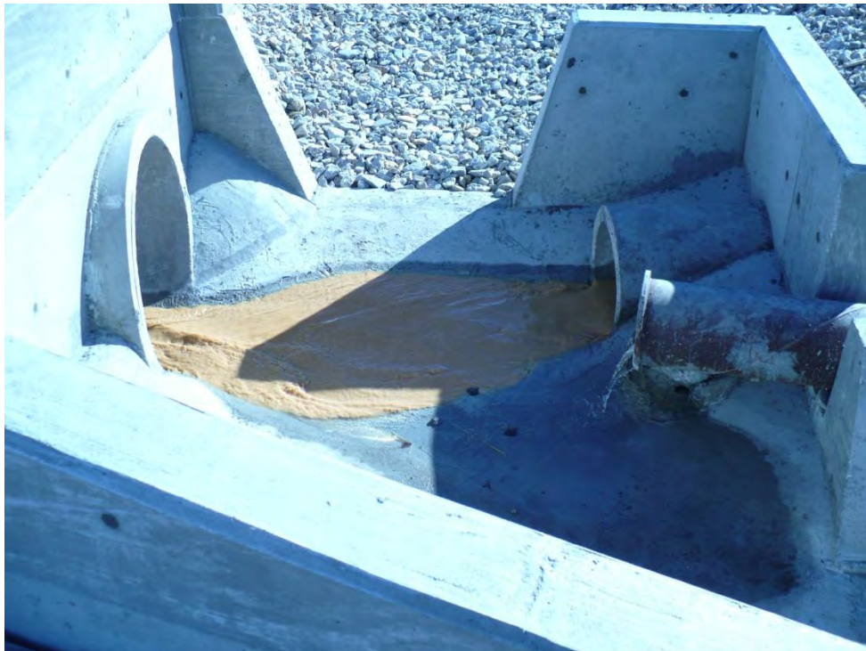
Photo 14: Inlet pipe to the Bottom Ash Pond.
