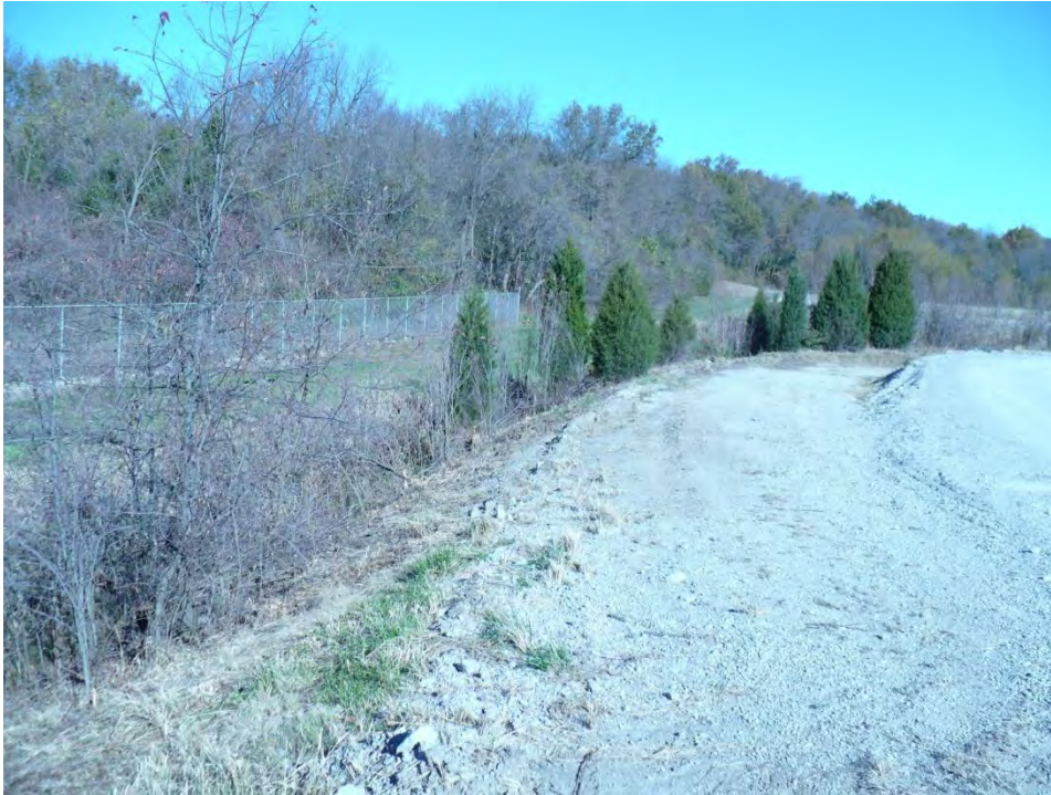
Photo 9: Trees on slope of pump house access road slope at the northwest corner of the Bottom Ash Pond
