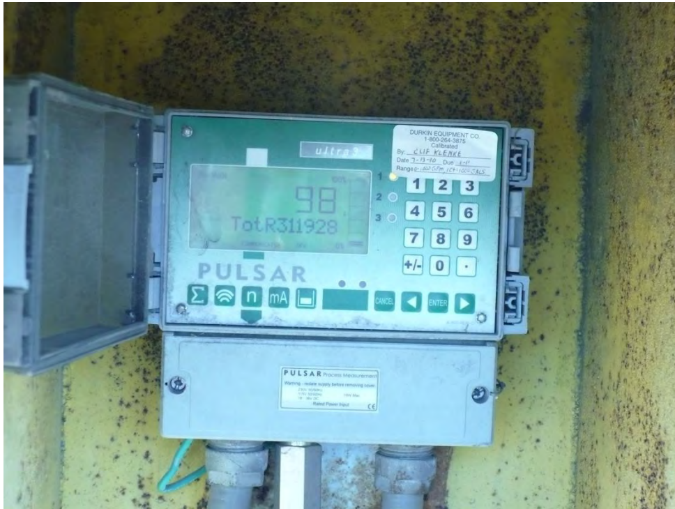
Photo 13: The flowmeter to monitor the discharge from the Bottom Ash Pond into the sanitary sewer system.
