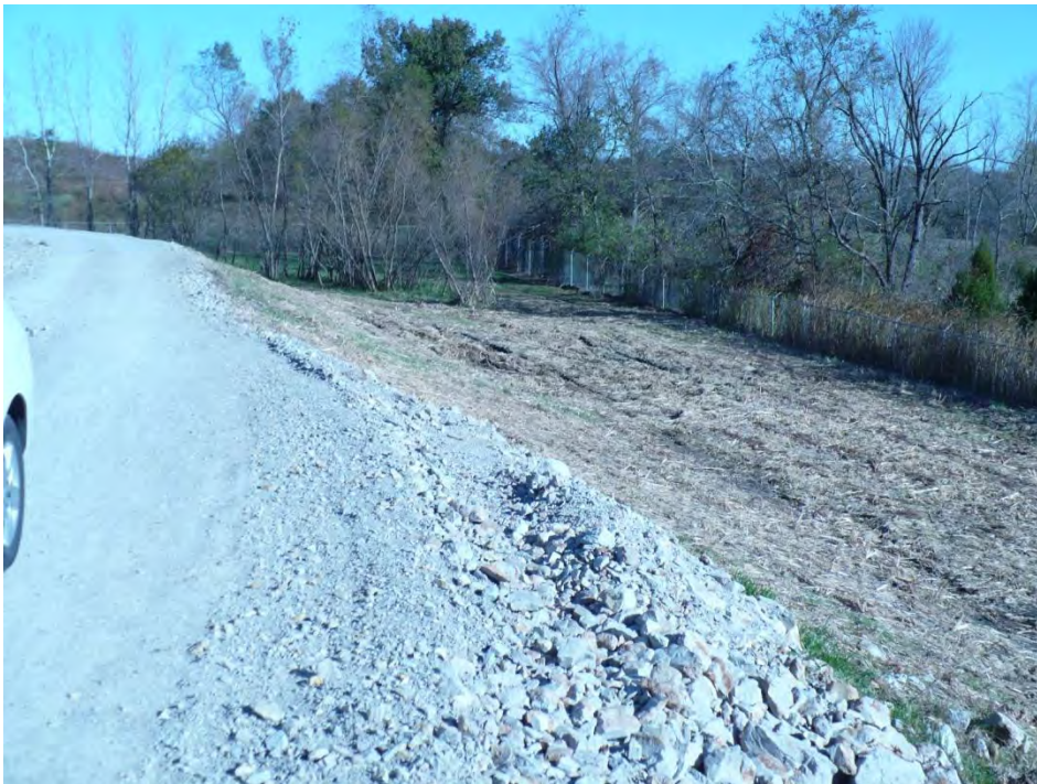
Photo 2: The north east corner of the North Fly Ash Pond dike. Note possible seepage occurring at dike toe.
