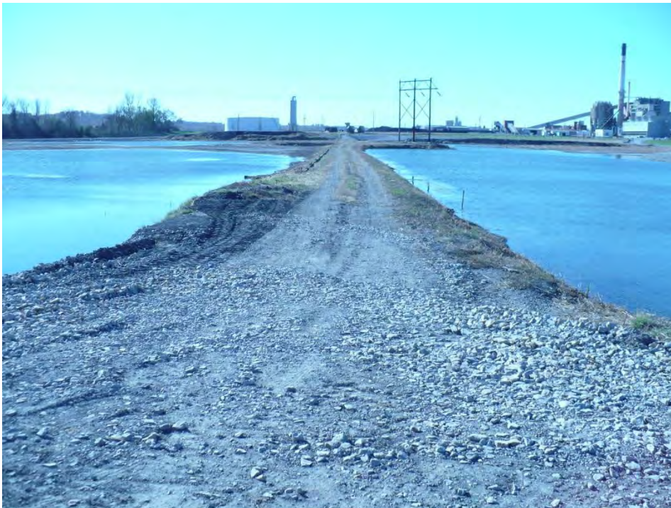
Photo 8: Looking south at the dike that separates the Bottom Ash Pond (right) from the South Fly Ash Pond (left).
