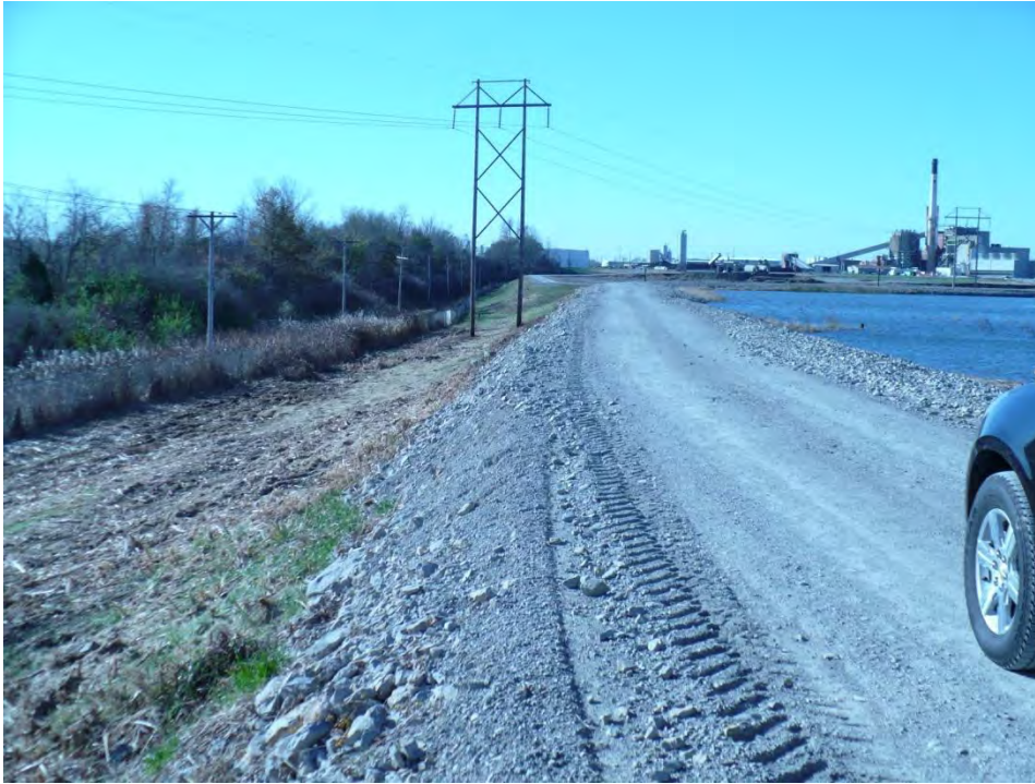
Photo 3: Looking south along the east dike of the North Fly Ash Pond. Note possible seepage occurring at the dike toe.
