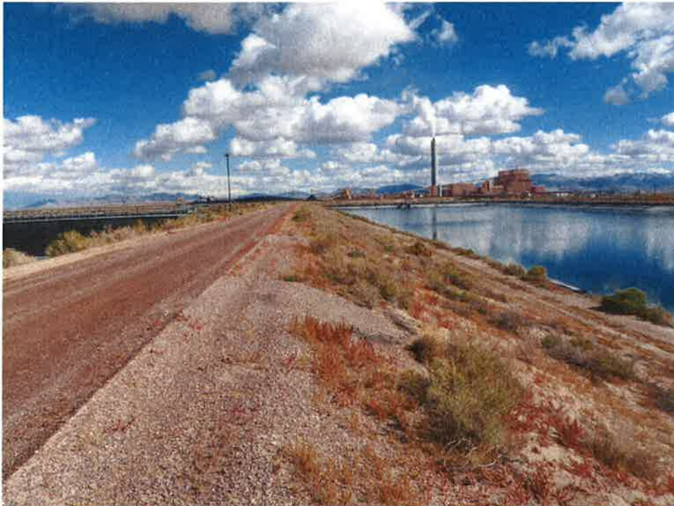
Photo 24: Bottom Ash Basin #1-3, looking east at south dike crest and downstream slope.
