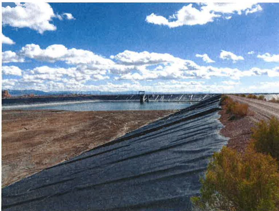
Photo 33: Bottom Ash Basin #1, looking south at intake and inner dike upstream slope and liner.
