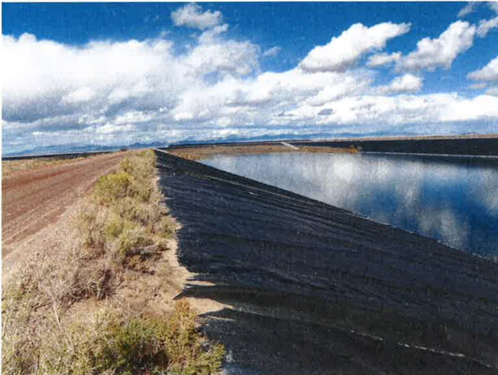
Photo 20: Bottom Ash Basin #3, looking north at west dike crest, upstream slope and liner.
