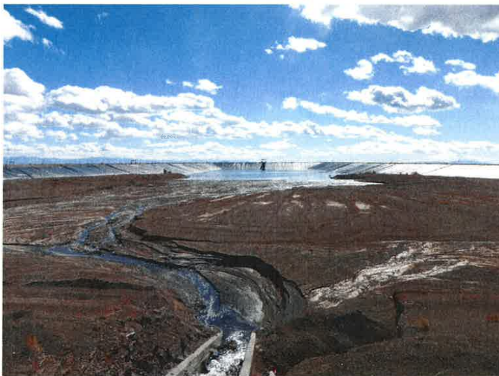
Photo 32: Bottom Ash Basin #3, looking south from north bank at inlet area and reservoir slopes.
