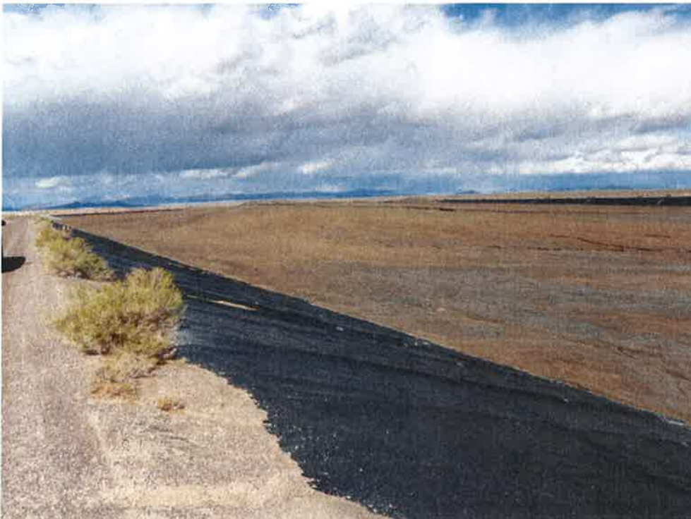
Photo 36: Bottom Ash Basin #1, looking northeast from inner dike at inlet and reservoir area.
