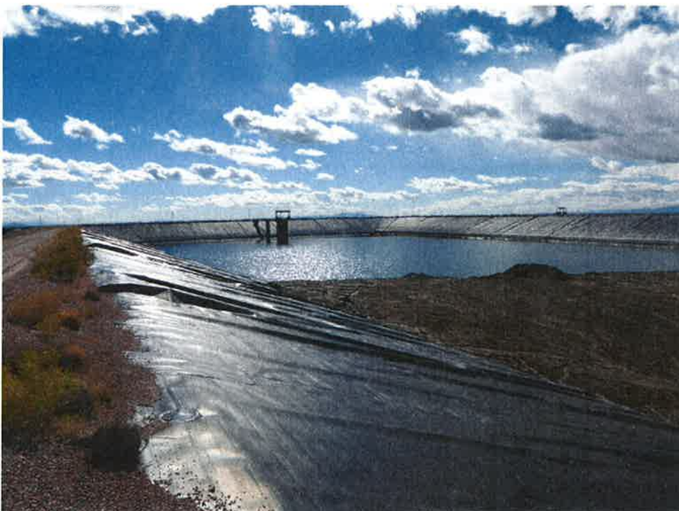
Photo 34: Bottom Ash Basin #2, looking south at intake and inner dike upstream slope and liner.
