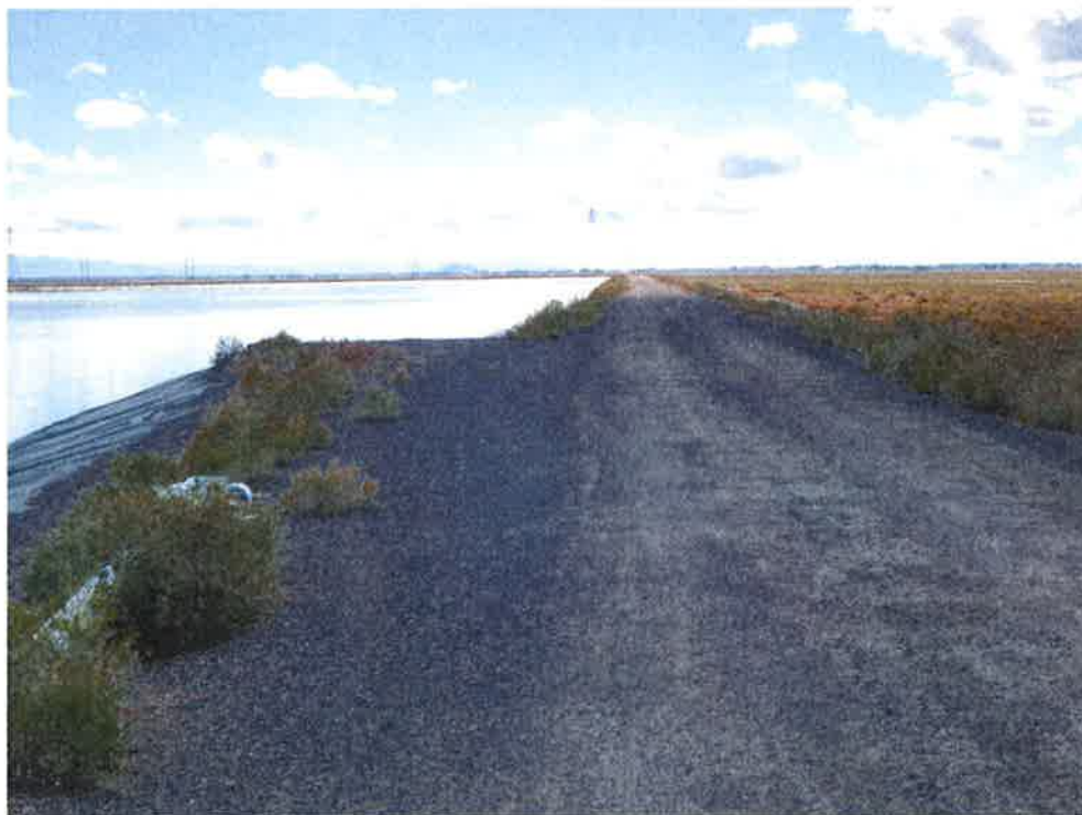
Photo 11: Wastewater Holding Pond, looking south from west dike at crest and entrance ramp.
