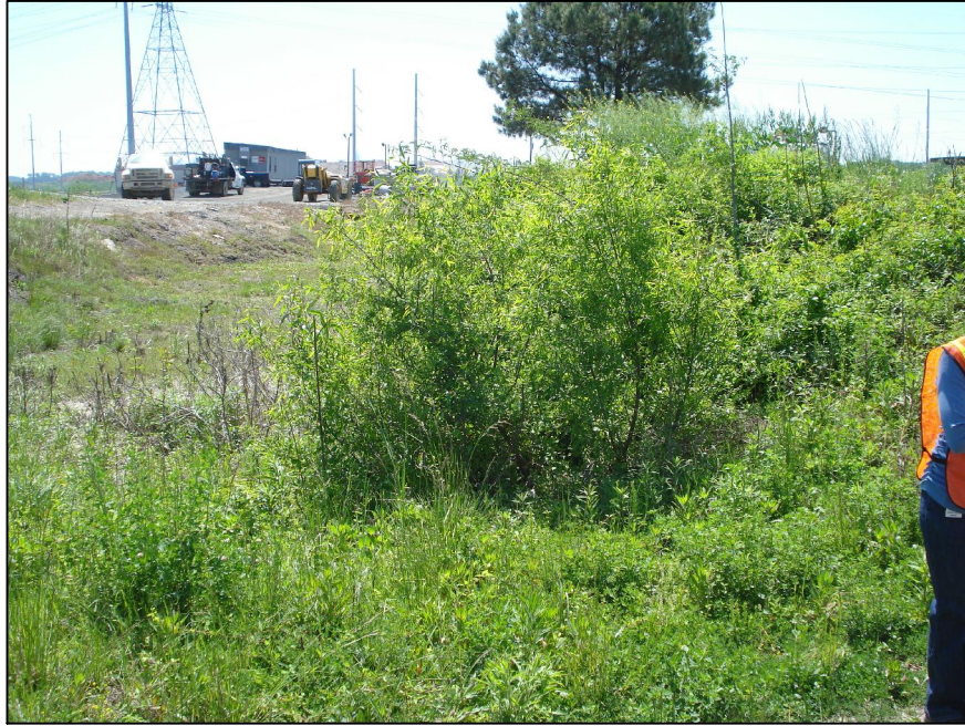
4-9 OVERGROWN EMERGENCY OVERFLOW
