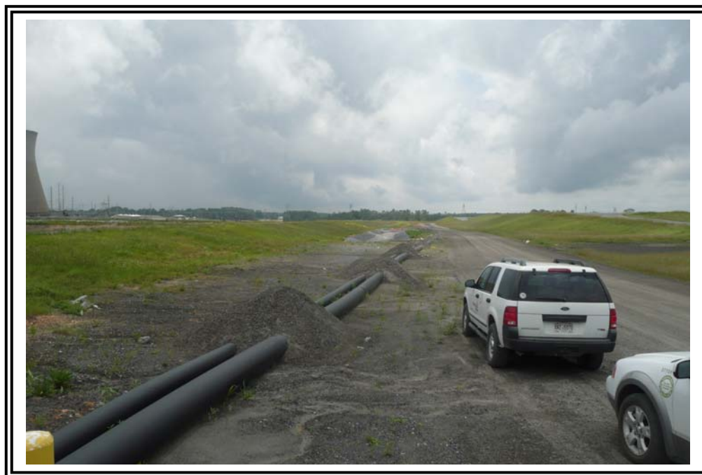
Within the main impoundment looking south. To the left of photo are the wet ash ponds (2) and to the right of the photo are the gypsum ponds (2).
