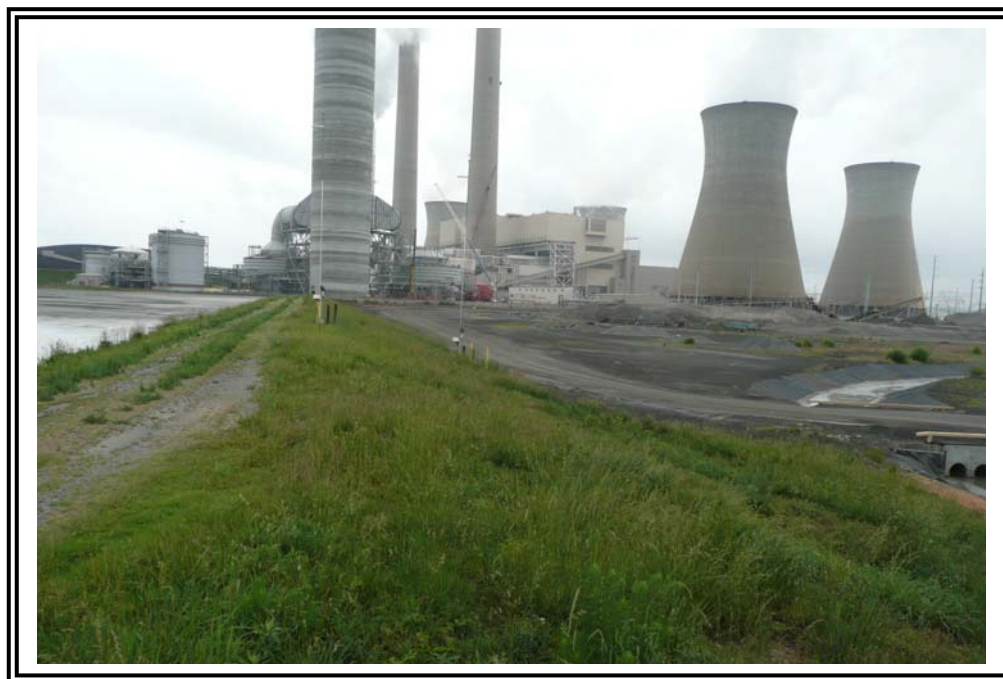
South embankment of wet ash ponds, looking East. Note the lined drainage swale in right of photo discharges into the reclaim pond.
