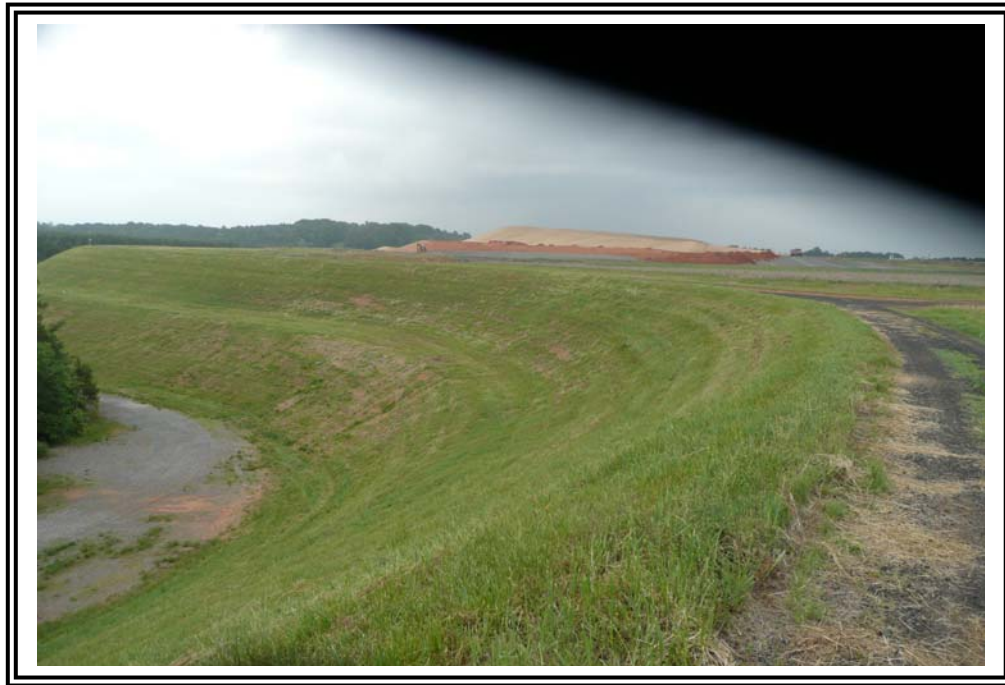
Embankment at the "Horseshoe" looking north. Gray coloring at toe of embankment is gravel placed during the grouting program to seal karst features below the embankment.
