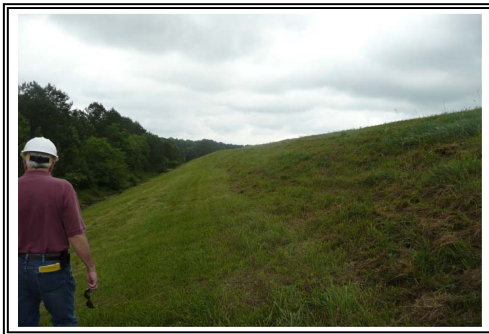
South end of the main dike, looking west. Note transition between natural cut slope and raised dike.
