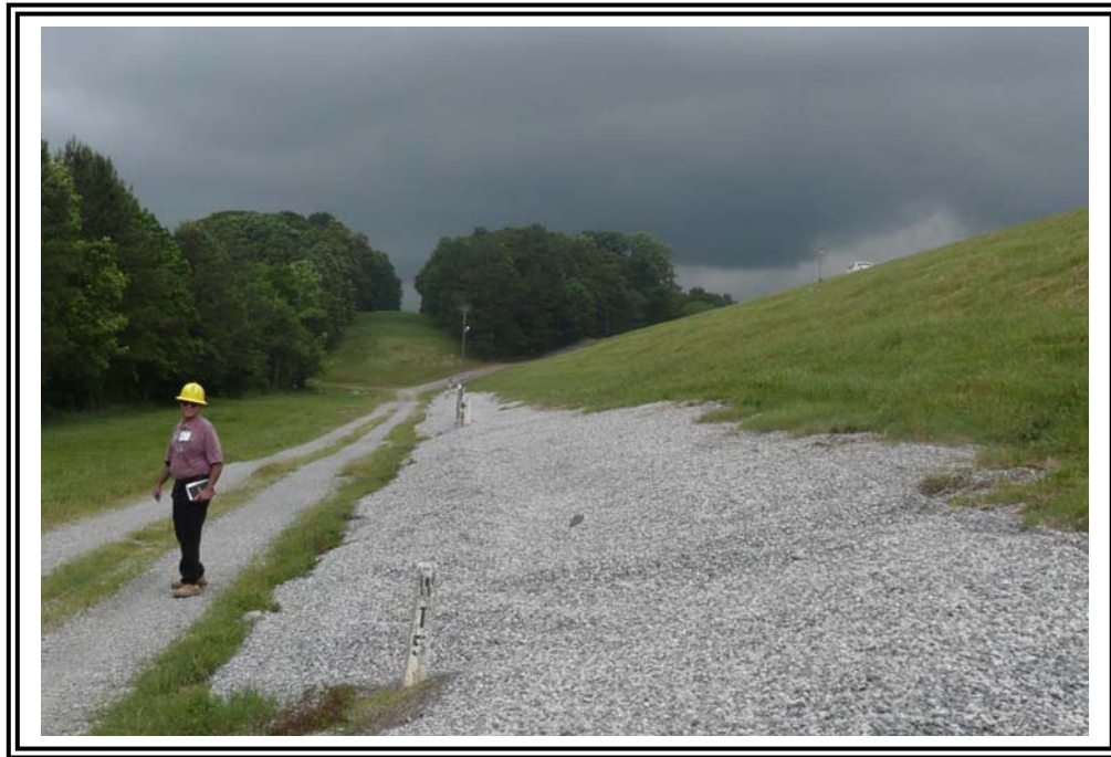
Stone cover at North end of main embankment placed during the grouting program to seal karst features below the embankment. The white numbered concrete posts mark toe drain locations.
