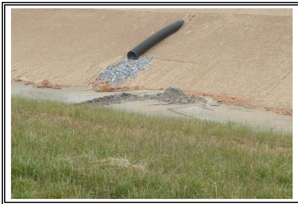
Surficial drainage system draining storm water runoff from ash stacks to the drainage swale.
