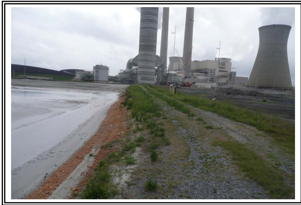
Upstream slope of south embankment of wet ash ponds, looking east. Note the red clay liner which overlays a liner.
