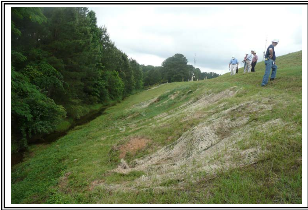
Continuing west on south end of main dike, another slough area in the natural slope reportedly unchanged in 6 to 10 years per Georgia Power engineer responsible for inspections. This area reportedly has had a difficult time re-establishing grass growth so more recent efforts included placing erosion matting.
