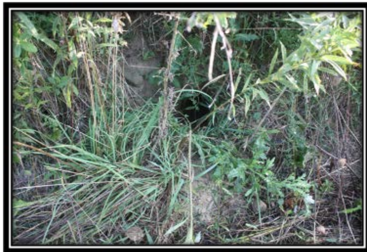
Figure 5.2.3-3 Animal hole in lower part of outside slope of perimeter dike embankment on southwest side of Ash Filter Ponds (next to Pond A).
