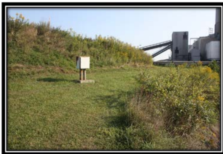
Figure 5.2.3-1 Outside slope and toe of highest embankment – southwest side of Ash Filter Ponds viewed southeast (next to Pond A).
