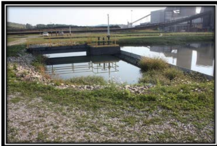
Figure 5.2.2-1 Typical inside slope – northwest side of Ash Filter Ponds viewed northeast (next to Pond A).
