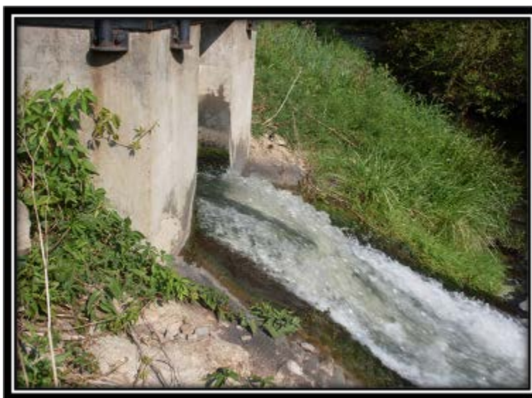
Figure 5.4.2-3 Thermal Pond discharge from Parshall flume at end of outlet pipe.
