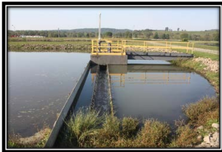
Figure 5.4.1-1 Typical outlet structure for Ash Filter Ponds – Pond B outlet viewed southwest.
