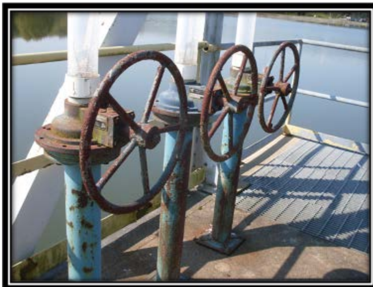
Figure 5.4.2-2 Surface corrosion on gate operators for the three drawdown valves on the south side of the Thermal Pond outlet structure.
