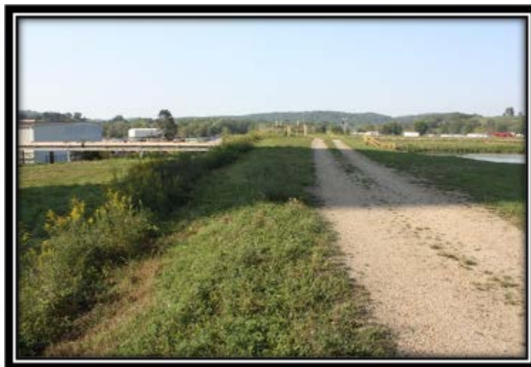
Figure 5.2.1-1 Crest and outside slope of Ash Filter Ponds – southwest side viewed northwest (highest embankment, next to Pond A).
