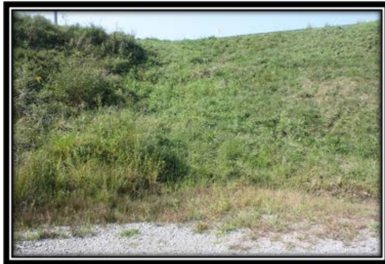
Figure 5.3.4-1 Groin area at south end of the east side main embankment dam above access road berm – viewed west.
