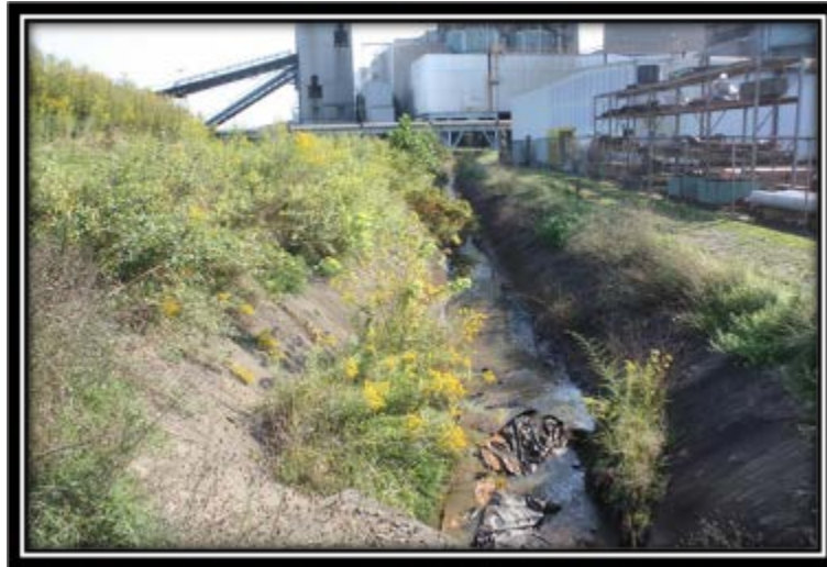
Figure 5.2.3-2 Outside slope and paved ditch below the toe of the perimeter dike embankment – southeast side viewed northeast (next to Pond A).
