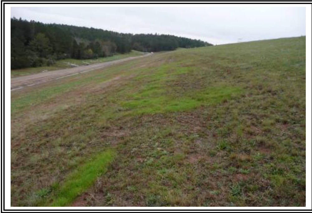
Ash Pond E, mid-height of dike, northern end of dam facing south. Mower-rutting observed throughout portions of the dike. Rye grass patching observed and indicated to be seasonal grass cover in effort to minimize sparse vegetation.
