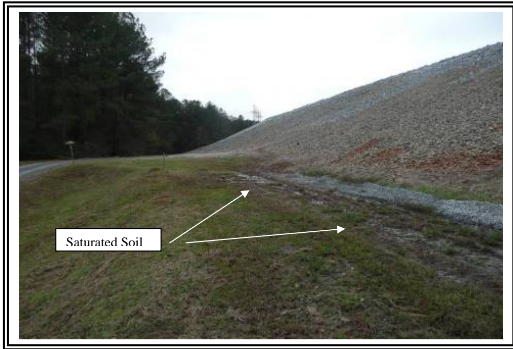
Ash Pond C, western central portion of south dike facing west. Saturated soil shown.
