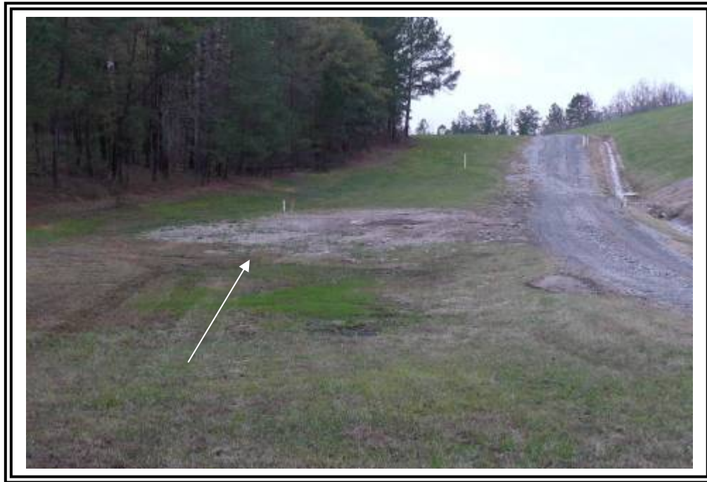
Ash Pond D, central portion of dike, west of toe facing north west. "Soft area" covered with rock indicated by arrow.
