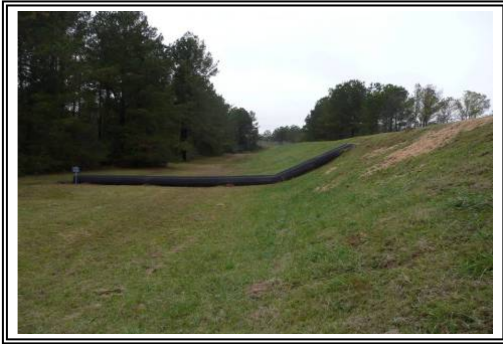
Ash Pond C emergency overflow located on southern portion of west dike north of historic discharge facility.
