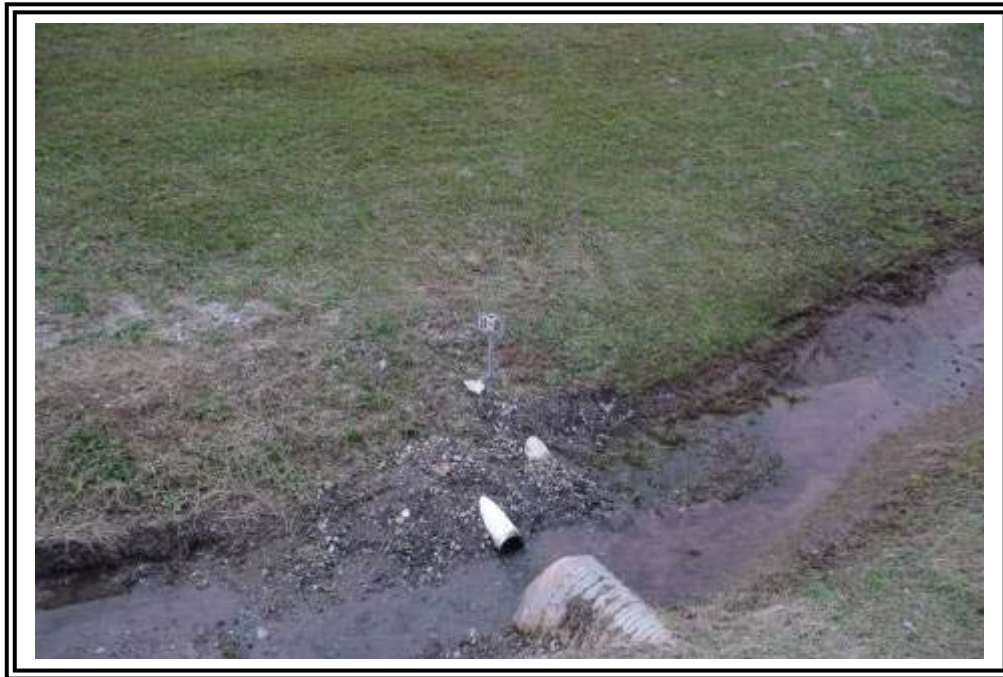
Ash Pond D finger drain D-3. .
