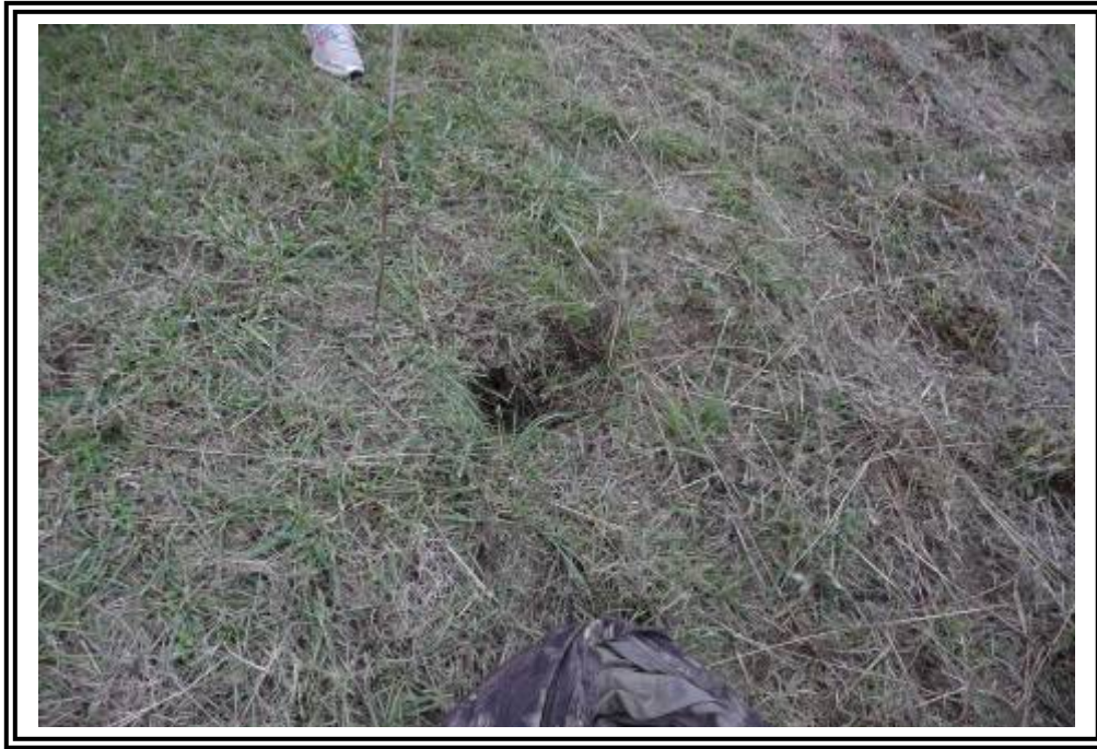
Ash Pond D, animal burrow located along central portion of the dike along the interior edge. One of several found throughout the length of the dike.
