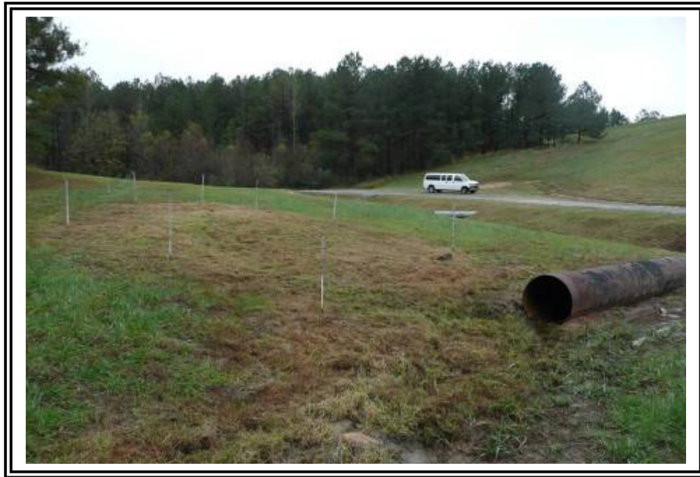
Ash Pond E, “soft spot” located south of emergency overflow drain (1 of 3 observed near Ash Pond E). This area has been monitored for nine years by Georgia Power with no additional expansion observed. Perimeter stakes have been placed to aid in monitoring.
