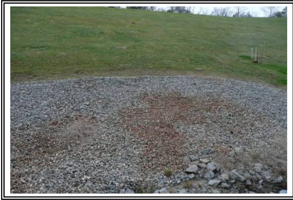
Ash Pond D, central portion of dike at edge of toe. Seepage remediation area shown. Georgia Power personnel indicated that this area was previously remediated and the concrete lined channel was inadvertently razed during remediation
