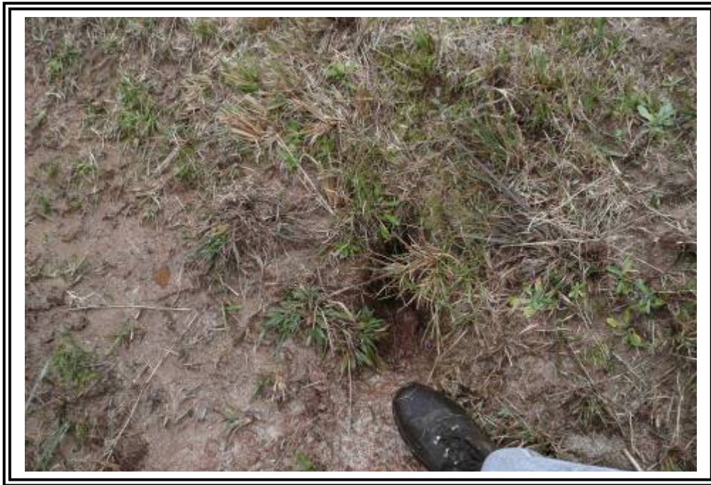
Ash Pond C, north portion of west dike, rodent burrow observed on upstream side of dike.
